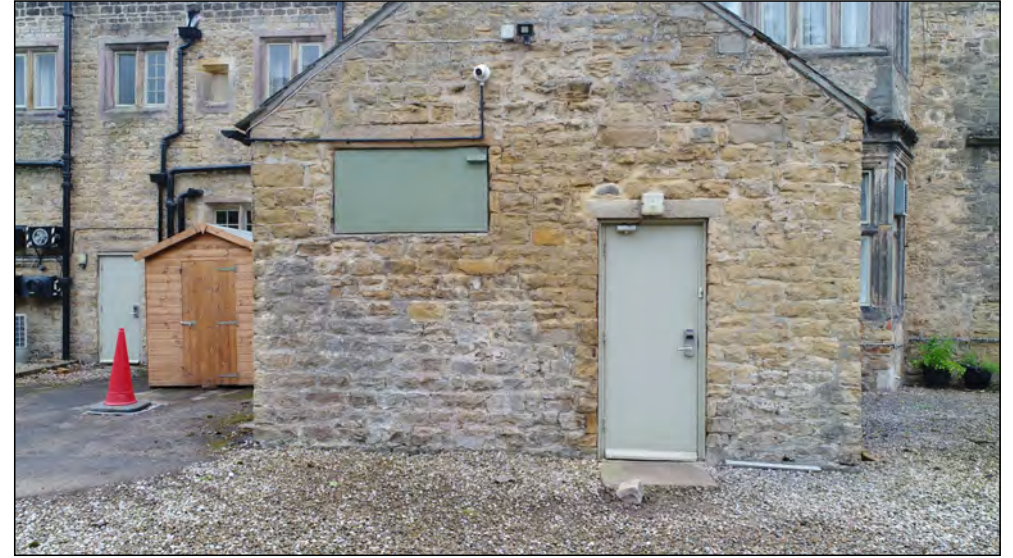
Photo 82. North facing exterior elevation, showing extension projecting northwards from west end of North Range, ground floor.
