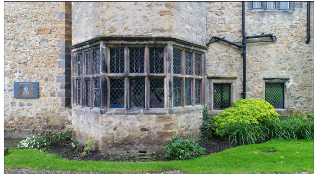
Photo 64. East facing exterior elevation of bay windows towards centre of East Range, ground floor.
