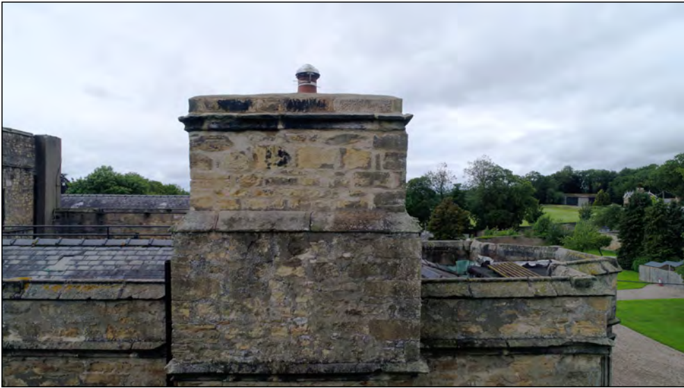
Photo 73. East facing exterior elevation, north end of East Range, upper part of first floor and roof, with detail of chimney stack.
