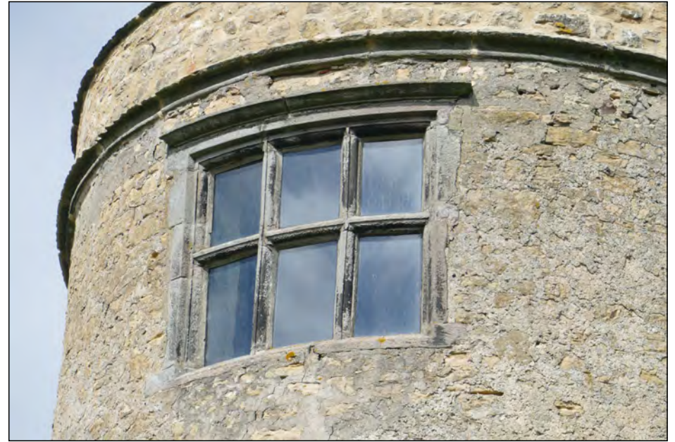
Photo 46. Detail of three-light transomed window, south facing, third floor of SE tower.
