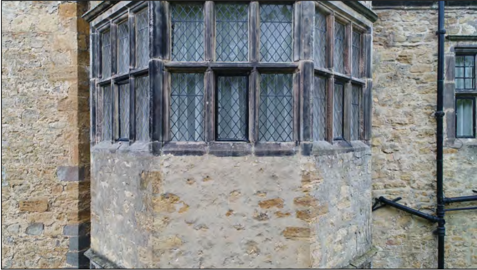
Photo 65. East facing exterior elevation of bay windows towards centre of East Range, first floor.
