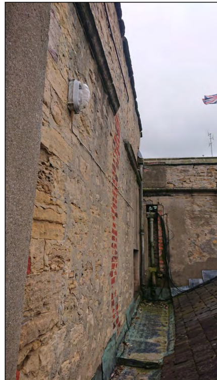
Photo 95. View looking south along roof corridor at west end of former manor house, second floor.
