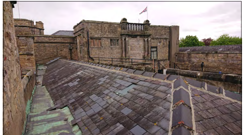
Photo 92. Oblique view towards Renaissance facade of former manor house, taken from NE corner of roof of North Range.
