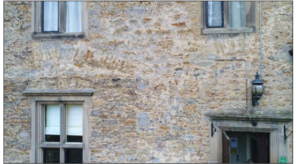
Photo 54. Detail of former arched openings in east facing exterior elevation, south end of former manor house, above later window and doorway.
