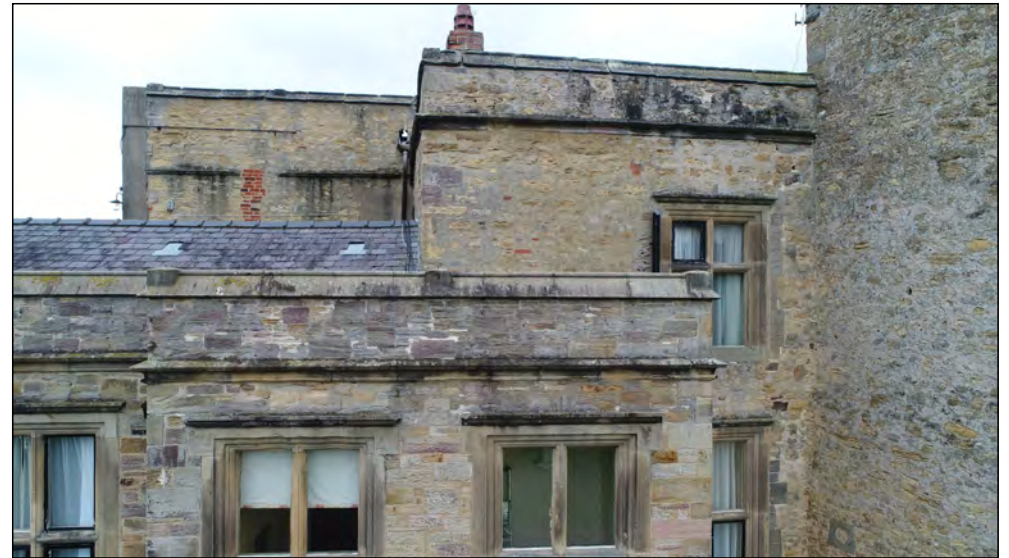
Photo 10. West facing exterior elevation, above reception entrance, upper first floor of west range and second floor of former manor house.
