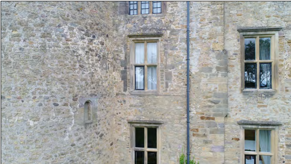
Photo 25. South facing elevation, west end of former manor house, first floor, with east facing round arched window in adjoining tower first floor.
