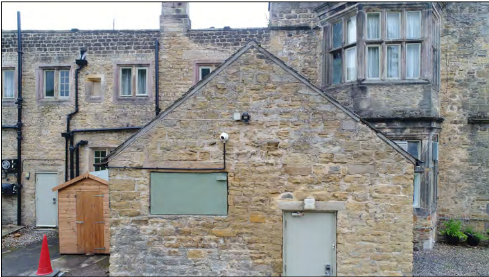
Photo 83. North facing exterior elevation, showing gable of extension projecting northwards from west end of North Range.
