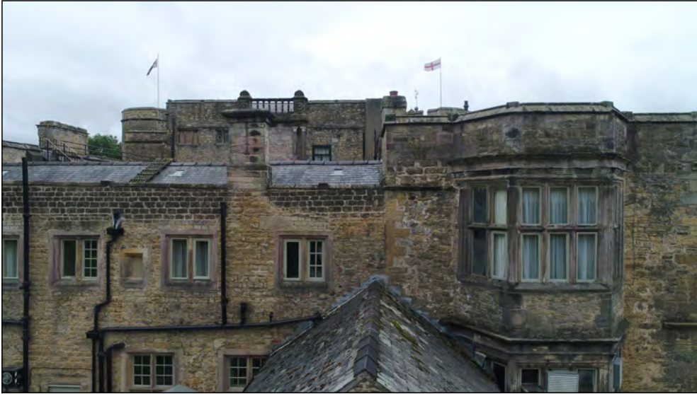
Photo 85. North facing exterior elevation, above extension at west end of North Range, upper part of first floor.
