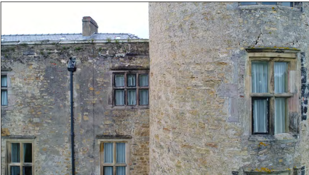
Photo 39. South facing exterior elevation of SE-tower and east end of former manor house, second floor.
