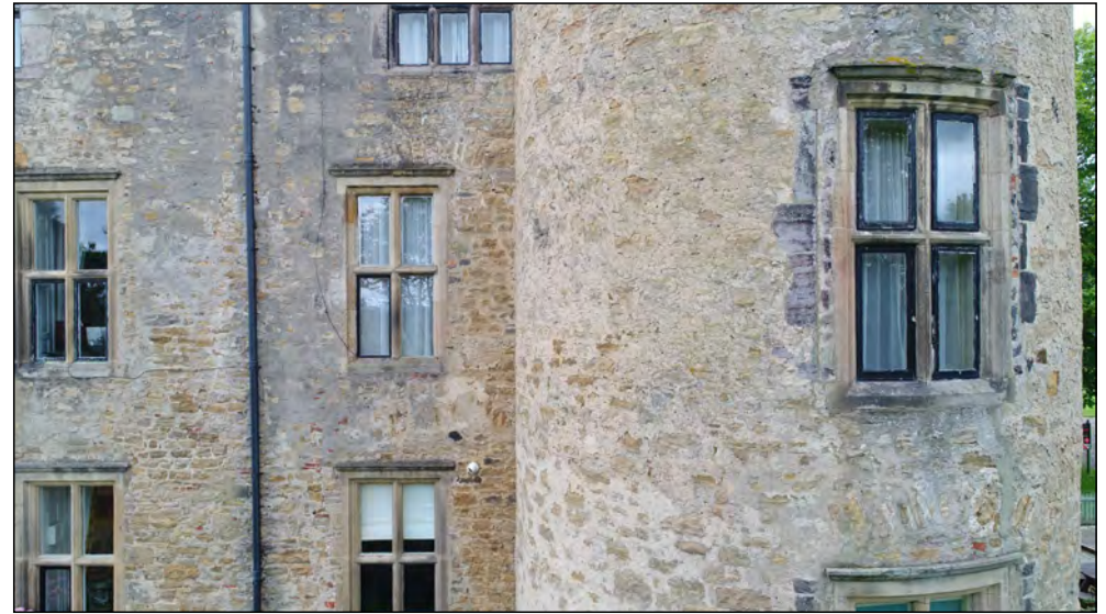
Photo 38. South facing exterior elevation of SE-tower and east end of former manor house, first floor.
