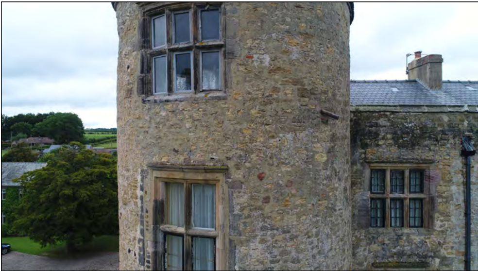
Photo 21. South facing exterior elevation of SW-tower and west end of former manor house, second/third floor.
