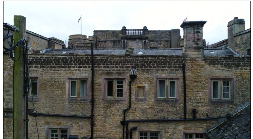
Photo 80. North facing exterior elevation, centre of North Range, upper part of first floor.
