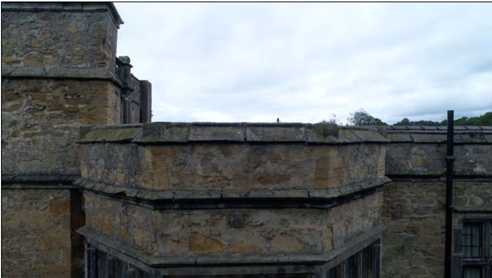
Photo 67. East facing exterior elevation of parapet above bay at centre of East Range.
