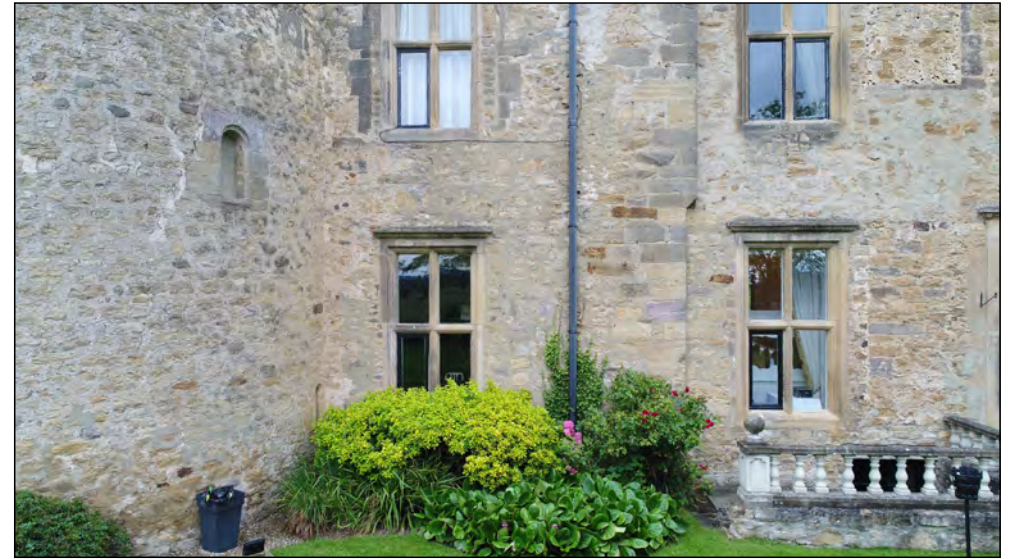
Photo 24. South facing elevation, west end of former manor house, ground floor, with east facing round arched window in adjoining tower first floor.
