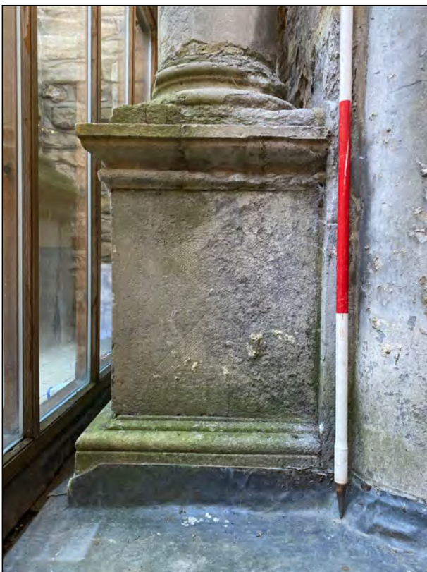
Photo 107. East view, showing detail of column pedestal on east side of doorway.
