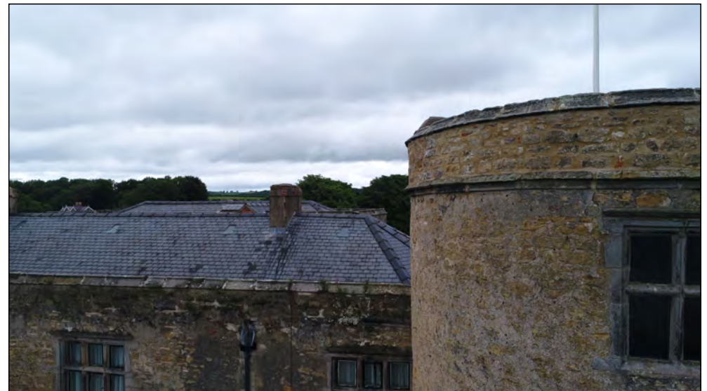
Photo 40. South facing exterior elevation of SE-tower and east end of former manor house, upper second floor and roof.
