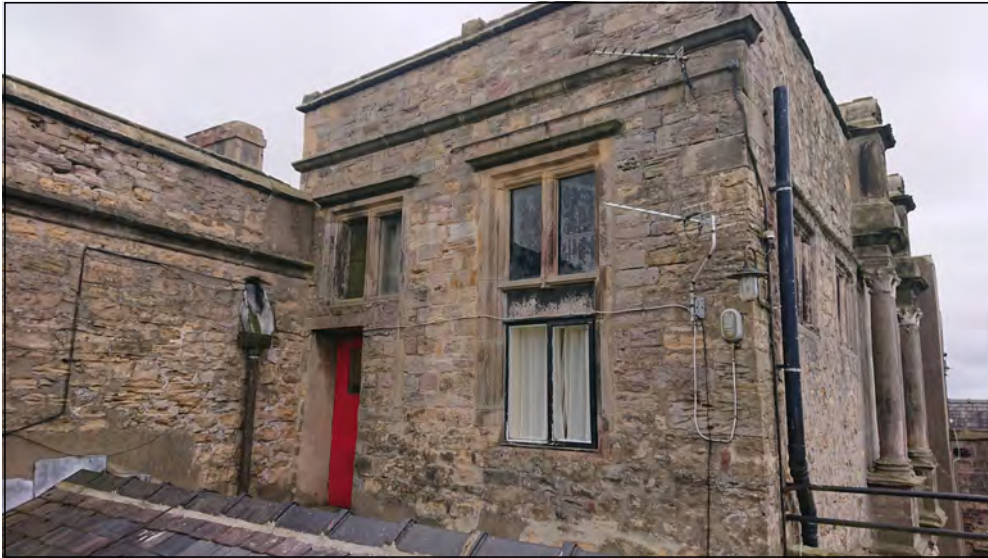
Photo 93. Oblique view of east facing exterior elevation of Renaissance facade second floor, from roof of East Range.
