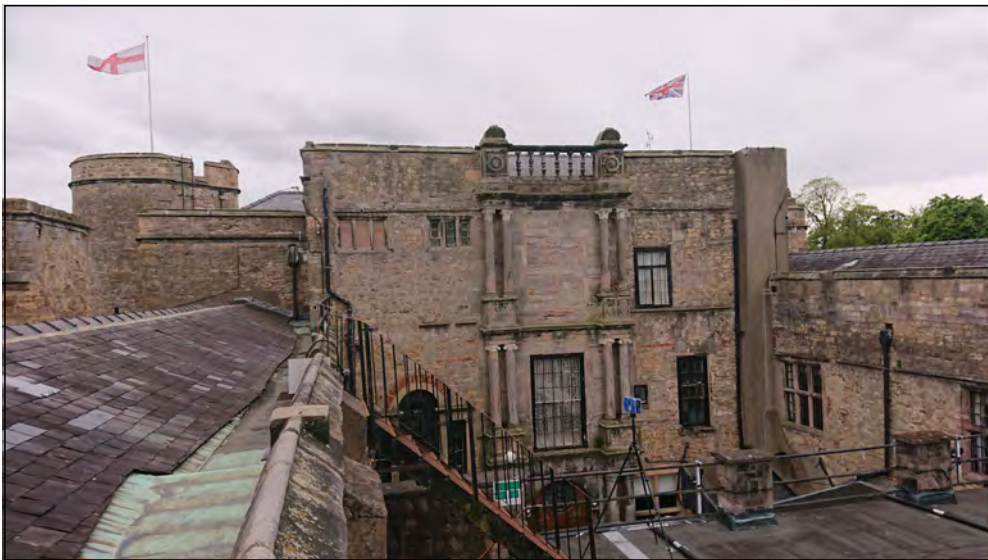
Photo 91. Oblique view towards Renaissance facade of former manor house, taken from roof of North Range.
