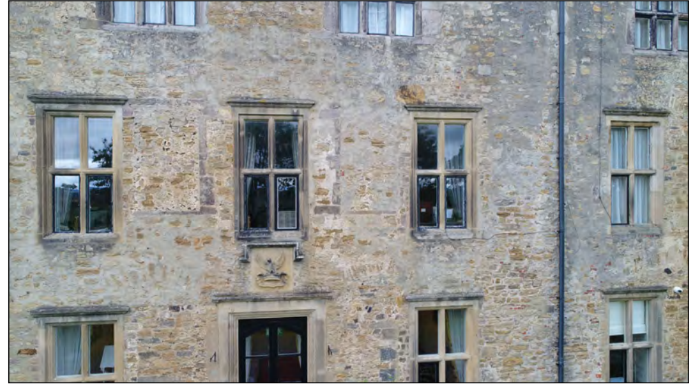
Photo 32. South facing exterior elevation, centre of former manor house, first floor, above entrance.
