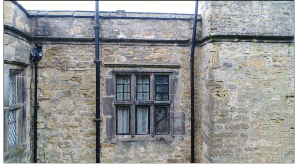
Photo 70. East facing exterior elevation, centre-north of East Range, upper part of first floor.
