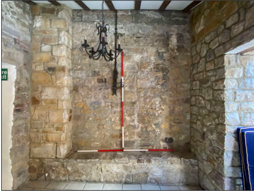
Photo 101. North facing elevation of Renaissance facade of former manor house, within courtyard extension, east side.
