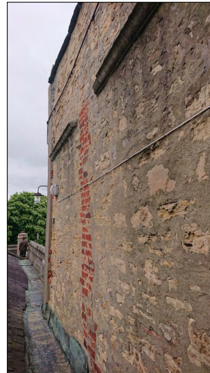
Photo 96. View looking north along roof corridor at west end of former manor house, second floor.
