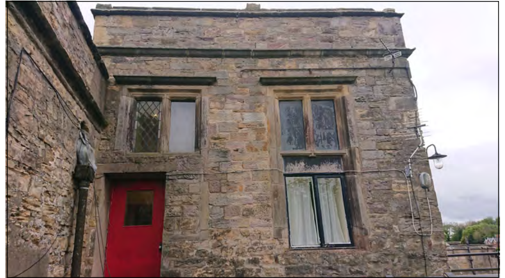
Photo 94. East facing exterior elevation of Renaissance facade second floor, from roof of East Range.
