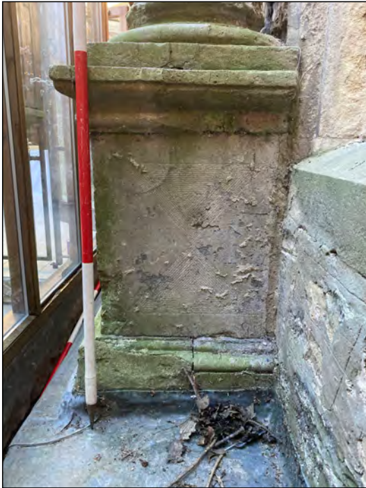
Photo 112. West view, showing detail of column pedestal on west side of doorway. 69
