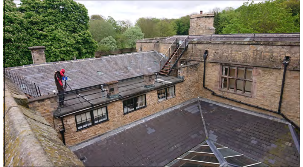
Photo 98. View looking north-east across Walworth Castle roof, from East Range towards North Range.
