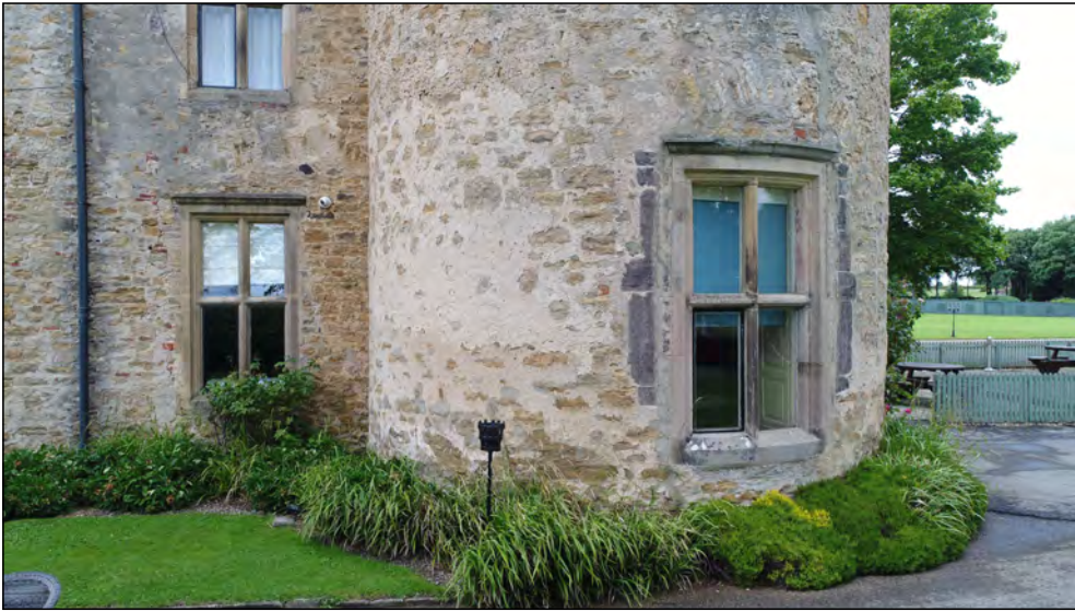
Photo 37. South facing exterior elevation of SE-tower and east end of former manor house, ground floor.
