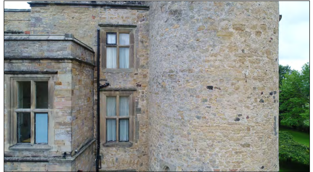
Photo 12. West facing exterior elevation, south of reception entrance, with former manor house and SW-tower first and second floor.
