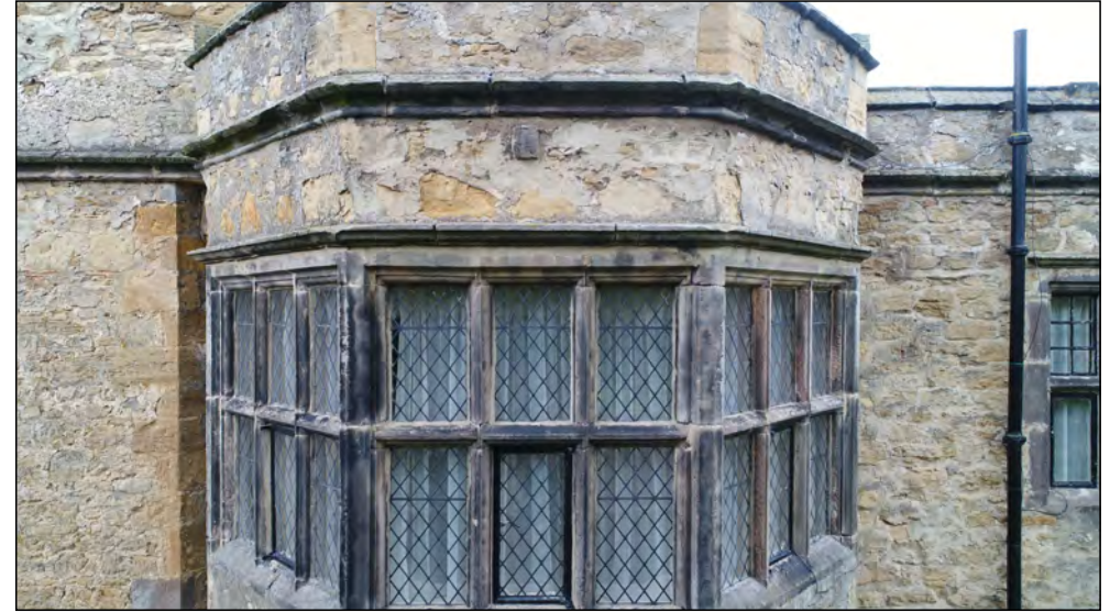
Photo 66. East facing exterior elevation of bay windows towards centre of East Range, upper part of first floor.
