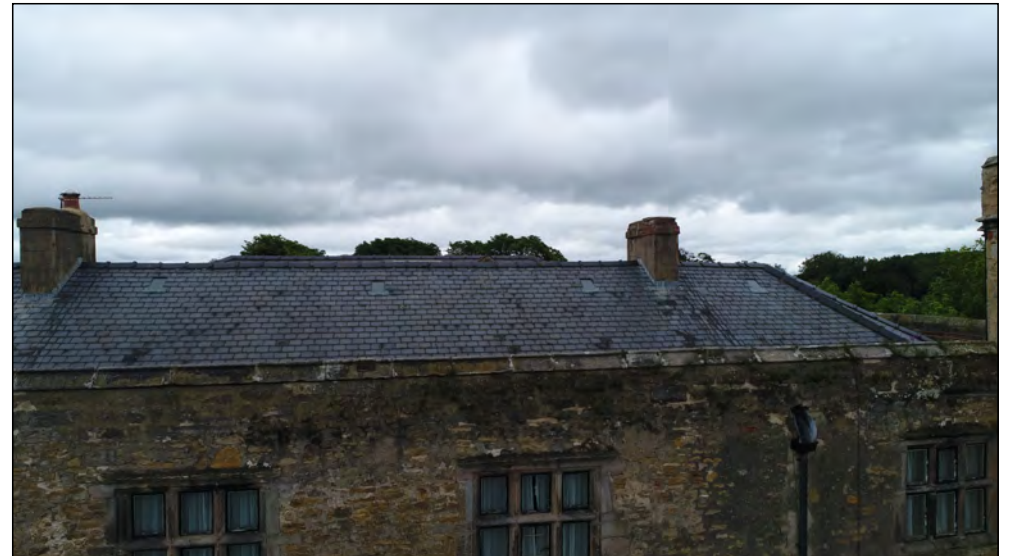
Photo 34. South facing exterior elevation, centre of former manor house, upper second floor and roof, above entrance.
