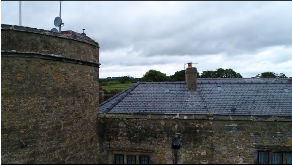
Photo 27. South facing elevation, west end of former manor house, upper part of second floor and roof.
