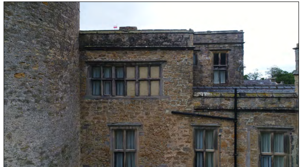
Photo 56. East facing exterior elevation, south end of former manor house, second-third floors.
