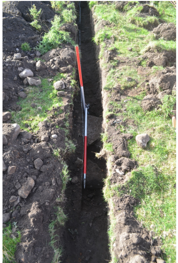
Photo 07. Oblique view of pipe trench looking north, showing [102] in the middle ground.
