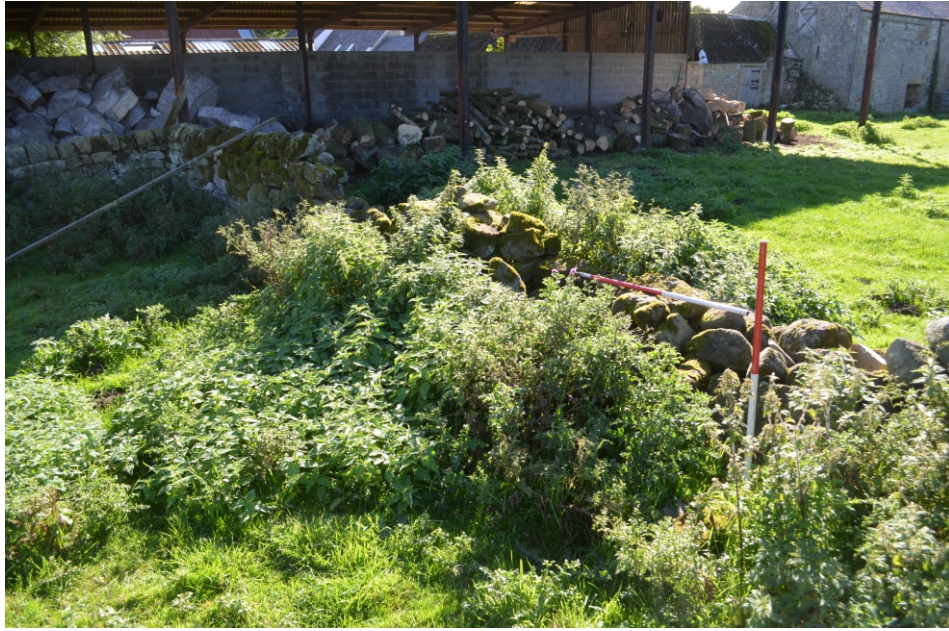
Photo 14. The collapsed drystone wall before deconstruction.
