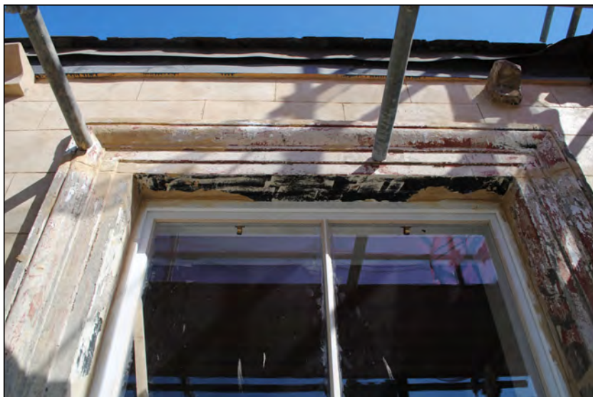
Photo 35. Exterior first floor, view looking NNW at upper architrave repairs to easternmost window of No. 2 High Street West, south wall.
