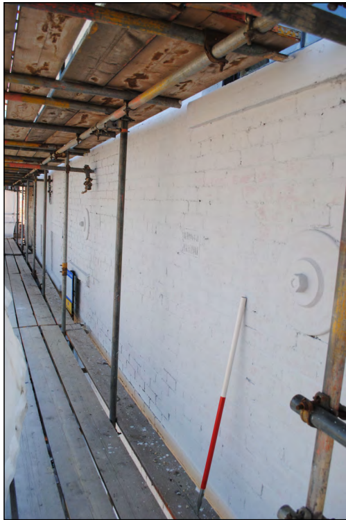
Photo 65. View looking NNW at concentric iron brackets bolted to the west wall of No. 1 High Street West.
