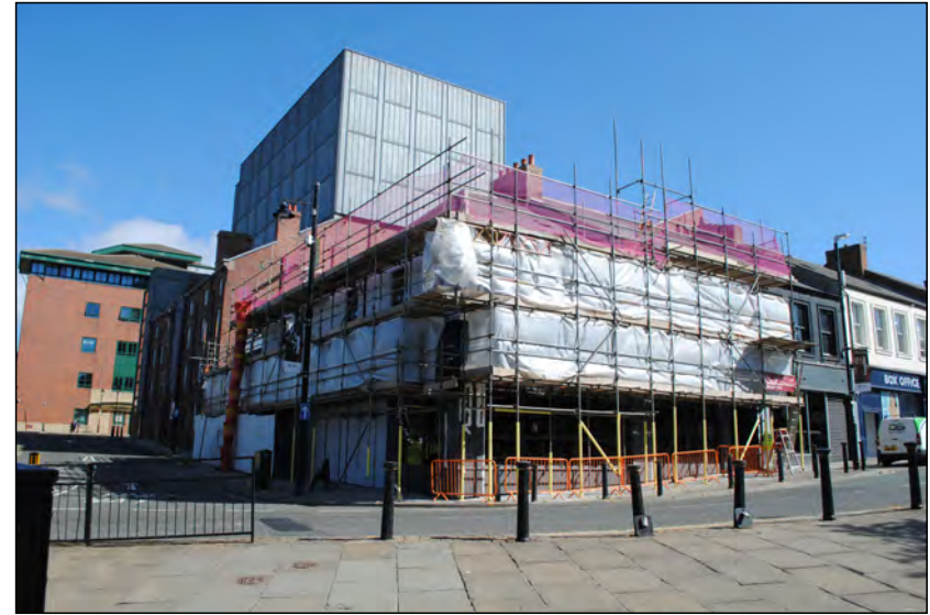
Photo 42. Broad view looking NE at 'The Rabbit', towards the end of renovation work.
