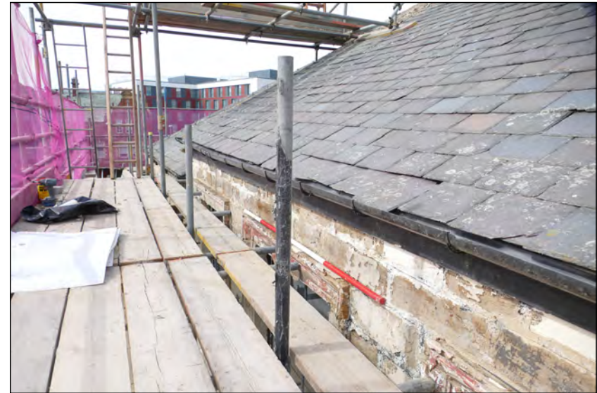
Photo 16. Interface of first floor exterior and roof, view looking WSW along the south wall of High Street West No. 2.
