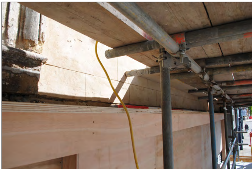
Photo 37. Interface between first and ground floors, exterior, south wall, view looking NE at repointed stonework.
