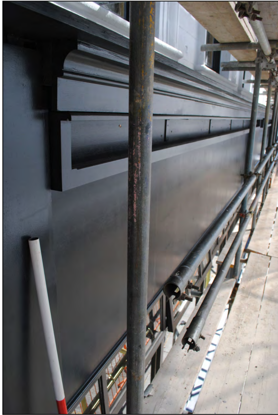
Photo 49. Exterior view looking NE along upper portion of 'shop-front' facade forming south elevation of High Street West Nos. 1-2.
