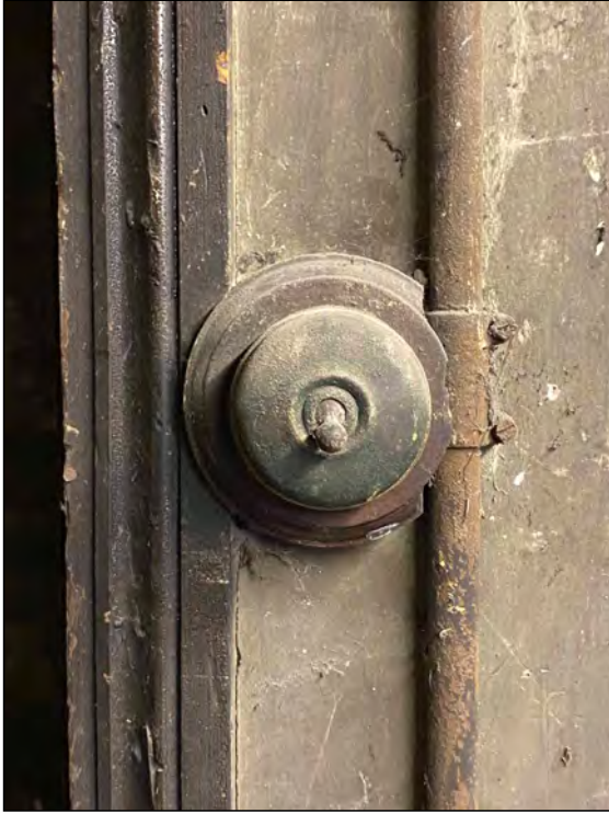
Photo 107. Detail of early-mid 20th century crabtree bakelite toggle light-switch, located in the north wall of the SW room in the attic space.
