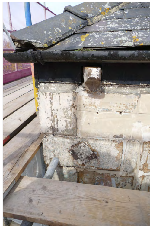
Photo 20. Interface of first floor exterior and roof, view looking NNW at SW corner of south wall.
