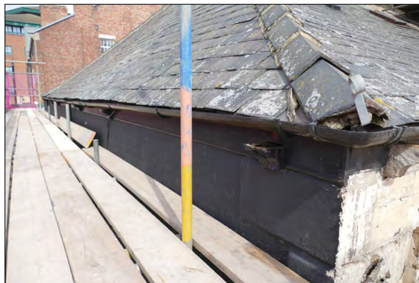
Photo 22. Interface of first floor exterior and roof, view looking NNW along the west wall of High Street West No. 1.
