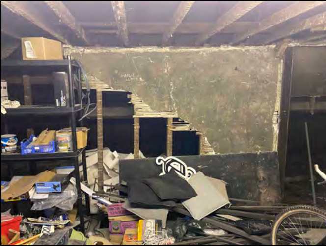
Photo 103. View looking NNW along the central part of the SW room of the attic space.
