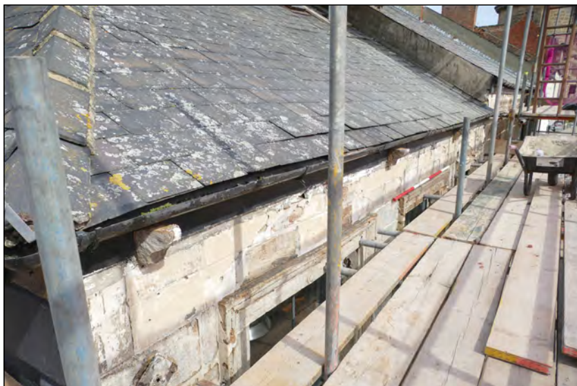
Photo 19. Interface of first floor exterior and roof, view looking ENE along the south wall of High Street West No. 1.
