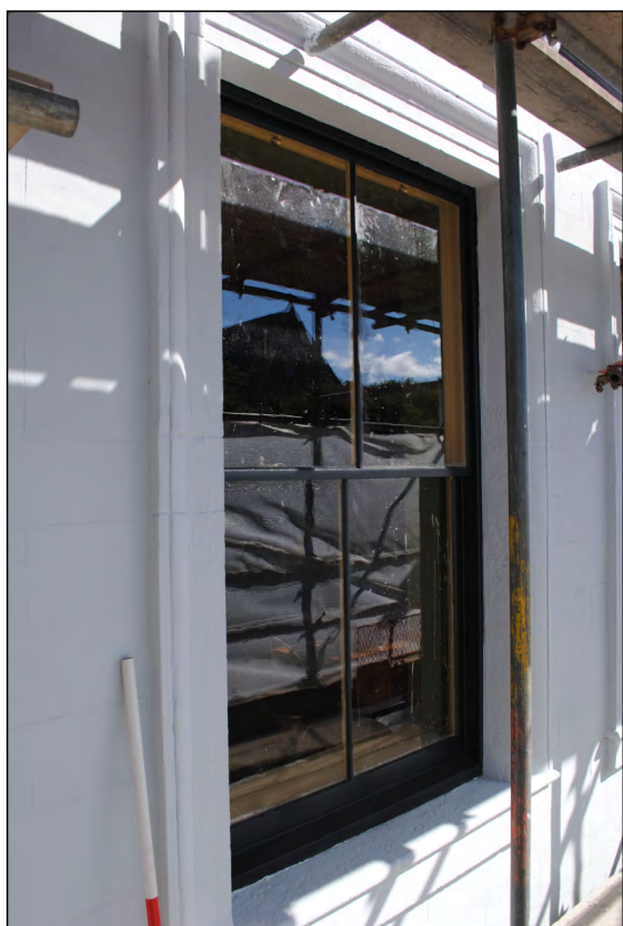
Photo 55. Exterior first floor, view looking North at finished easternmost window in the south wall of High Street West No. 2.
