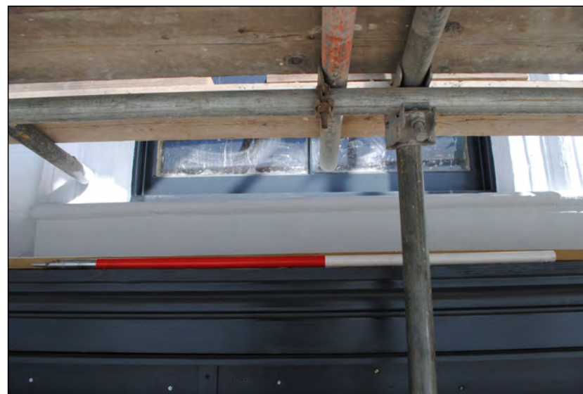
Photo 48. View looking NNW at finished sill of westernmost window in No. 2 High Street West, south wall, first floor.
