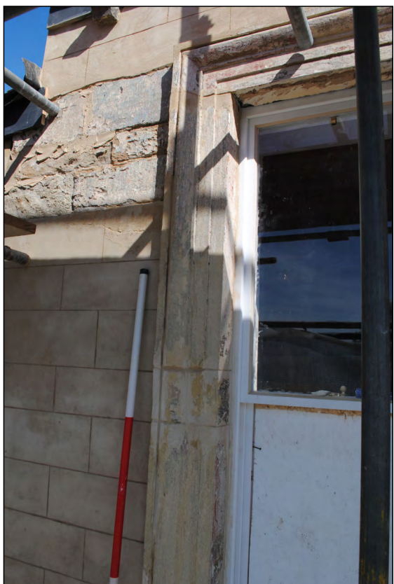
Photo 31. Exterior first floor, view looking NNW at detail of architrave repairs to westernmost window of No. 2 High Street West, south wall.
