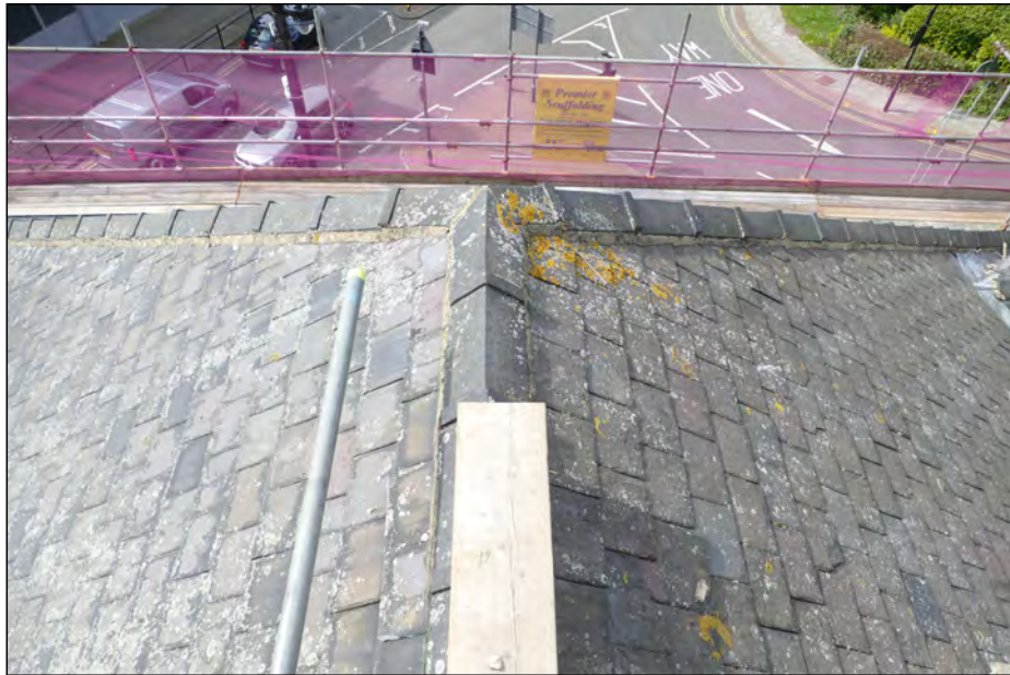
Photo 23. External roof, view looking WSW along apex ridge of High Street West No. 1.
