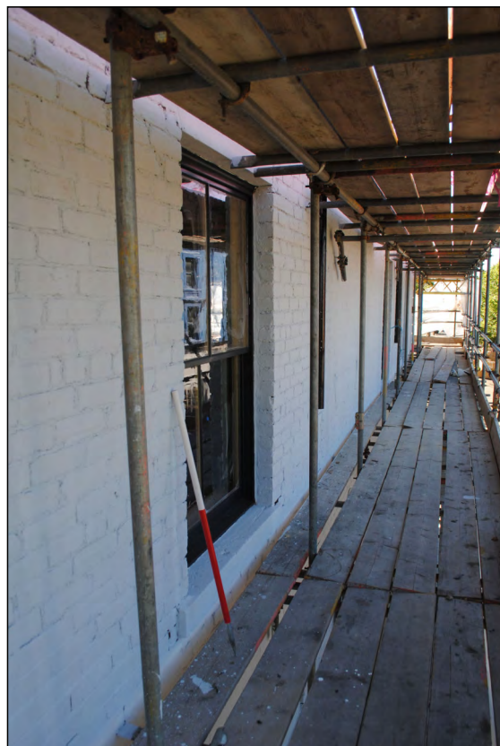
Photo 70. Exterior first floor, view looking SSE along west wall of No. 1 High Street West.
