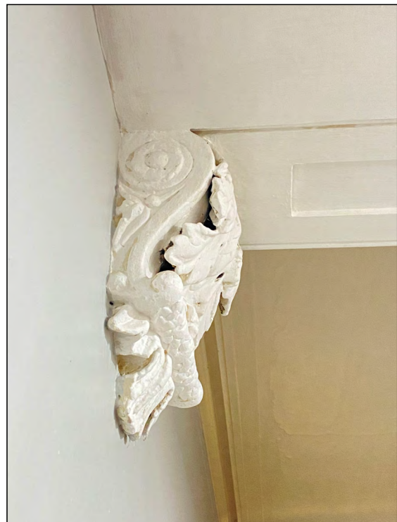
Photo 92. Detail of scrolled bracket with leaf design, as in 90. View looking NNW.
