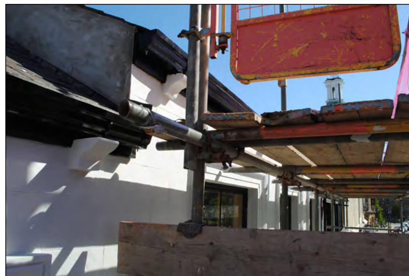
Photo 76. Interface of first floor exterior and roof, view looking ENE along the finished south wall of High Street West No. 2.
