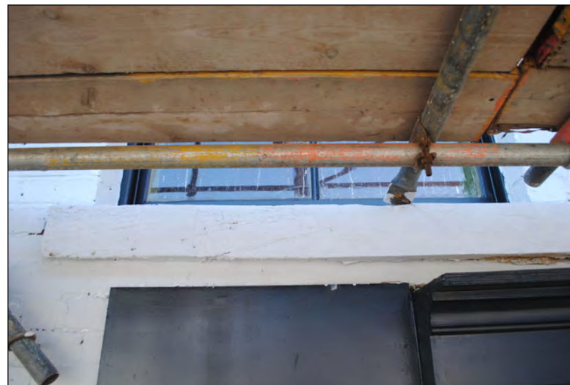
Photo 64. As 63, but a little to the north, showing detail of the finished southernmost sill above the 'shop-front' in the west wall.
