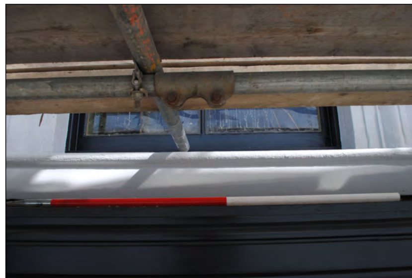
Photo 46. View looking NNW at finished sill of easternmost window in No. 2 High Street West, south wall, first floor.
