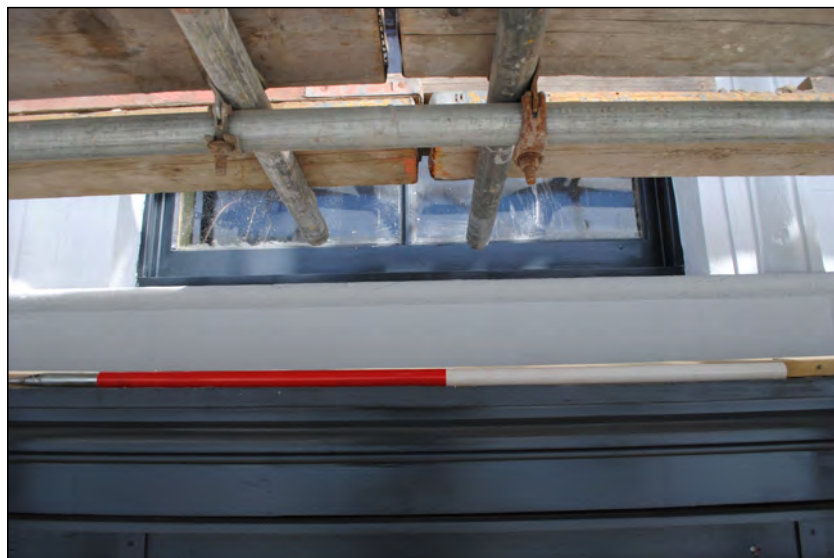
Photo 47. View looking NNW at finished sill of central window in No. 2 High Street West, south wall, first floor.
