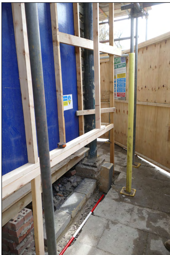
Photo 05. Ground floor exterior, view looking SE at detail of south-westernmost cast-iron column, supporting the 'shop-frontage'.
