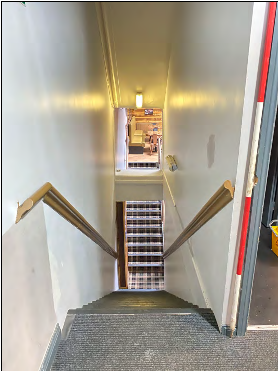
Photo 89. Interior view looking NNW down the stairs from outside the toilets located in the SE corner of the first floor, No. 3 High Street West.
