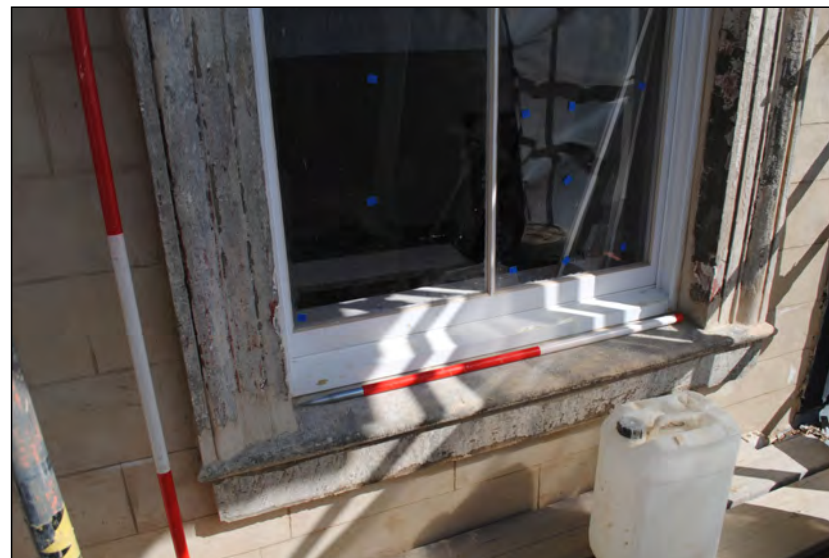
Photo 34. Exterior first floor, view looking NNW at sill and architrave repairs to easternmost window of No. 2 High Street West, south wall.
