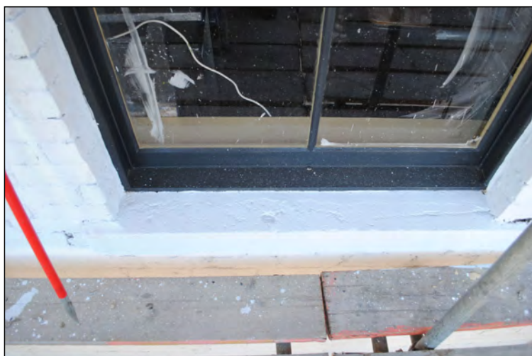
Photo 71. Exterior first floor, view looking SSE at finished sill in northernmost window of west wall, No. 1 High Street West.
