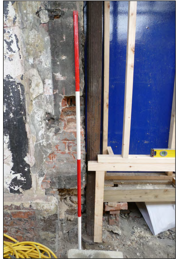
Photo 04. Ground floor exterior, view looking ENE at detail of north-westernmost cast-iron column, supporting the 'shop-frontage'.
