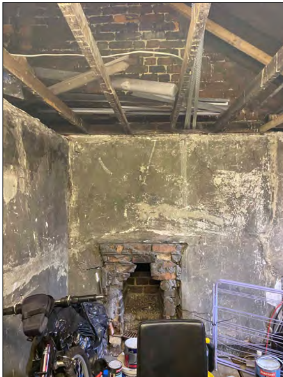
Photo 105. View looking ENE at east wall of the SW room in the attic space.
