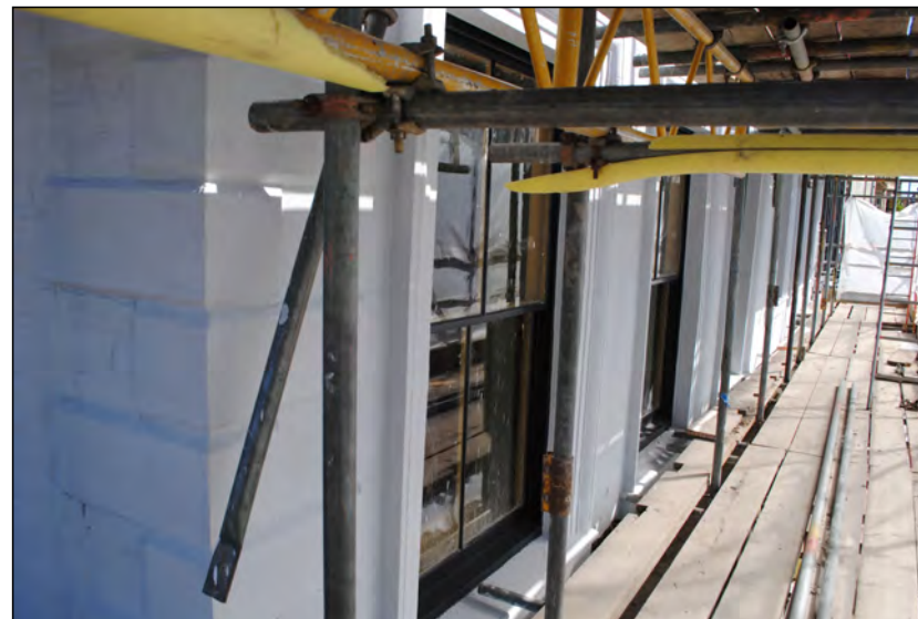
Photo 74. Exterior first floor, view looking ENE along south wall of No. 1 High Street West from the SW corner.
