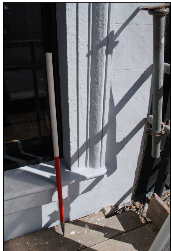
Photo 52. Exterior first floor, view looking NNW at detail of finished architrave in easternmost window in the south wall of High Street West No. 2.
