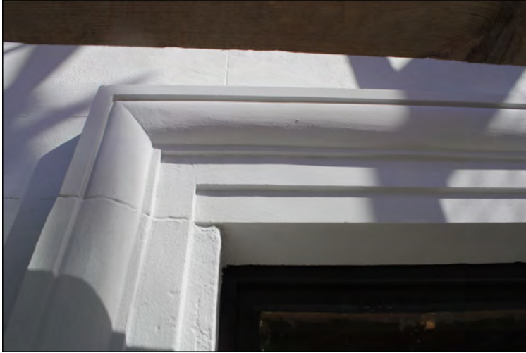
Photo 57. Exterior first floor, view looking NNW at finished upper architrave detail in easternmost window in the south wall of High Street West No. 1.
