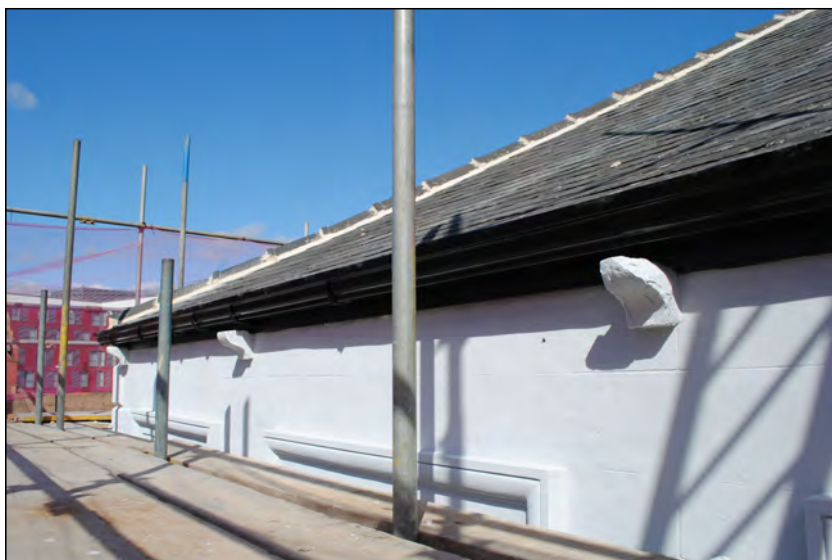
Photo 75. Interface of first floor exterior and roof, view looking WNW along the finished south wall of High Street West No. 1.
