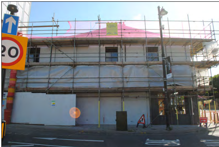
Photo 43. Broad view looking ENE at 'The Rabbit', towards the end of renovation work.
