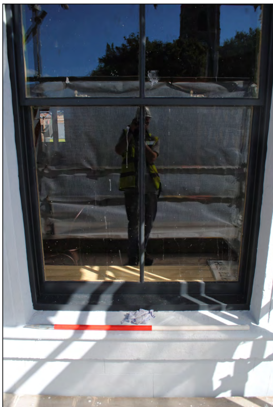
Photo 51. Exterior first floor, view looking NNW at finished easternmost window in the south wall of High Street West No. 2.
