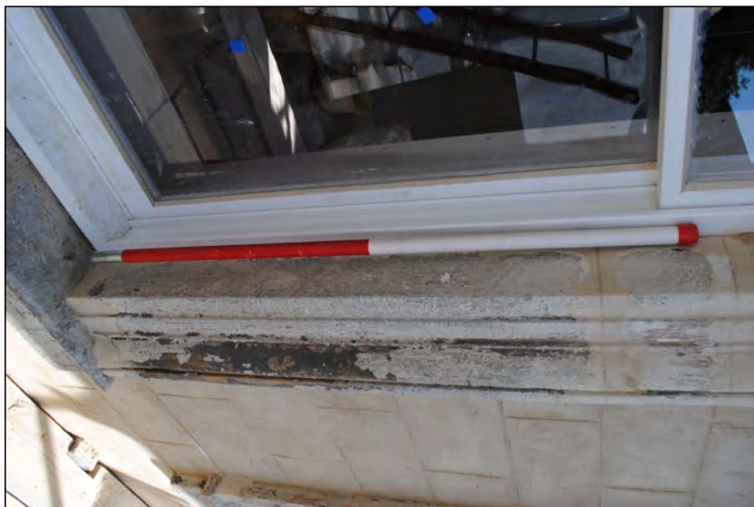
Photo 33. Exterior first floor, view looking NNW at sill repairs to central window of No. 2 High Street West, south wall.
