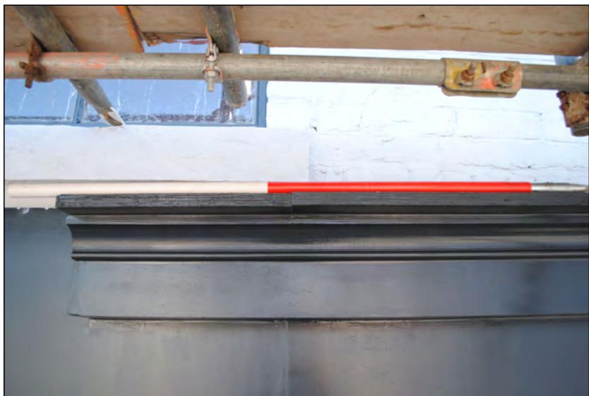
Photo 63. Exterior view looking ENE at upper portion of 'shop-front' in the west elevation of High Street West No. 1.
