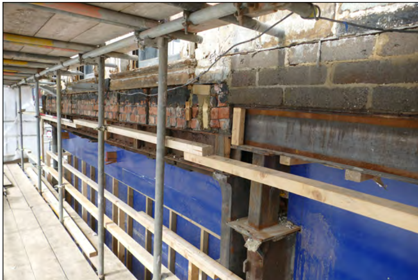
Photo 09. Interface between ground and first floors, view looking NW across the south wall, with detail of iron girder and column where High Street West No. 1 extends from No. 2.
