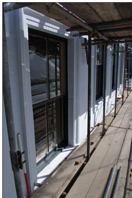
Photo 56. Exterior first floor, view looking NE along finished windows in the south wall of High Street West Nos. 1-2.
