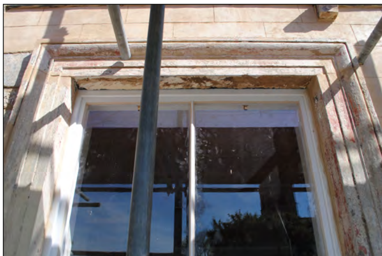
Photo 30. Exterior first floor, view looking NNW at upper architrave repairs to westernmost window of No. 2 High Street West, south wall.
