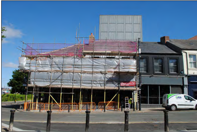
Photo 41. Broad view looking NNW at 'The Rabbit', towards the end of renovation work.
