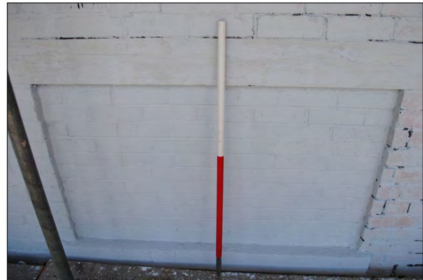
Photo 68. Exterior of west wall, view looking ENE at blocked opening with lintel and sill, towards the north end of No. 1.
