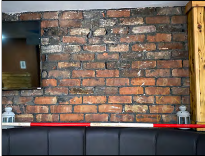
Photo 81. Interior ground floor, view looking WSW at detail of brickwork in the west wall at the NW portion of The Rabbit.
