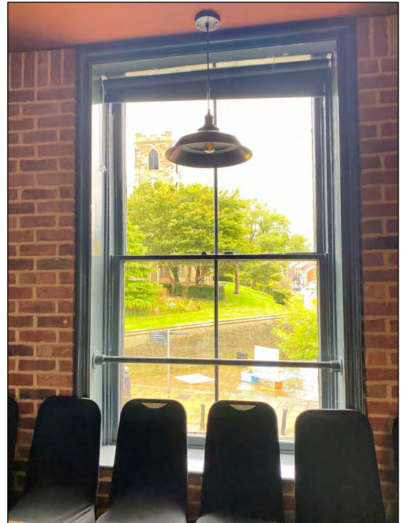
Photo 86. Interior first floor, view looking SSE at the westernmost window in the south wall No. 2 High Street West.
