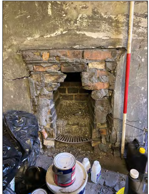
Photo 104. View looking ENE at detail of small fireplace in the east wall of the SW room in the attic space.
