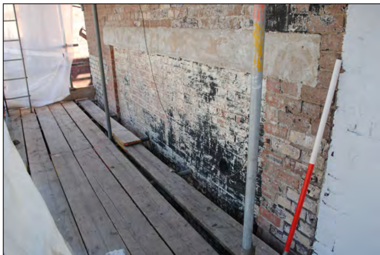
Photo 69. Exterior of west wall, view looking north at a second blocked opening with lintel and sill at the north end of No. 1.
