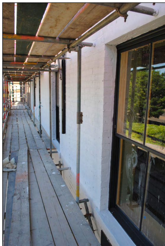
Photo 72. Exterior first floor, view looking NNW along west wall of No. 1 High Street West.
