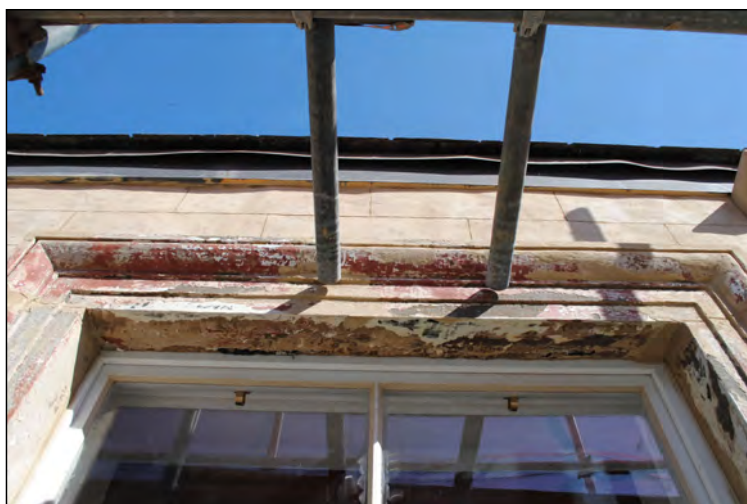
Photo 32. Exterior first floor, view looking NNW at upper architrave repairs to central window of No. 2 High Street West, south wall.
