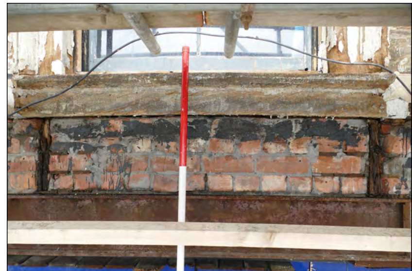
Photo 10. Interface between ground and first floors, view looking NNW at lower part of crumbling window architrave and lintel in the south wall, easternmost window of High Street West No. 1.
