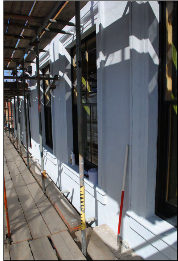
Photo 50. Exterior first floor, view looking west along finished windows in the south wall of High Street West Nos. 1-2.
