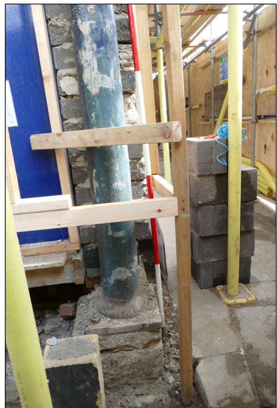
Photo 06. Ground floor exterior, view looking ENE at detail of south-westernmost cast-iron column, supporting the 'shop-frontage'.
