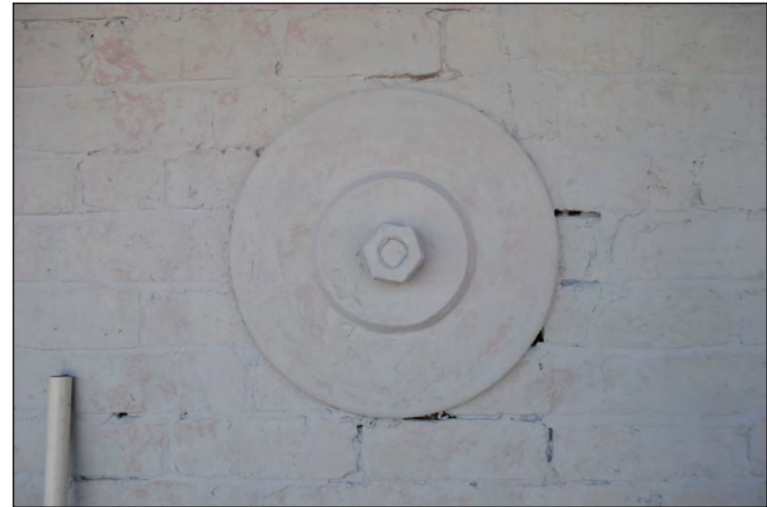
Photo 66. Detail of large concentric iron bracket, bolted on to the west wall of No. 1 High Street West, beneath the most central window.
