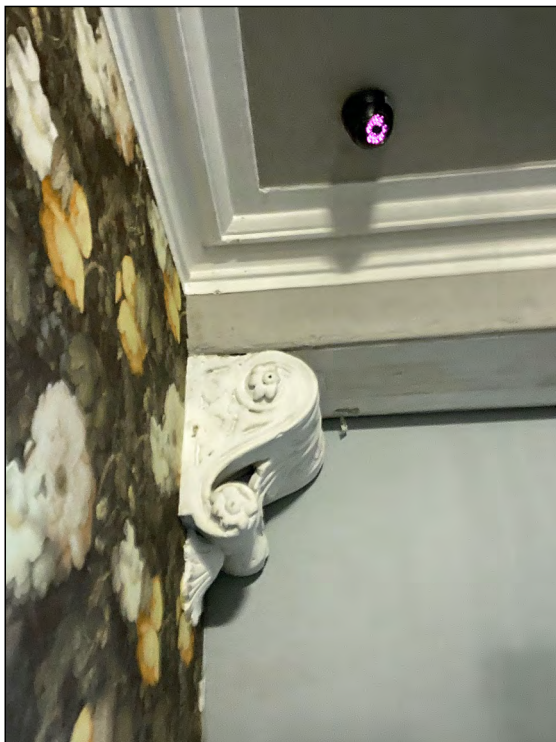
Photo 83. View looking NW at scrolled bracket with leaf decoration, located at the doorway in the corridor at the NW area of The Rabbit interior.
