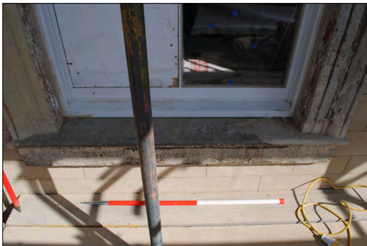
Photo 29. Exterior first floor, view looking NNW at sill and architrave repairs to westernmost window of No. 2 High Street West, south wall.
