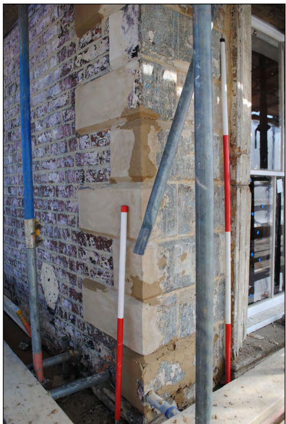
Photo 25. Exterior first floor, view looking NE at repair work to quoins in SW corner.
