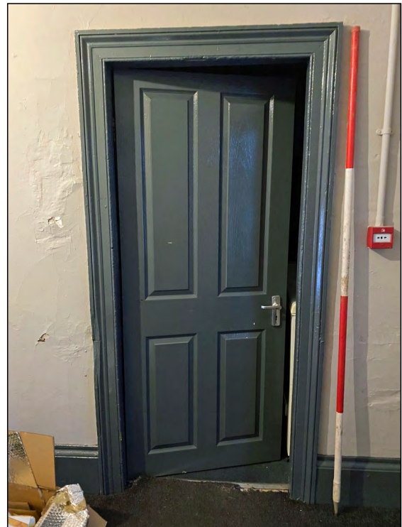
Photo 96. Door on loft landing at top of back stairs (left door in Pic. 95).
