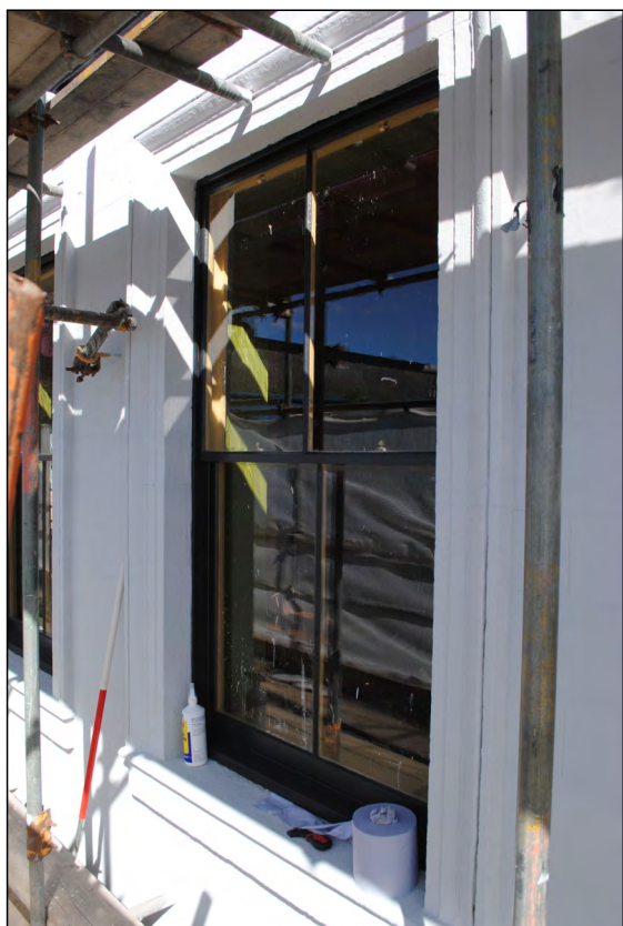
Photo 53. Exterior first floor, view looking NW at finished central window in the south wall of High Street West No. 2.
