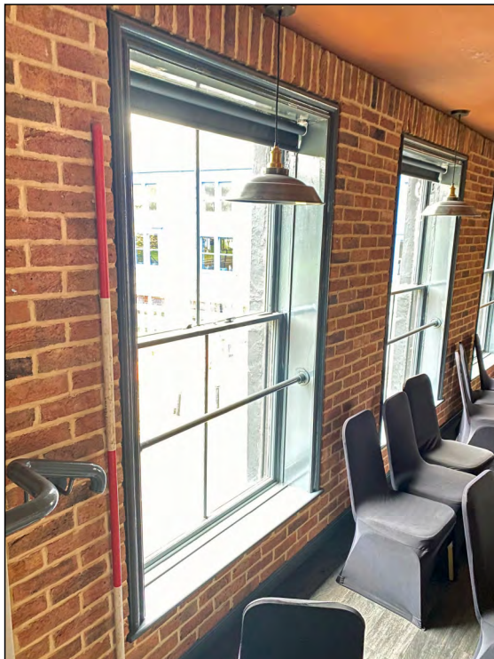
Photo 87. Interior first floor, view looking WSW at windows in the south wall of No. 1 High Street West.
