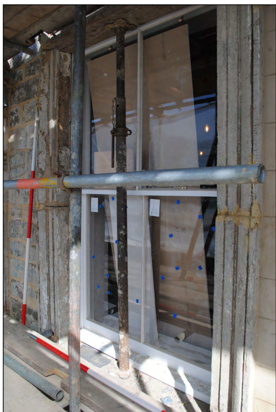
Photo 27. Exterior first floor, view looking NW at repairs to westernmost window in south wall.
