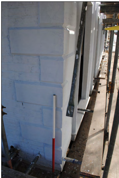
Photo 61. Exterior first floor, view looking NE at finished quoin work in the SW corner of High Street West No. 1.
