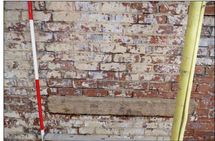
Photo 08. Ground floor exterior, view looking ENE at timber lintel in the west wall.
