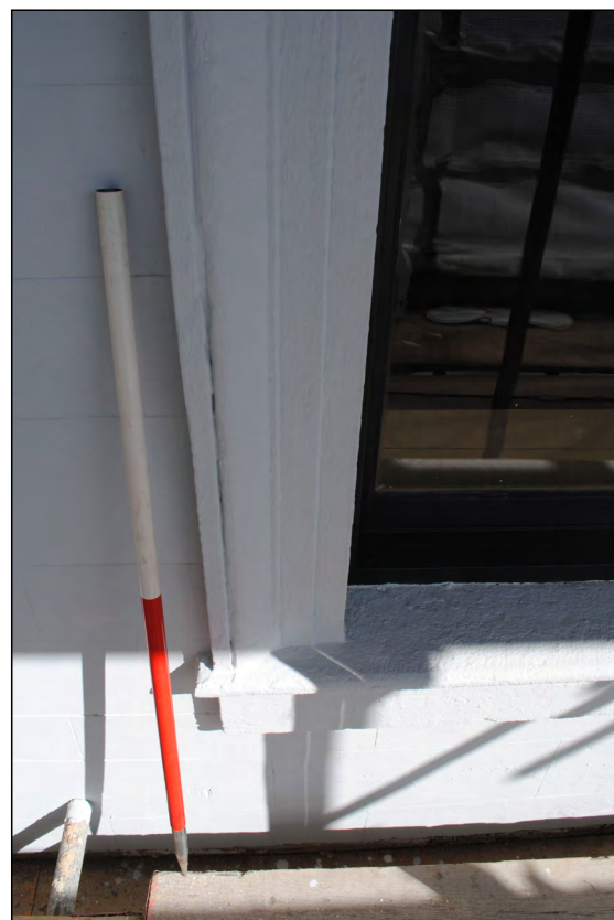
Photo 54. Exterior first floor, view looking NNW at finished architrave detail in easternmost window in the south wall of High Street West No. 2.
