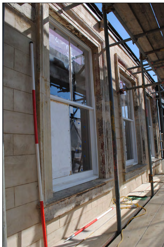
Photo 28. Exterior first floor, view looking NE at window repairs in south wall.
