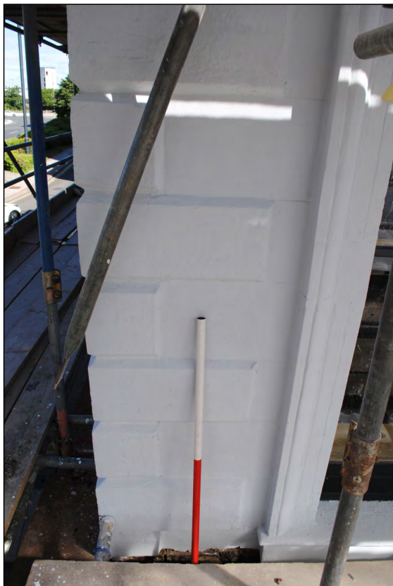
Photo 59. Exterior first floor, view looking NNW at finished quoin and architrave work in the SW corner of High Street West No. 1.
