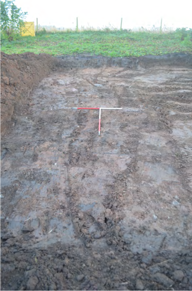
Photo 01. A strip of clay natural exposed within the building footprint. S view.
