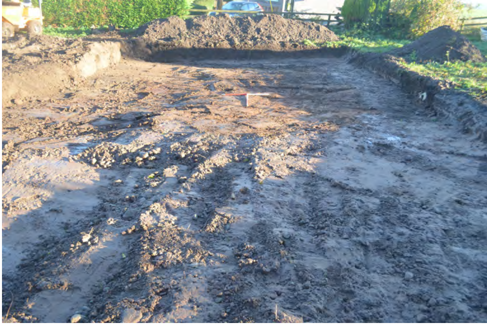
Photo 04. The complete building footprint stripped to natural or to height. E view.
