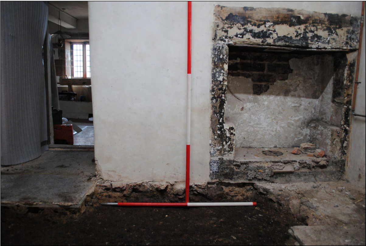
Photo 9. West facing section of the Butler's Pantry floor, following excavation of concrete debris and rubble layers.
