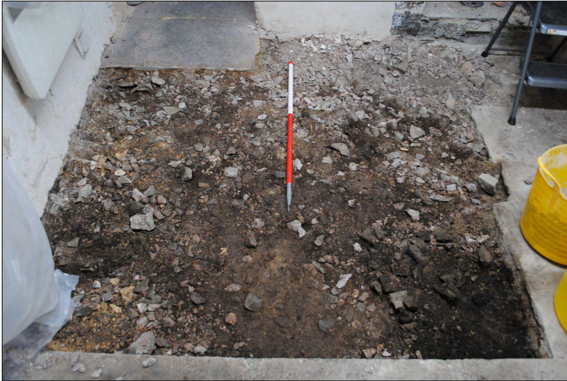
Photo 3. View looking east across the floor of the Butler's Pantry, following removal of concrete.
