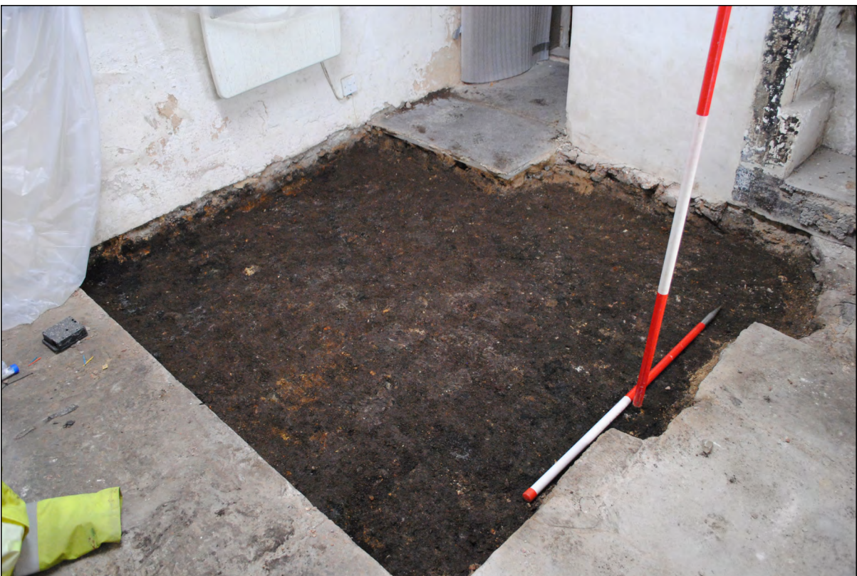
Photo 10. View looking north-east across the floor of the Butler's Pantry, following excavation of concrete debris and rubble layers.
