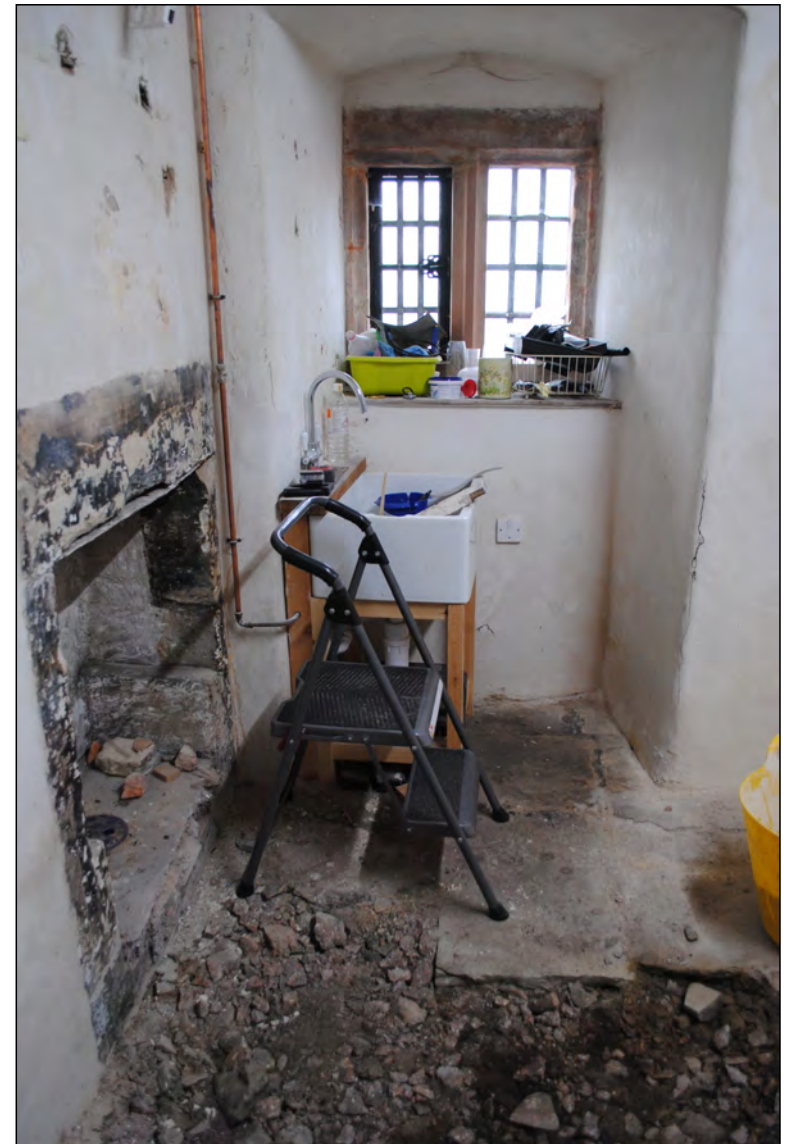
Photo 4. View looking south across the floor of the Butler's Pantry, following removal of concrete.
