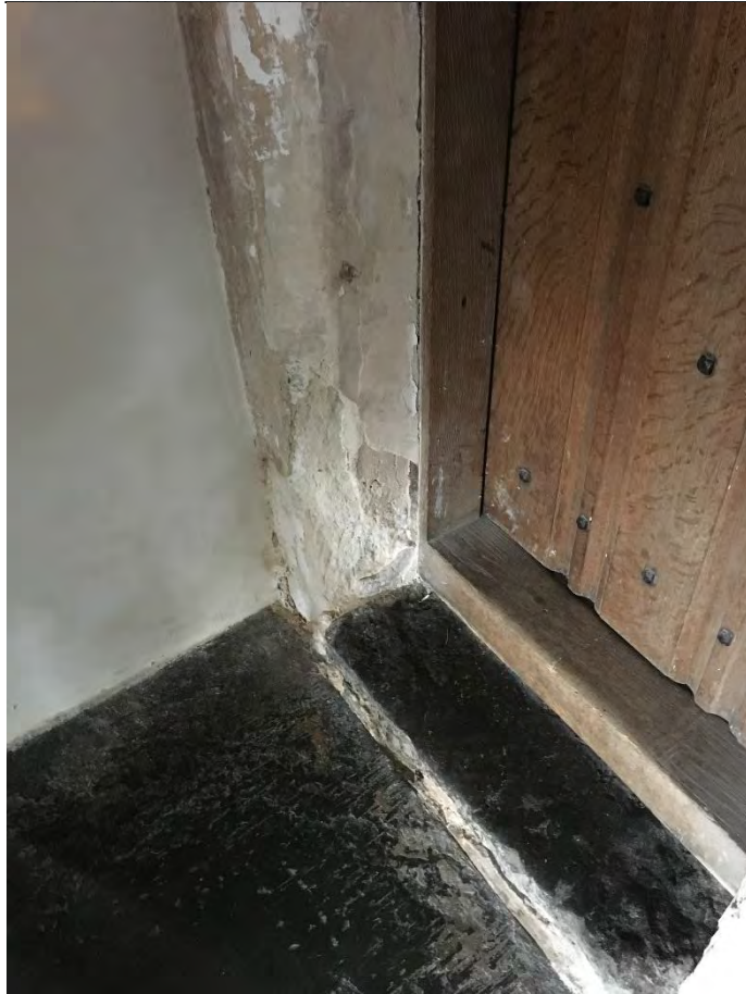
South-East corner: damage to the door jamb leading into the Pantry
