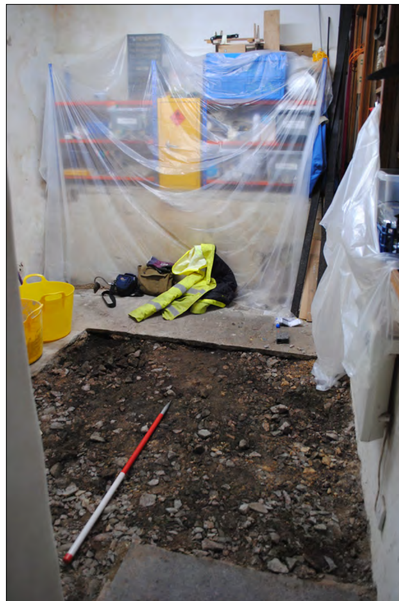
Photo 2. View looking WSW following the removal of concrete on the floor of the Butler's Pantry.
