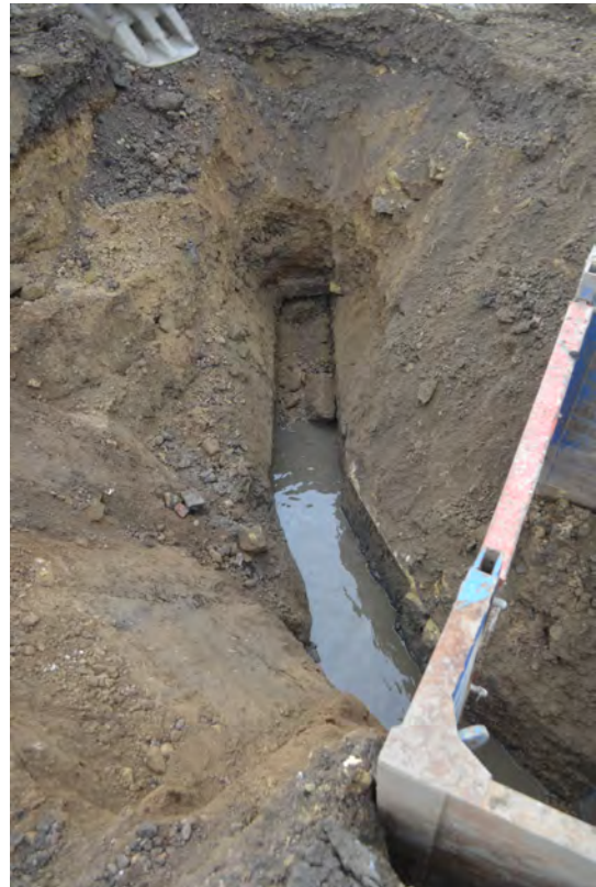
Photo 43. The NW-SE culvert leg, angling in stages after the angular direction change in Photo 42. SE view.
