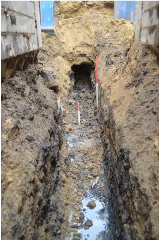
Photo 47. The NW-SE culvert, at the S extent of the site area. SE view.
