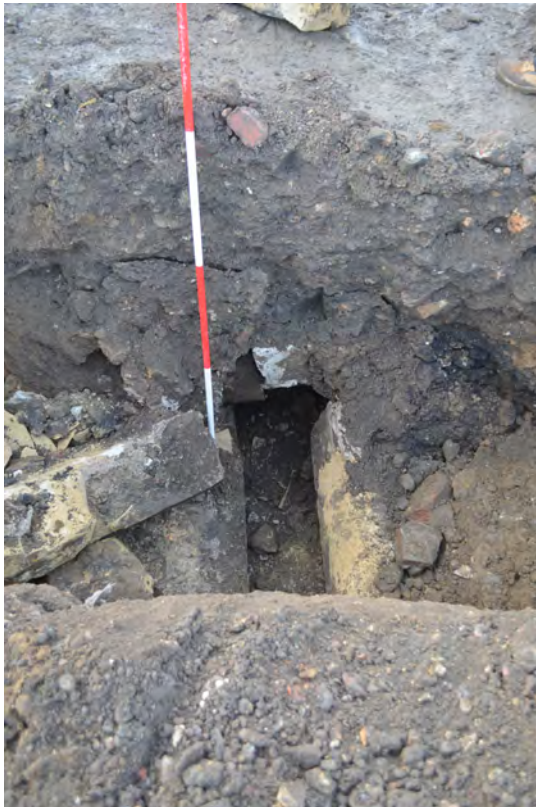
Photo 24. The culvert, with voussoirs for capping, exposed in a trial pit. S view.
