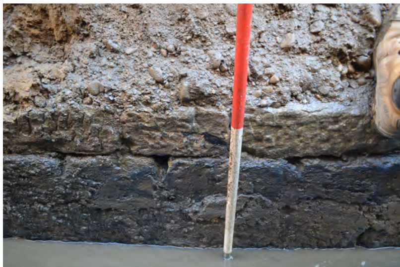
Photo 31. A section of culvert side wall towards the E end of site.
