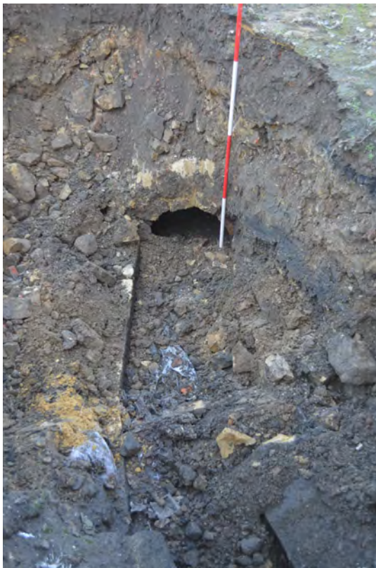
Photo 27. The culvert in the SW corner of site, showing vaulted capping. N view.
