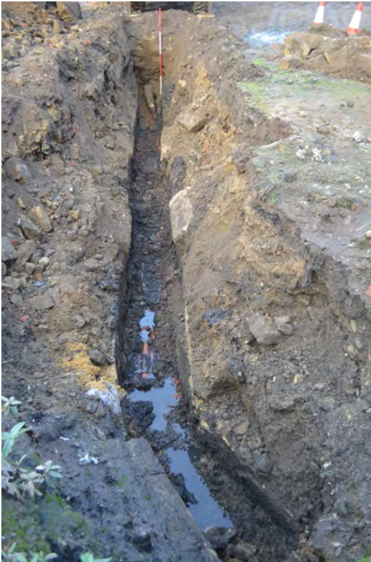
Photo 29. The culvert in the SW of site, with capping stones removed. N view.
