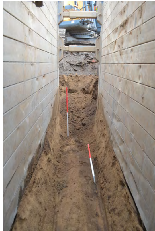
Photo 48. A trench excavated down to natural sand for a drainage run as part of the system of catchpits. SE view.
