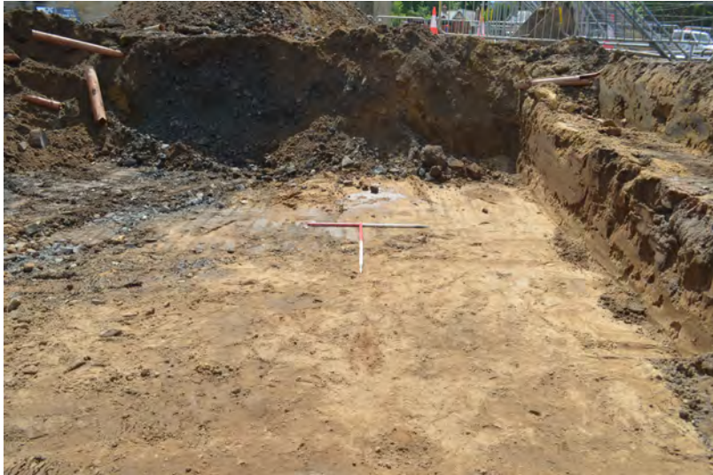
Photo 68. Excavations for the large water attenuation system at the E end of the site. SW view.
