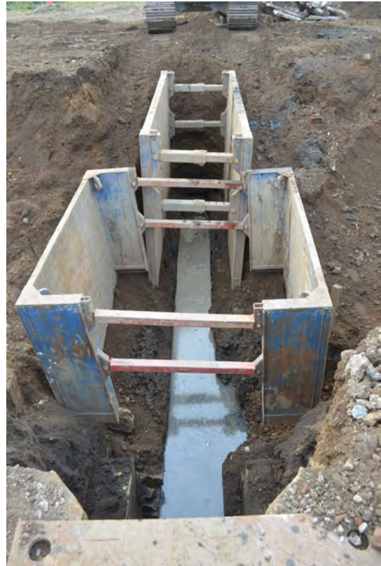
Photo 36. The culvert, viewed from the top of the larger part of the chamber, with the meeting of culverts visible within the square manhole box. SE view.
