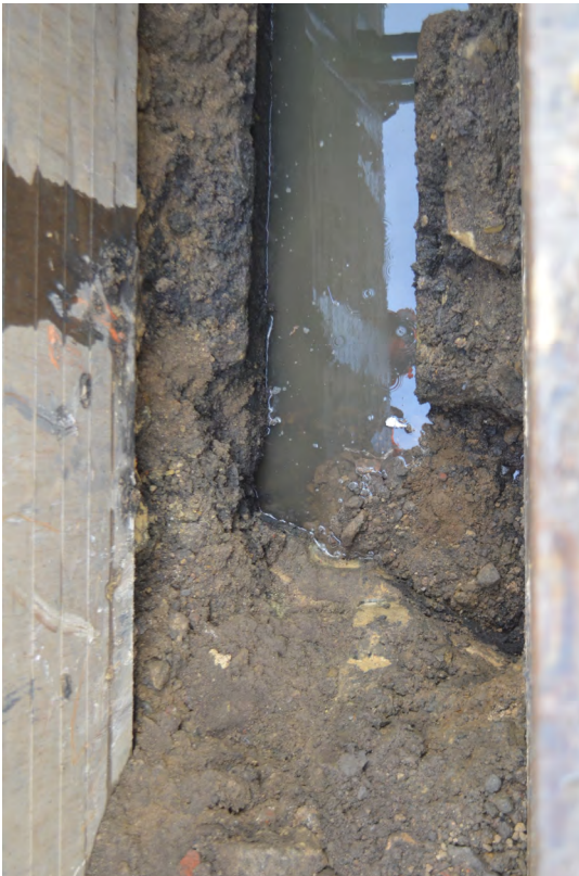
Photo 42. Vertical shot of the NW-SE culvert's angular direction change S of the chamber.
