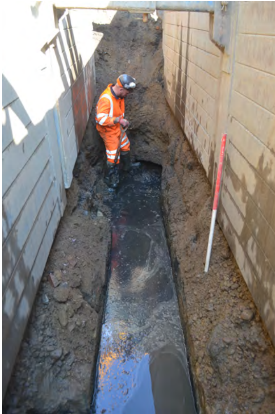
Photo 32. The culvert in the NE of site, gently angling to meet the NW-SE leg of the culvert. NE view.
