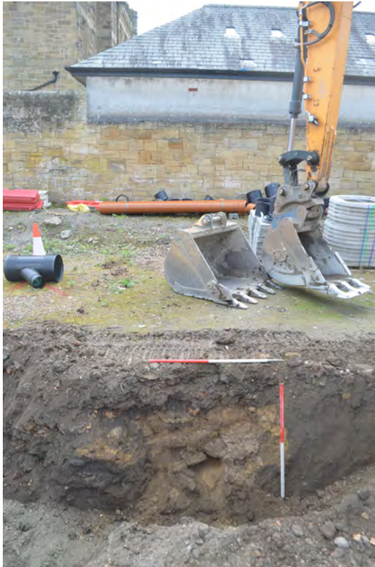
Photo 50. One of the four yard division walls [120] encountered between CP06 and CP09. SE view.
