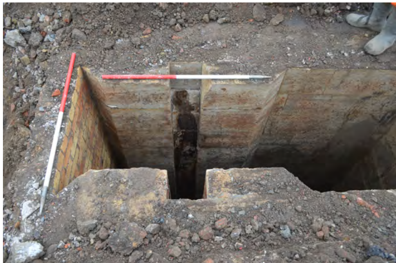
Photo 37. The larger part of the chamber, showing the sluice gate setting. SW view.
