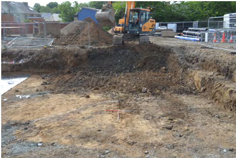
Photo 69. Excavations for the large water attenuation system at the E end of the site. SE view.
