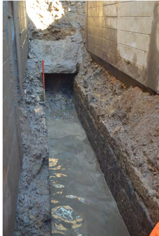
Photo 30. The culvert towards the east of site, with a flat capping stone visible E view.
