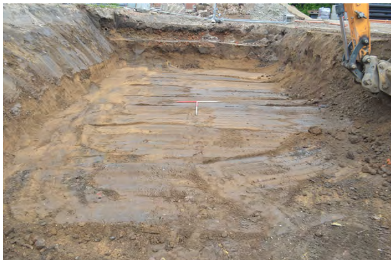
Photo 67. Excavations for the large water attenuation system at the E end of the site. SE view.
