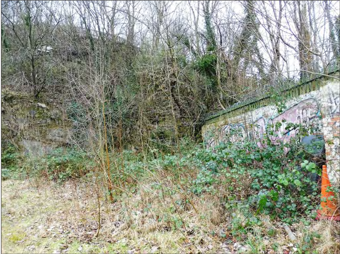
Photo 3: The southern end of the level part of the site showing the brick retaining wall and the quarried face cut into the slope of the valley side.
