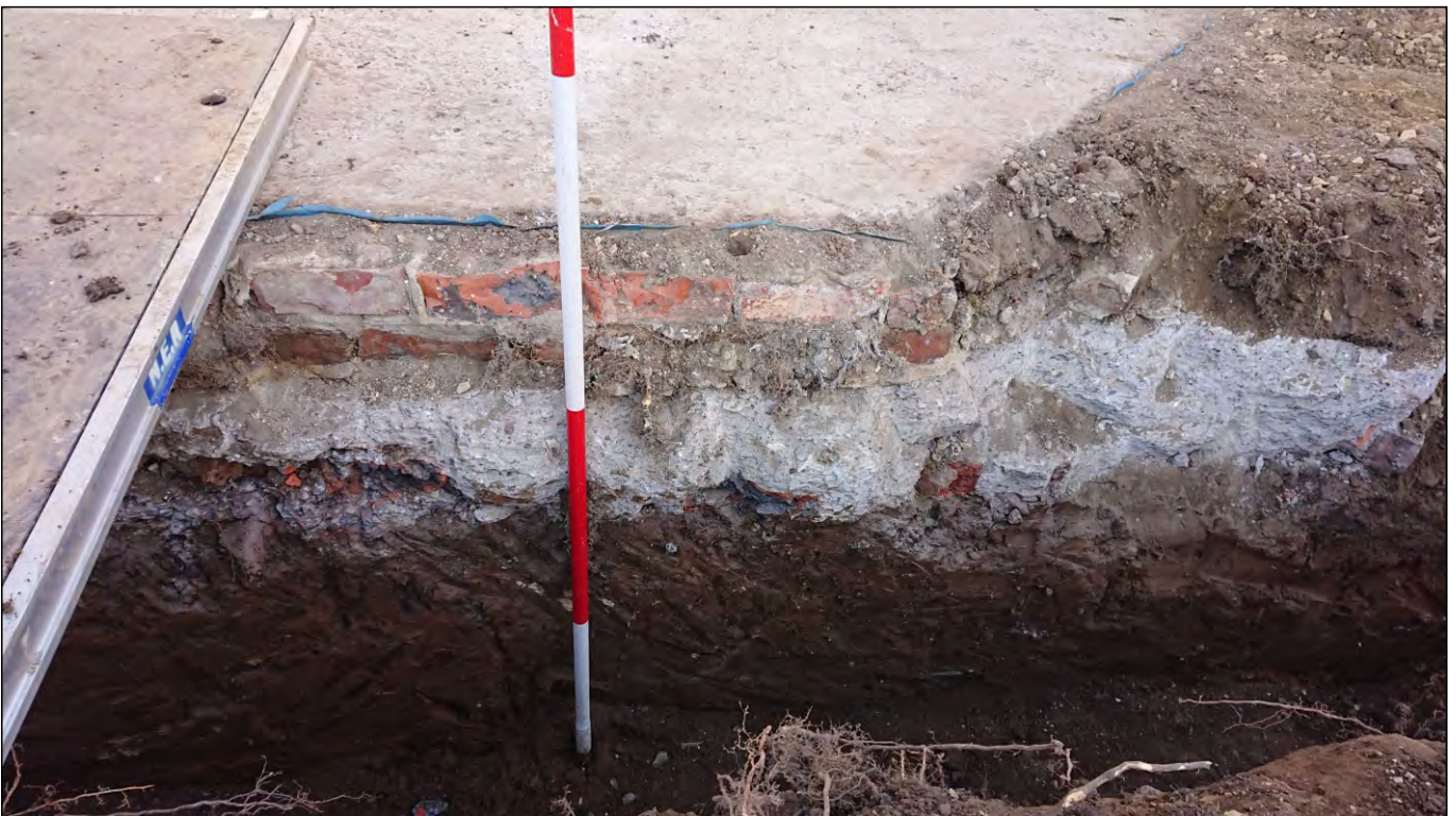
Photo 08. Foundation trench A-E, south facing section at west end of trench, showing foundation of recently demolished conservatory.
