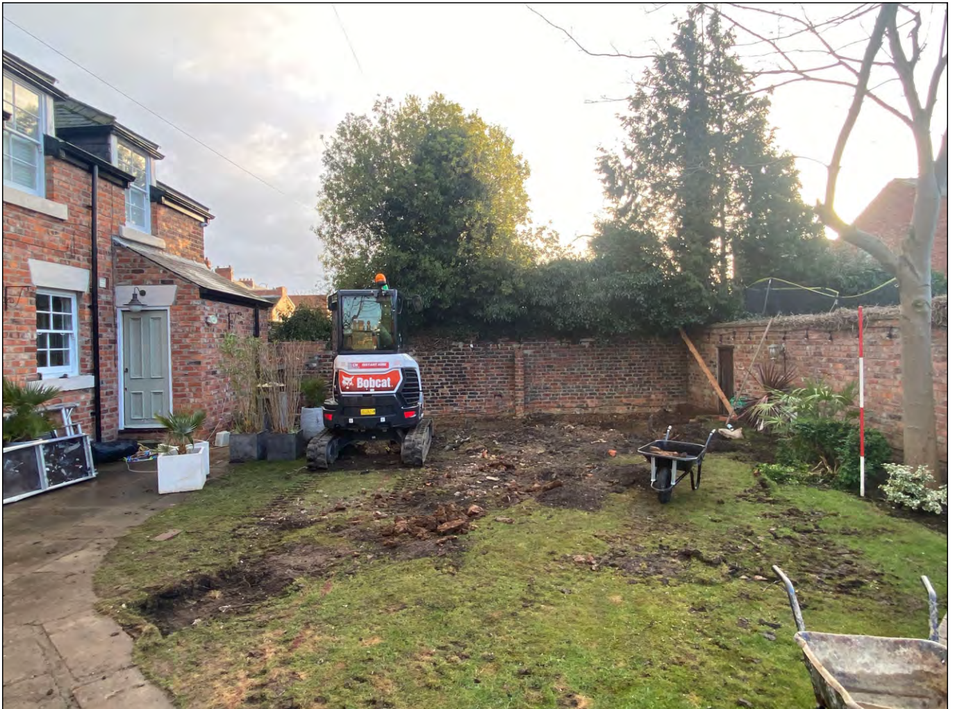
Photo 02. Broad view, looking east at the extension plot for Vanbrugh House at the start of foundation trenching.
