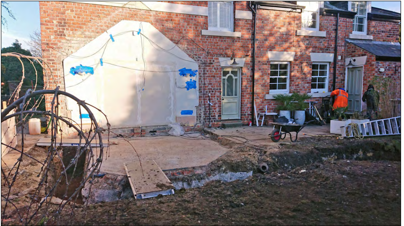
Photo 01. Broad view, looking north at new foundation trenches for proposed extension to Vanbrugh House, with the earlier footing of a recently demolished conservatory visible.
