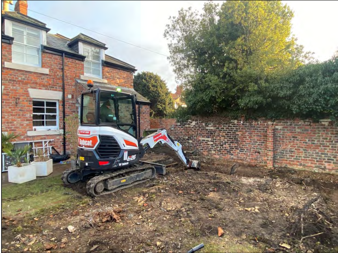
Frontispiece: View looking north-east during foundation trenching for an extension to Vanbrugh House, East Boldon in February 2023.
