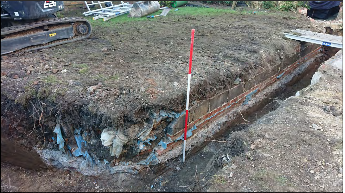
Photo 07. Foundation trench E-A, oblique view looking south-west, showing modern foundation of possible post-1970s garage structure.
