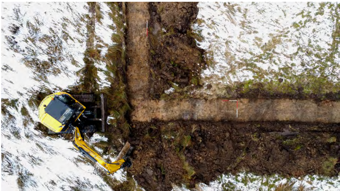
Photo 05: Drone shot showing detail of meeting point of trench legs. Drain cuts can be discerned in the middle-right of shot. West is top of shot.
