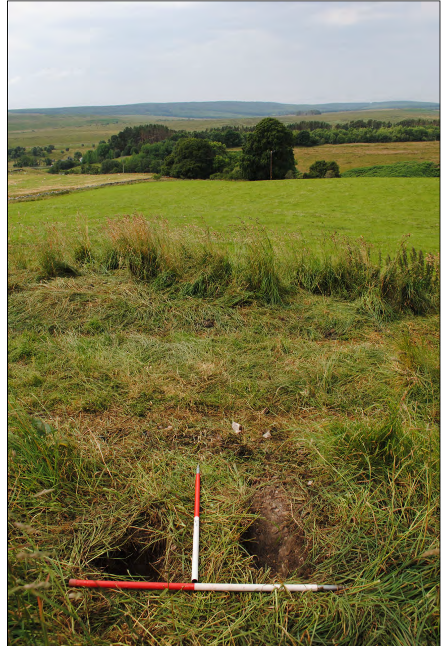
Photo 4. View looking east at excavated post-holes for interpretation panel, with vicus terrace in background.
