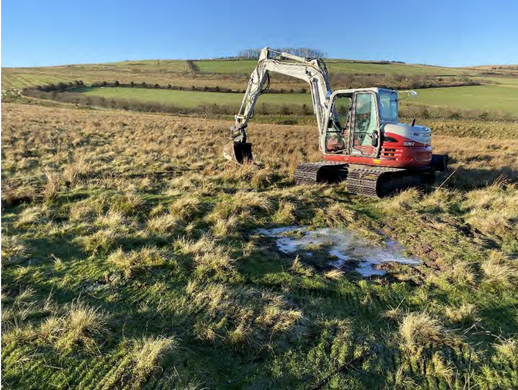
Photo. 09: View of machine work in progress in the west part of the site.
