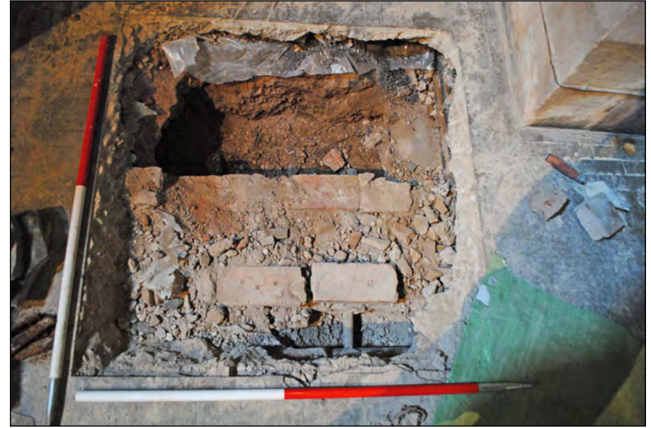
Photo 22. Test Pit 3, view looking west, following the removal of further rubble backfill, revealing some pipework and the aforementioned brick wall/conduit.
