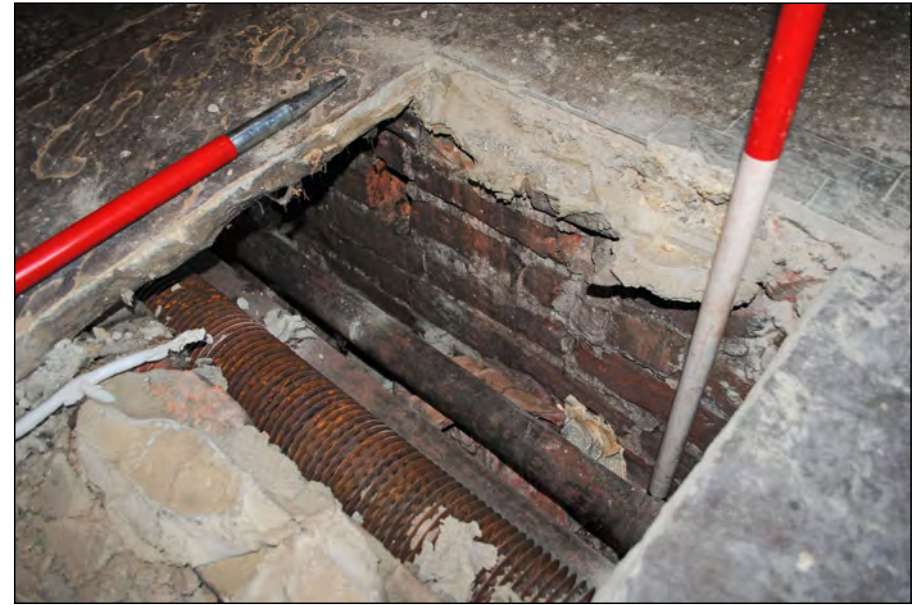
Photo 14. Test Pit 2, view looking south-east at north-facing C19 brick sleeper wall and exposed pipework below the flags in the central aisle.
