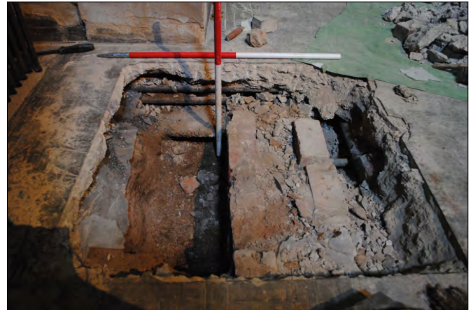
Photo 24. Test Pit 3, view looking north at exposed piping in south facing section and in NE corner of test pit running perpendicularly into brick wall/conduit.
