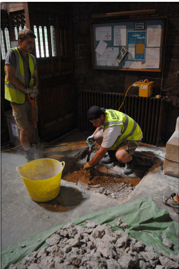
Photo 19. Test Pit 3, view looking WSW at the removal of concrete following breaking.
