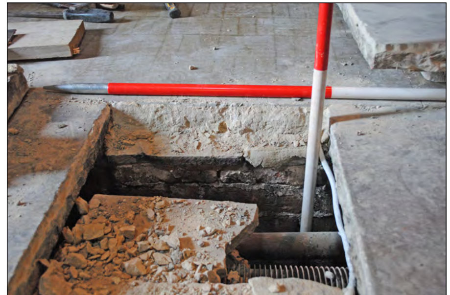
Photo 16. Test Pit 2, view looking north at south-facing C19 brick sleeper wall and exposed pipework below the flags in the central aisle.
