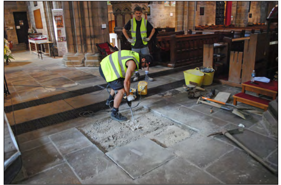
Photo 02. Test Pit 1, view looking south-west during removal of modern concrete beneath the flags.
