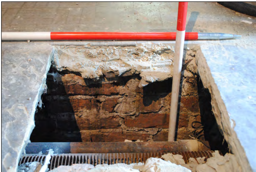
Photo 15. Test Pit 2, view looking south at north-facing C19 brick sleeper wall and exposed pipework below the flags in the central aisle.
