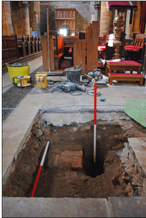
Photo 05. Test Pit 1, west view, showing east-facing section and partially truncated C18/19 brickwork and concrete below the floor.
