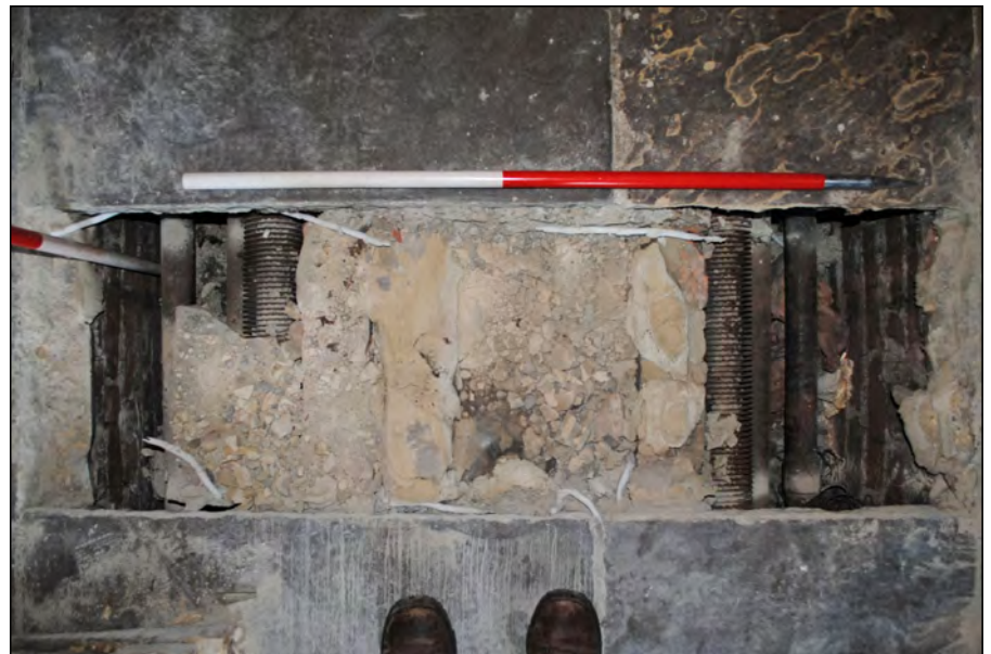
Photo 12. Test Pit 2, vertical view looking east, over the test pit with flags removed to reveal underlying pipework.
