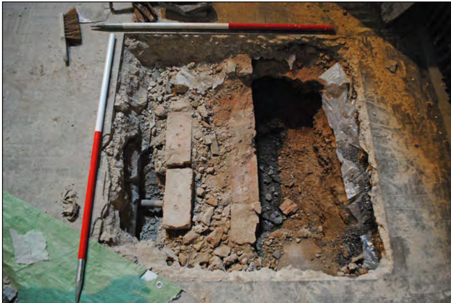
Photo 23. Test Pit 3, view looking south at exposed pipe running perpendicularly into brick wall/conduit.
