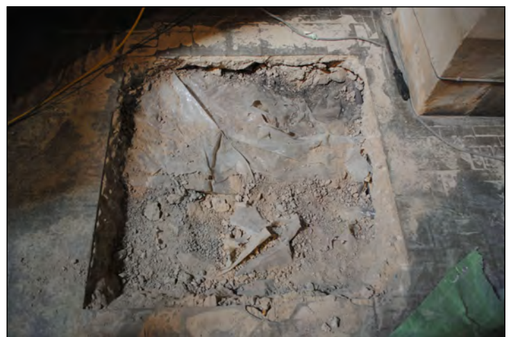
Photo 20. Test Pit 3, view looking west at plastic membrane, revealed beneath the concrete.
