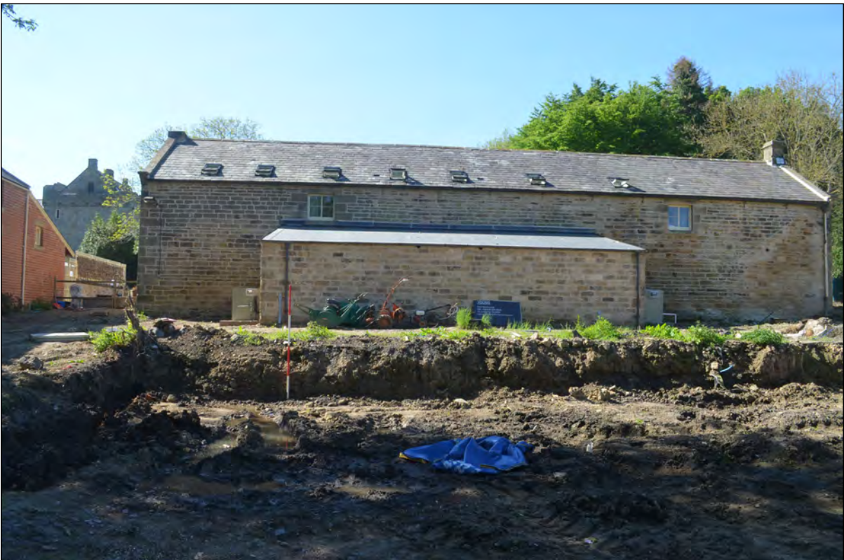
Photo 02. Pre-excitation shot. View looking south towards the Coach House, following demolition of the Pole Barn.
