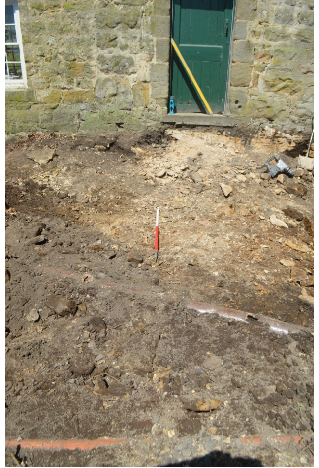
Photo 06. View looking north across the centre of the ground reduction. Modern service runs course through the area..
