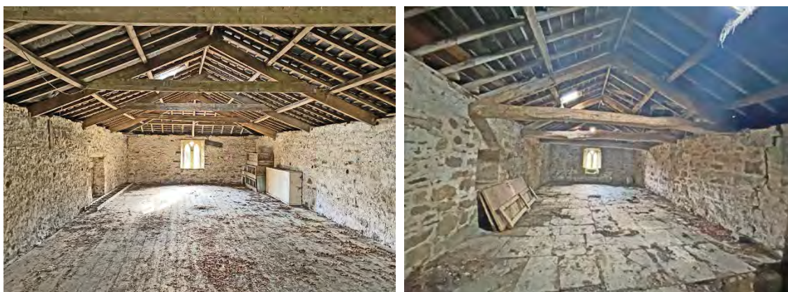
Illus. 06 (above left): Southward view of the southern, 19 th century extension to the barn.
