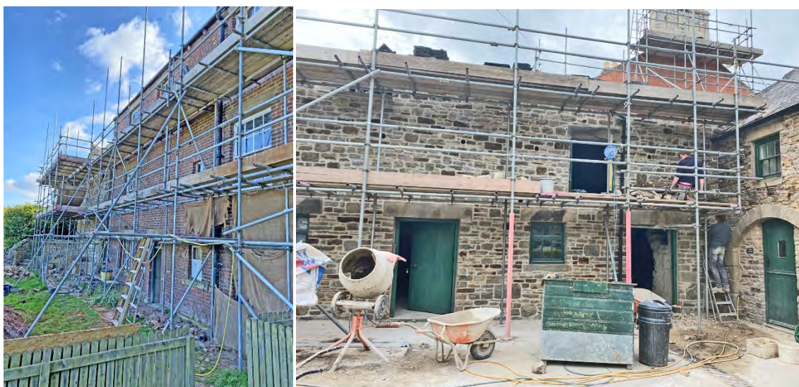
Illus. 12 & 13 (above left): The north-facing rear façade of the cross-wing of a 13 th -century house (rear) and main house (foreground) during consolidation works.
