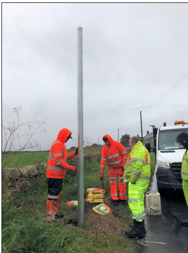
Frontispiece: View towards northwest showing installation of new road sign in progress.
