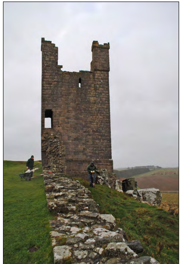
Photo 3. View looking SSW during excavations for a new safety sign on the north side of Lilburn Tower.
