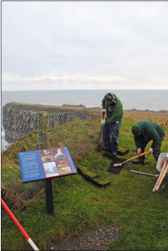
Photo 11. View looking ENE during deturfing for Test Pit 1, inside the existing north fence-line.
