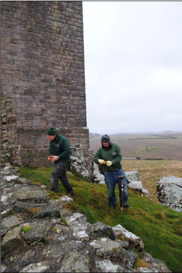
Photo 4. View looking southwest during excavations on the north side of Lilburn Tower.
