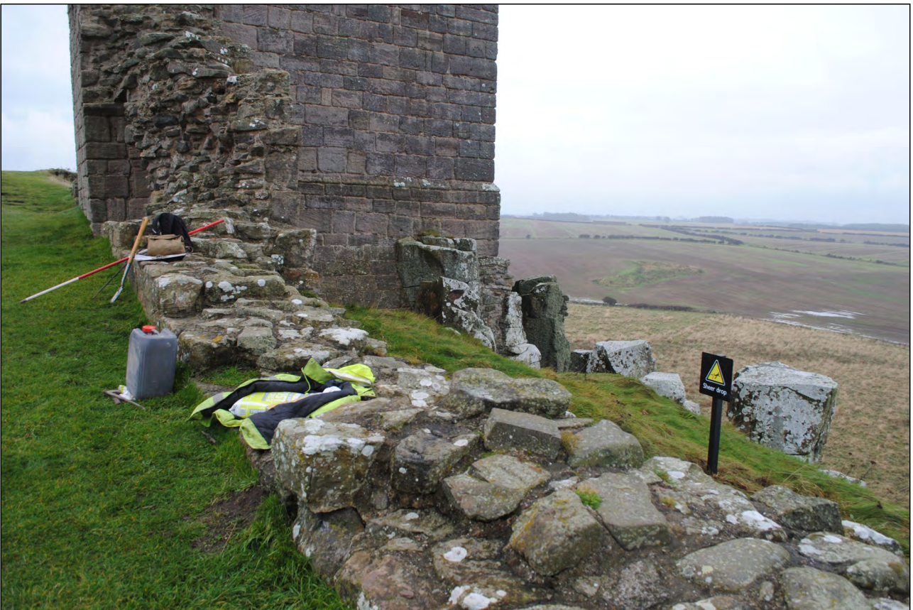
Photo 10. View looking southwest at newly erected safety sign on the north side of Lilburn Tower.
