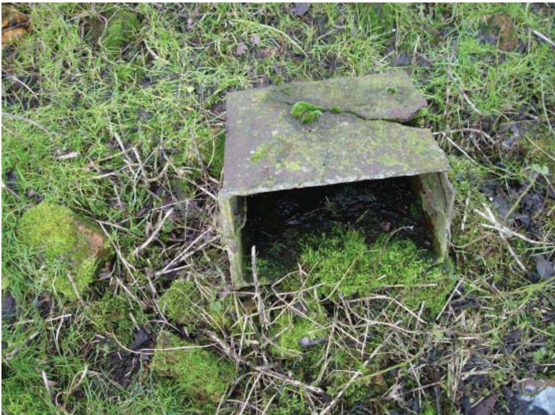
Plate 28: Cast iron cistern within enclosure
