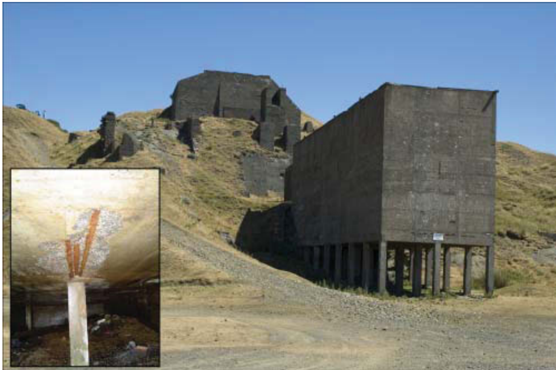
Plate 19: Concrete built stone crusher and sorter SO 5928 7752. The inset bottom left shows oxidisation of steel reinforcing bars creating flaking of the concrete. The structures above supported the overhead supply track from the quarry
