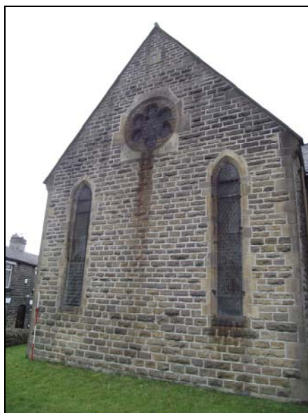
Plate 10, 3: view of the transept's gabled north elevation with multi-foil circular window, from the north northwest
