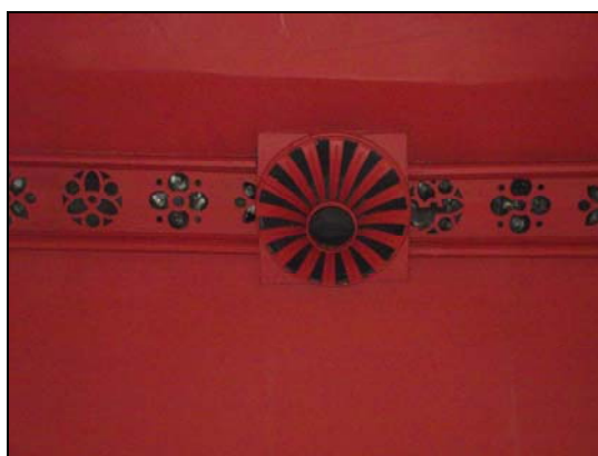
Plate 26, 168: Room 4b , Detail of the transept ceiling with decorative ventilator and fluted fan housing, from the west
