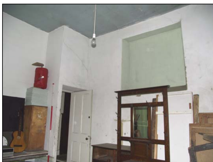
Plate 48, 125: View with the blocked window to the east wall (Rm. 26), from the northeast
