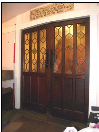
Plate 33, 161: view of the inner double doors to the main south entrance (Rm. 5), from the northwest
