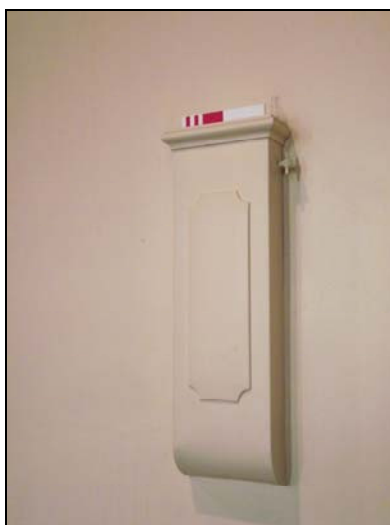
Plate 23, 126: room 4a, detail of one of the ventilators with a 'hand' knob, from the southeast
