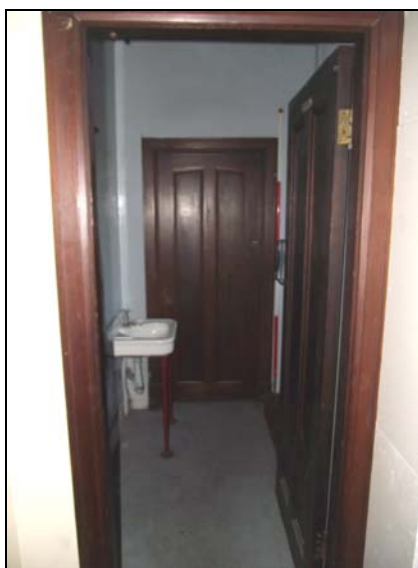
Plate 44, 109: View into the 'Gentleman' toilet (Rms. 19 & 20) with hand-basin and type 2 doors, from the south
