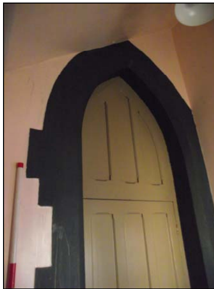
Plate 17, 94-5: room 1, view of the arched door way with 6 panel door into the church (transept), from the east
