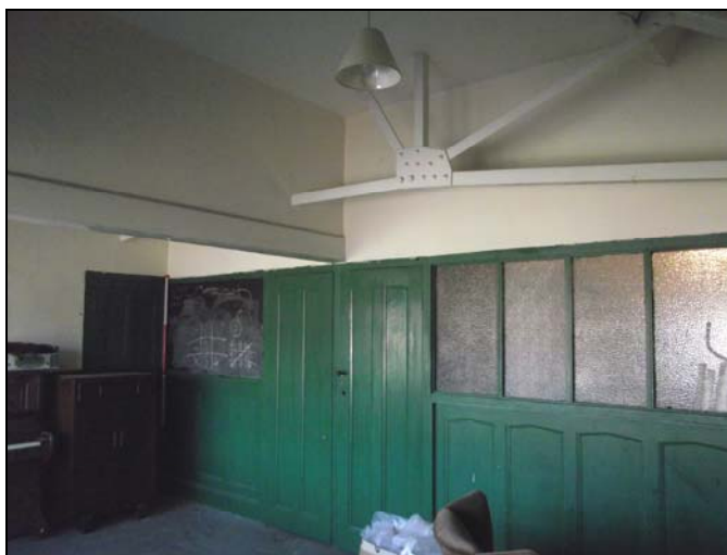
Plate 45, 114: view of the divider and roof trusses (Rm. 21) and the half glazed timber partition and type 2 doors, from the northwest
