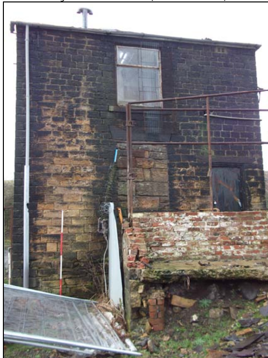
Plate 8, 54: View of the rear elevation of the Talley House, from the SSE
