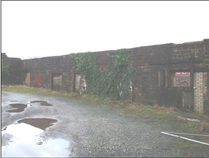
Plate 9, 55: view of the external wall of the recessed 5 bay, 3 storey building, from the SW
