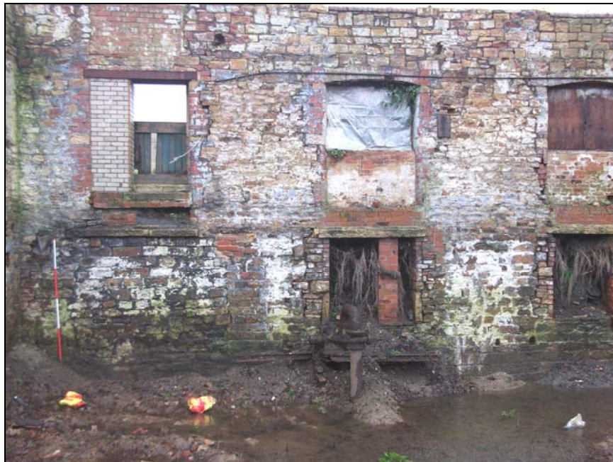
Plate 20, 22: General view of the 'internal' NE wall with inserted CI pipe to the ground floor windows, from the southeast
