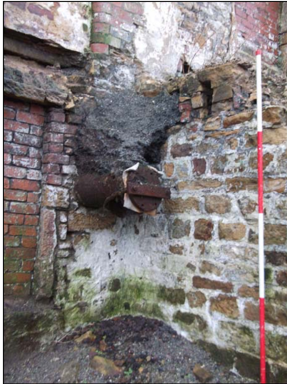
Plate 21, 40: Detail of the former work's ground floor with sealed cast iron pipe, from the south
