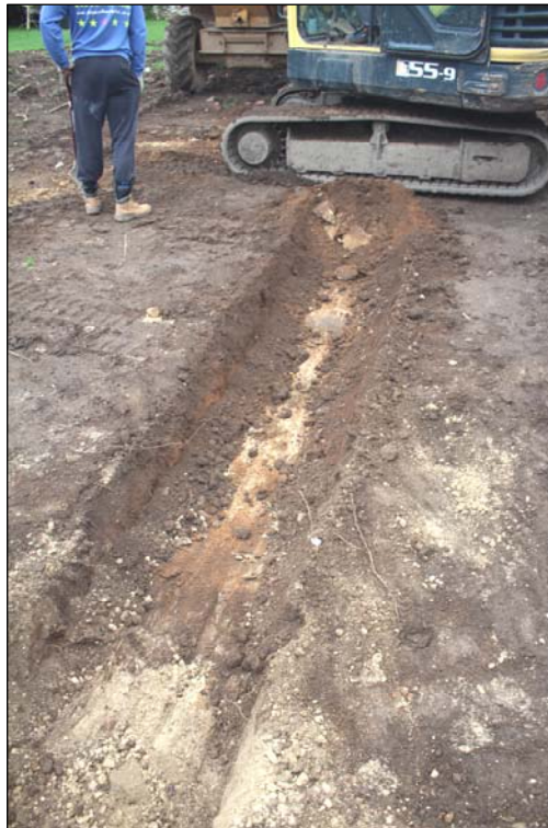
Plate 2: typical foundation excavation view, before the excavation of the natural limestone, looking northeast
