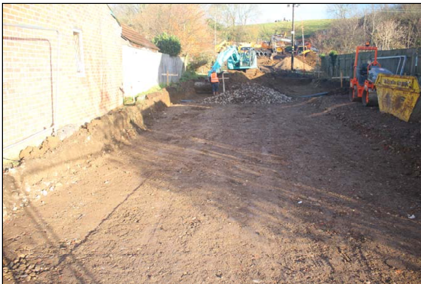
Plate 6: further excavation view during the site strip of access road off Meagil Rise, looking northwest
