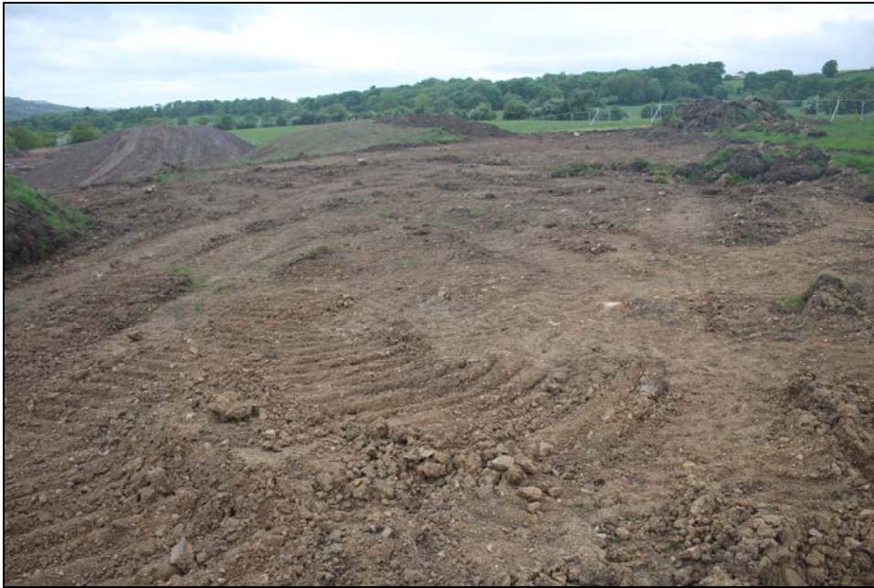
Plate 27: post excavation view following the top soil strip towards the northeast corner of the site, looking northwest
