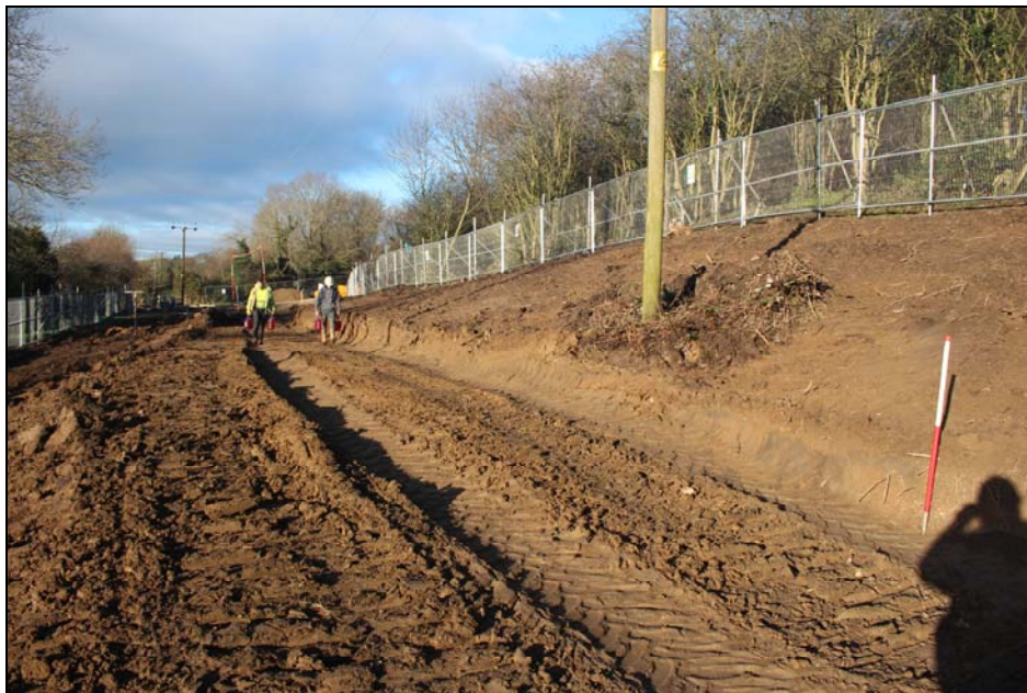
Plate 10: further general view of the east-west access road with truncation of colluvial/glacial deposits, looking west
