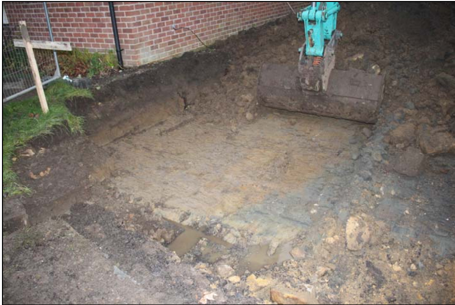
Plate 5: excavation view during the site strip of access road off Meagil Rise, looking northwest
