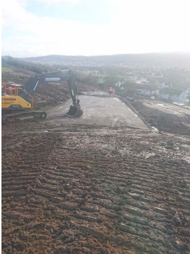
Plate 23: view towards a fill zone during earthworks excavations, looking east down the Wharfe valley
