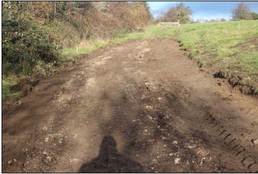
Plate 11: general view of the re-surfacing of the 'farmer's track up slope, looking northwest
