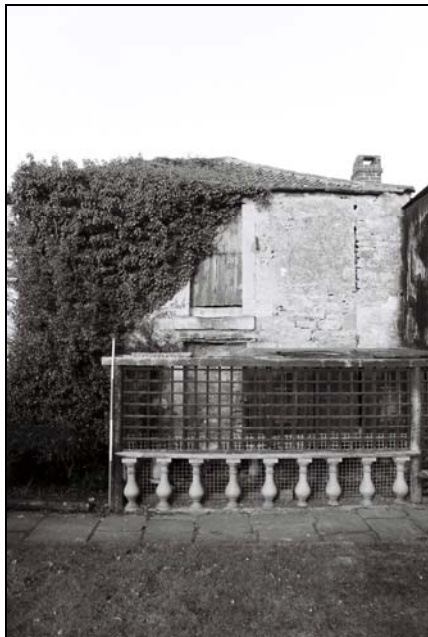
Plate 56 , 280: the barn (Blg.7), view of the partially obscured south elevation, from the south
