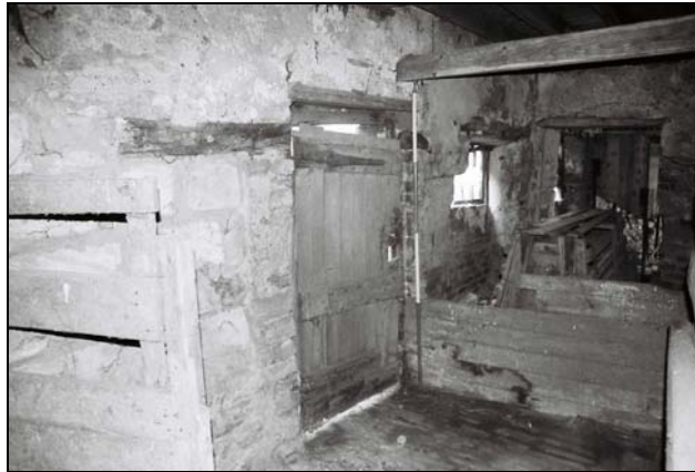
Plate 58 , 245: the barn (Blg.7/45), general view with the blocked window and probably heightened doorway with stone setts to the floor from the southwest
