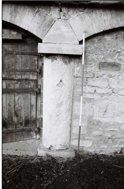
Plate 63 , 288: the shelter shed (Blg.8), external detail of one of the cylindrical stone piers with square capitals, from the south
