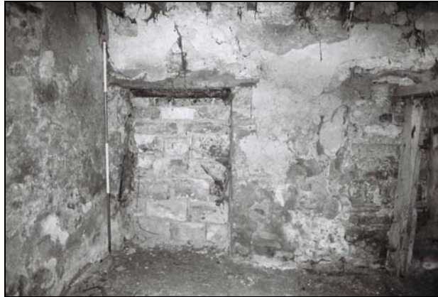
Plate 57 , 240: the barn (Blg.7/39), view of the blocked doorways to the west wall, from the east
