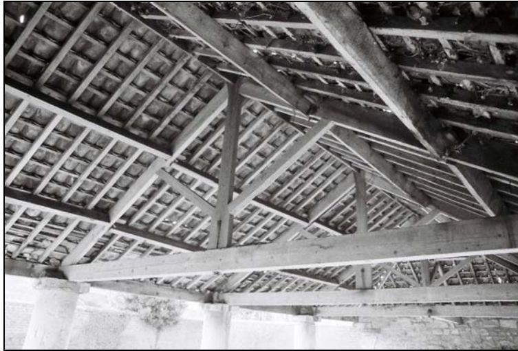
Plate 71, 268: the shelter shed (Blg.9), general view with the exposed roof, from the north east
