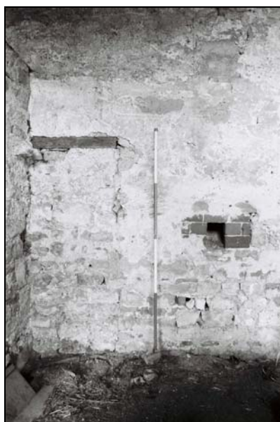
Plate 61 , 257: the barn (Blg.7/44), detail of the blocked opening and brick opening to the west wall, from the east
