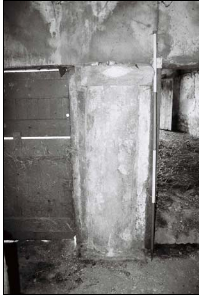
Plate 66 , 265: the shelter shed (Blg.8), detail of one of the protruding stone piers to the south wall, from the north
