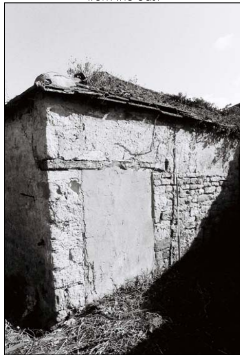
Plate 65, 314: the shelter shed (Blg.8), view of the west elevation with an inserted and blocked doorway, from the northwest
