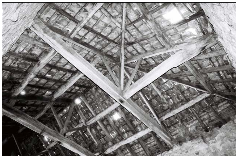
Plate 59 , 305: the barn (Blg.7/44), view of the hipped roof from the ground floor, from the northeast
