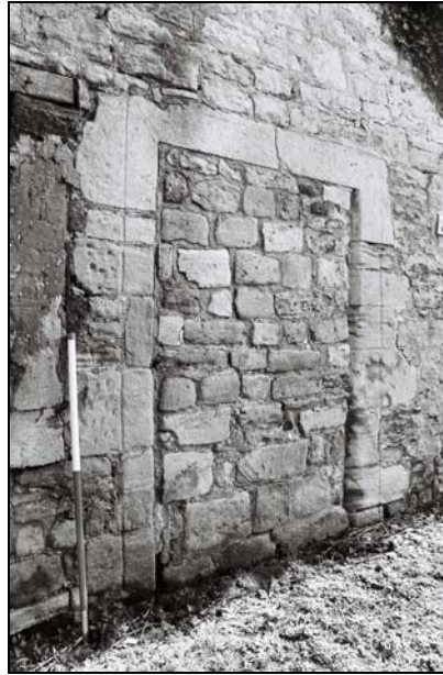
Plate 55 , 306: the barn (Blg.7), detailed view of the chamfered doorway [8], from the northwest
