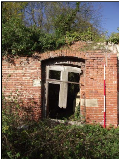
Plate 29 , 29: view of the doorway [3] which now accesses building 2 - The Fernery, from the southeast
