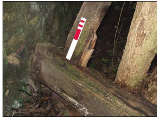
Plate 22, 123: detail of the tie-beam and post, from the Northeast (0.2m scale), from the northeast
