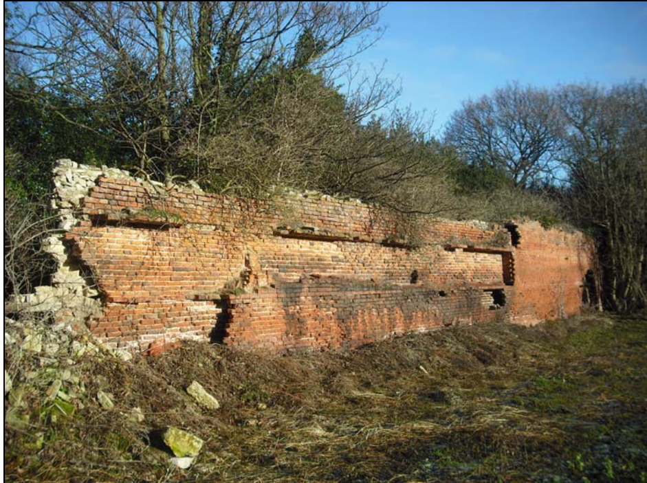
Plate 1: view of the south facing elevation of the north wall, with exposed heating ducts
