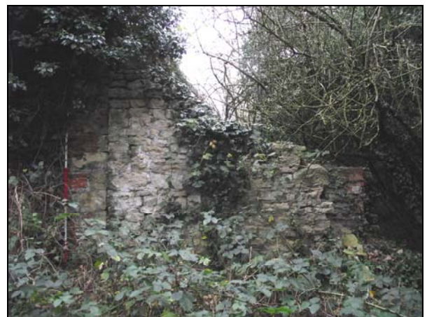
Plate 24, 142: View of the quoin corner of the northeast wall with the bothy's (building 3) limestone wall abutting, from the northeast
