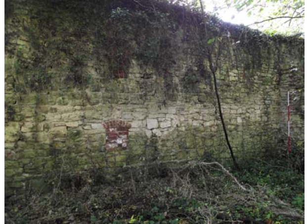
Plate 14 , 12: View of the northwest wall, northwest elevation with the blocked arched alcoves [35], from the north
