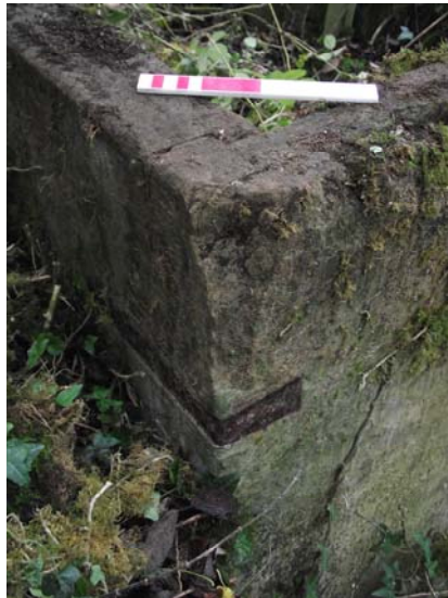
Plate 21, 121: detail of the cistern's [7] iron dovetail tie and rebated joint to the sandstone sides, from the west (0.2m scale)
