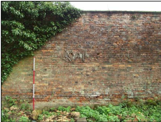
Plate 3, 4: detail of an exposed section of the external SW wall, from the west southwest
