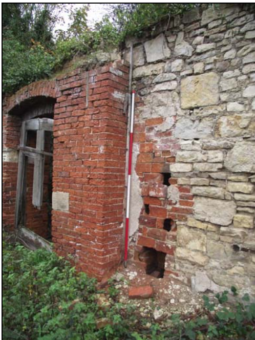
Plate 9, 77: detail of the part eroded heating duct within the NW wall, (SE Elevation), from the east
