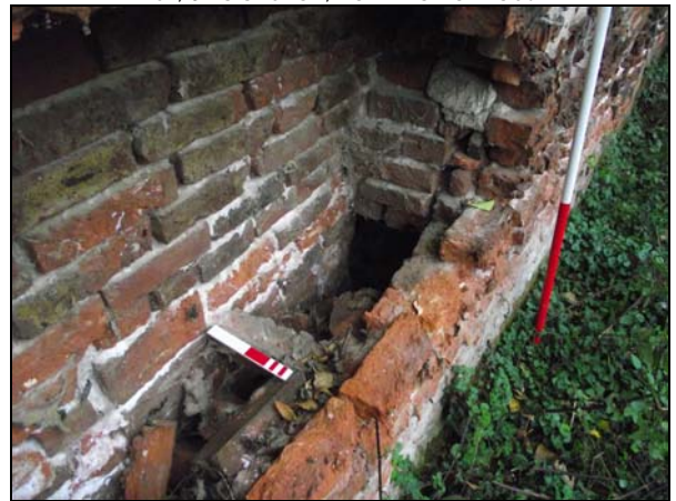
Plate 12, 73: Detail of the exposed heating duct above the twin furnace duct [33] (NB Plate 6)
