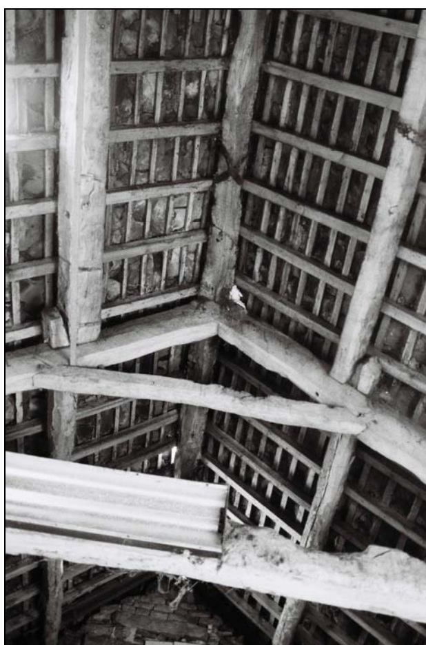
Plate 14, 55: View of the roof collar and purlins (Truss 2) and cross brace to the ridge purlin, looking southeast
