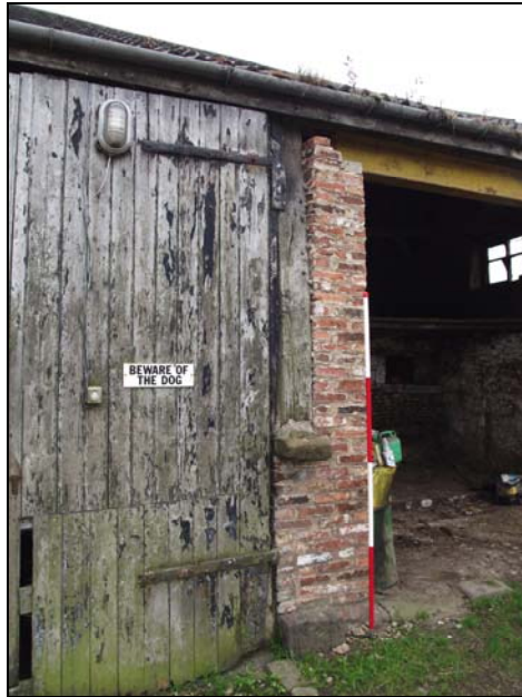
Plate 4, 7: detail of the post and post pads [2] with 2 sets of dowel holes, looking southwest
