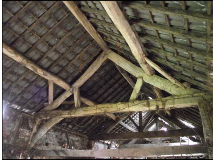
Plate 13, 38: General view of roof with truss T3 and T1-2 in the background, looking east
