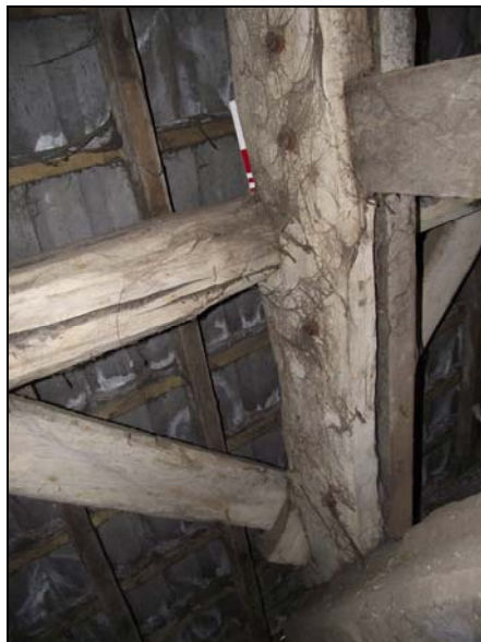
Plate 18 , 57: detail of the carpentry joints to the south side of truss T4, looking southwest
