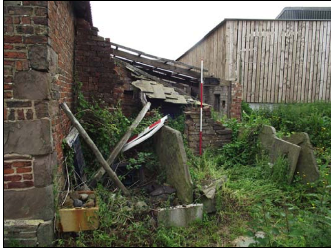
Plate 7, 11: view of the collapsed pigsty (Blg.2), looking east
