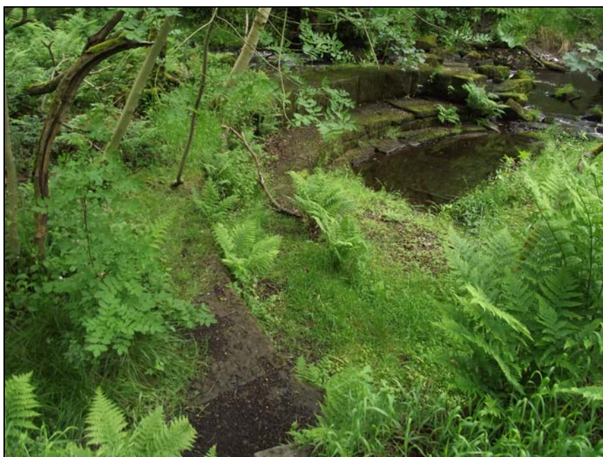
Plate 1: the curved Longworth Mill weir [5] represented by large ashlar sandstone blocks, looking northeast
