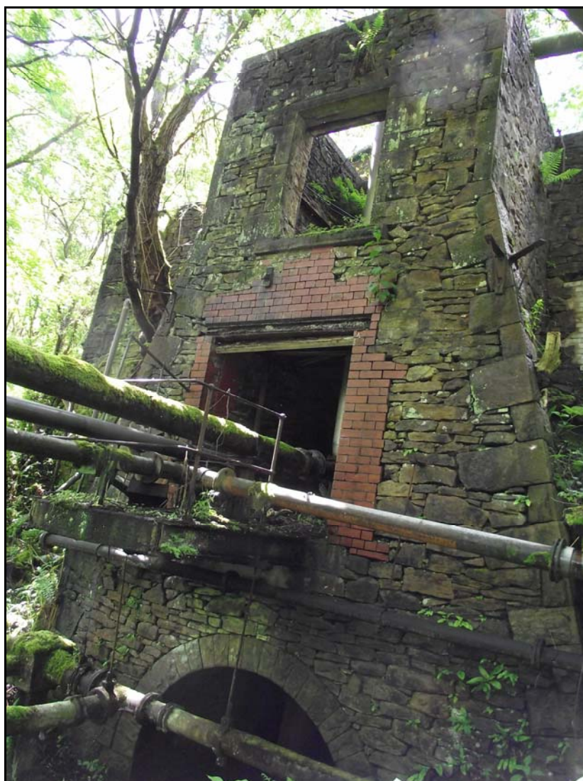
Plate 4: view of building 1E with its arched mill stream, from the north
