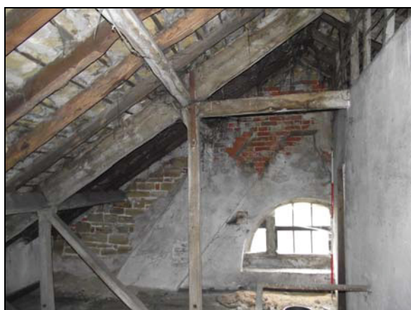
Plate 30, 83: General view of the store rooms and northwest gable wall, which reveals the brick chimney flues and solid rubble walls, from the southeast
