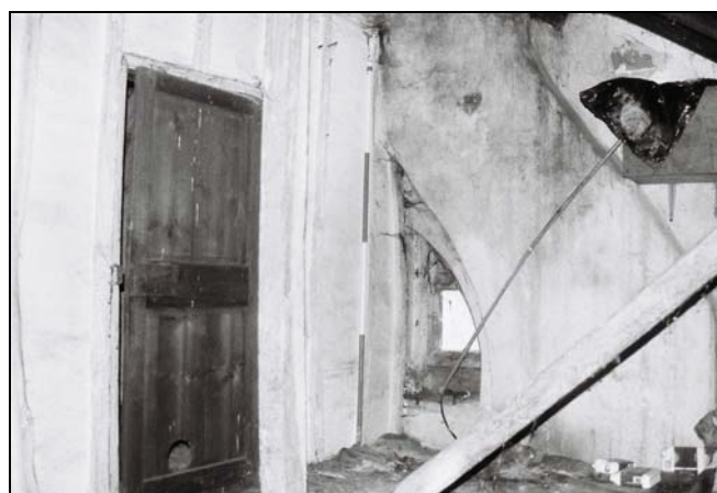
Plate 27, 70: General view with single light window and internal chimney, from the southeast
