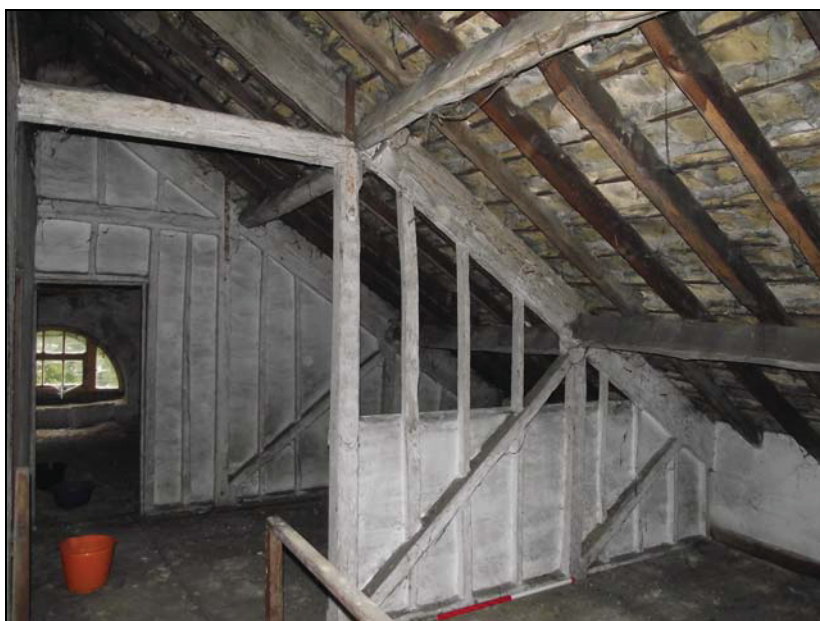
Plate 25, 146: General view with the half lathe and plastered walls, from the north
