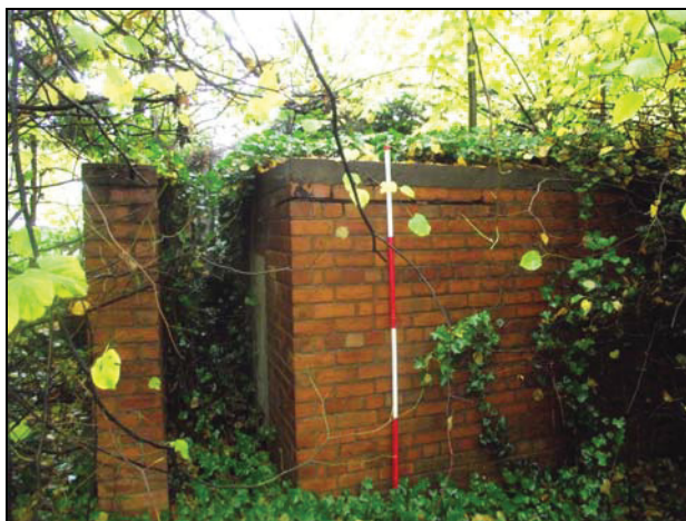
Plate 47, 167: General view of the external walls and blast wall, from the south
