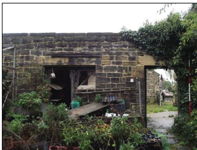
Plate 34, 157: Building I, View of the Southwest Elevation with doorway and door/window opening, from the southwest
