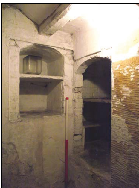
Plate 12, 34: View of the arched alcoves originally probably representing lockable spirit cupboards [1-2], from the north
