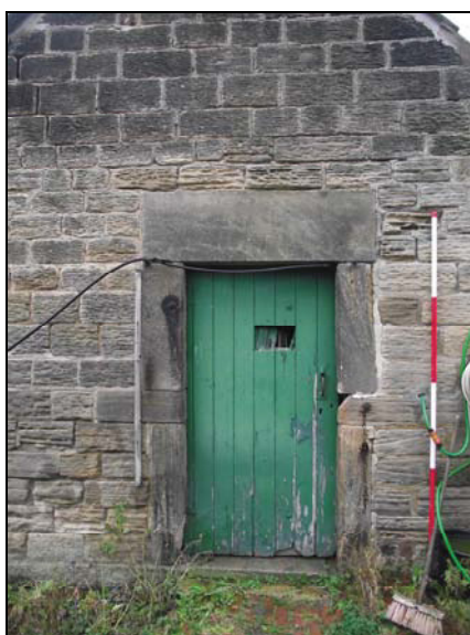
Plate 36, 105: Detail of the doorway [17] with its interrupted ashlar surround, from the southwest
