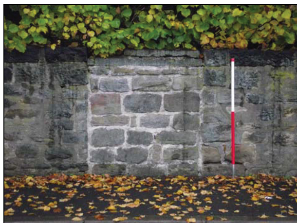
Plate 49: view of the block access point into the air raid shelter (Blg. H) from the southeast (Spring Lane)
