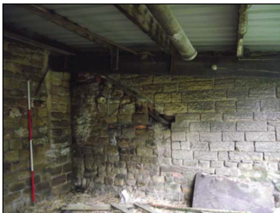
Plate 41, 106: General view of the once exterior walls of buildings C1 & C2, with inclined roof scar of former pigsties, from the north northeast
