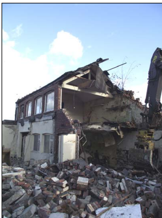
Plate 4 , 71: General view of building A with King-post roof truss, from the southwest
