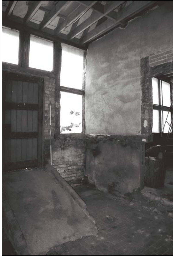
Plate 15, 32: view of the inserted doorway and the NW corner, from the southeast
