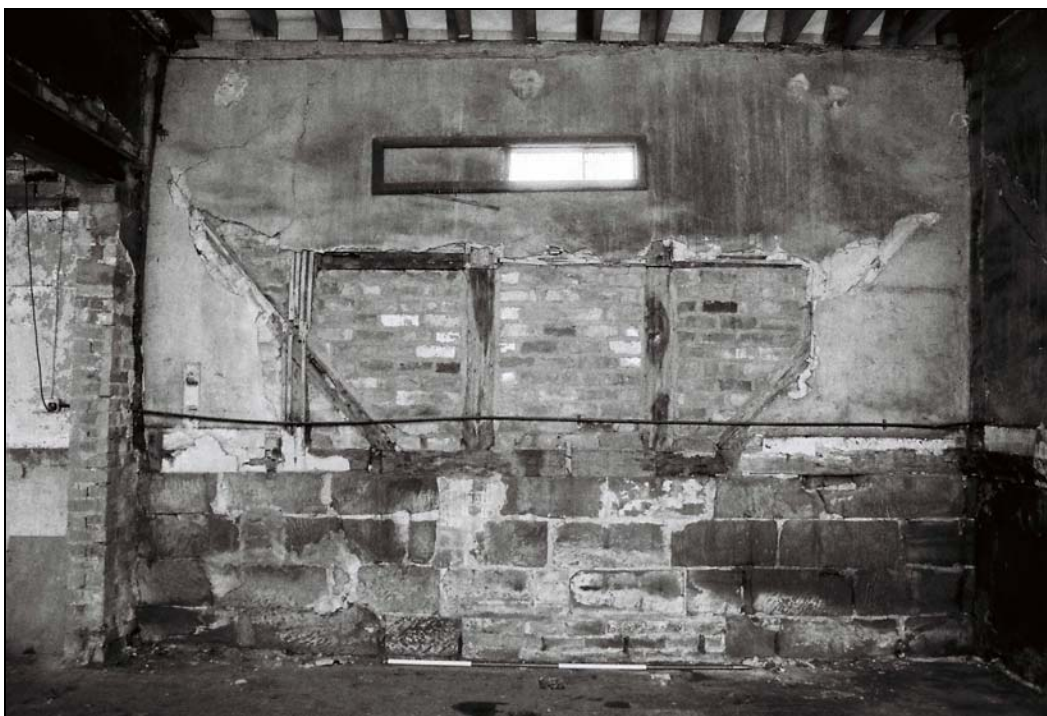
Plate 10, 25: view of the east wall with original oak walling with brick infill/noggin, from the west
