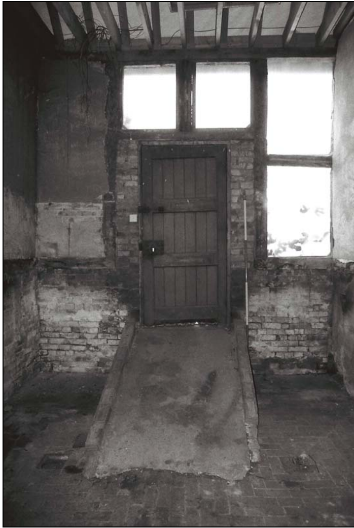
Plate 13, 31: view of the inserted doorway and the NW corner, from the southeast
