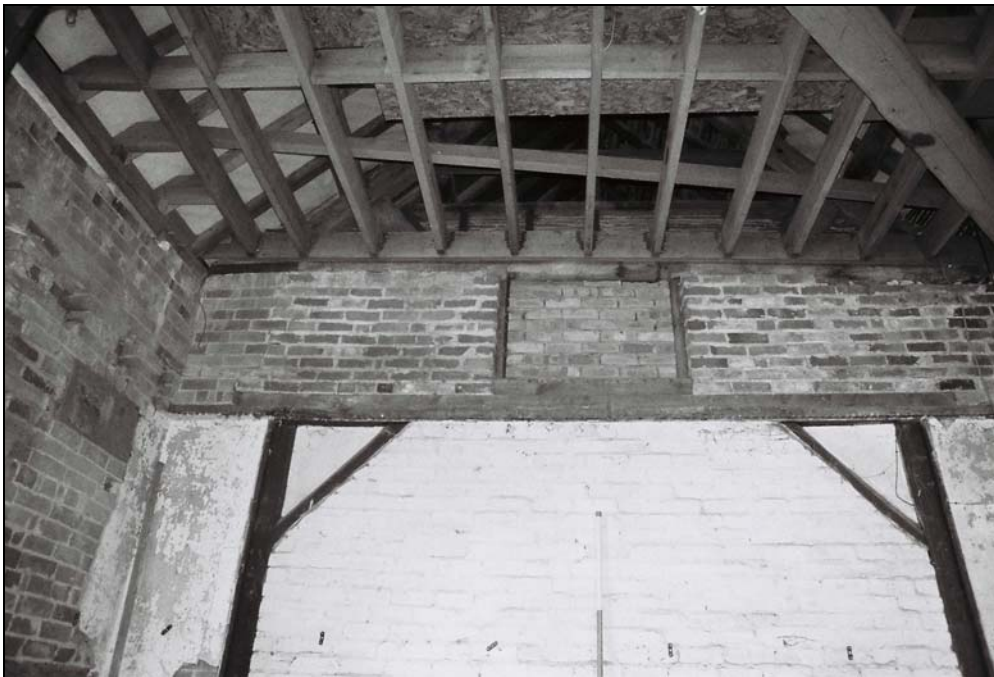
Plate 8, 15: view of the blocked opening [1] with pitching hole [2] above, from the west
