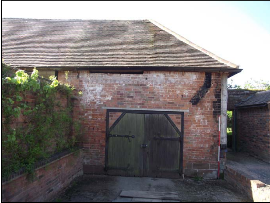
Plate 5, 1: view of the north elevation with inserted doorway and flue scars beneath the eaves, from the north
