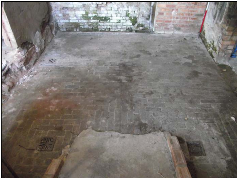
Plate 14, 39: view of the brick set floor with stall drains, from the west
