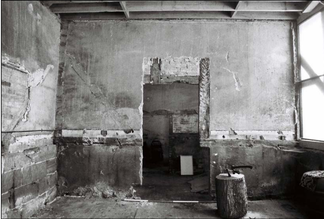
Plate 11, 24: View of the south wall with the straight braces of the framing visible below the plaster, from the north
