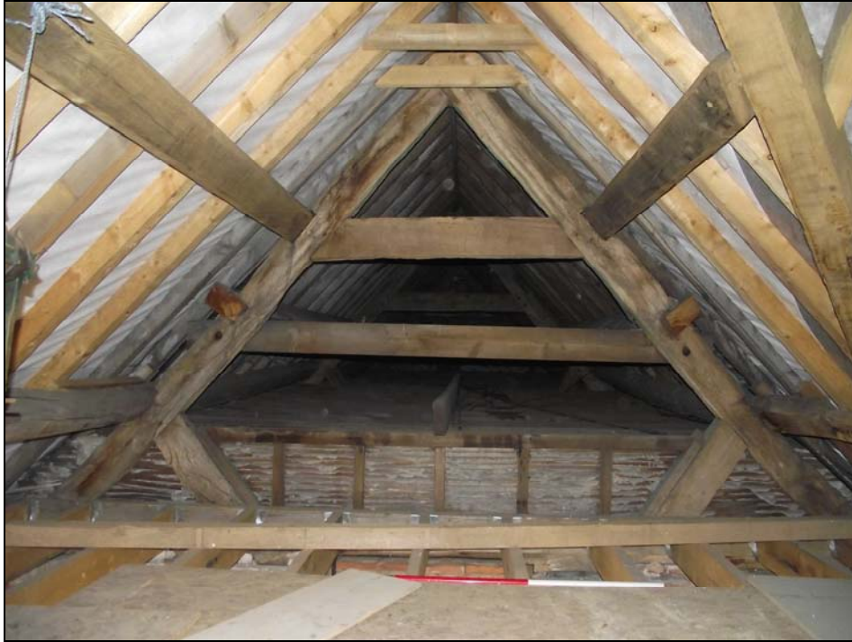
Plate 21/55: View of the surviving roof truss T1, from the west looking into the phase 4 extension (in separate ownership)
