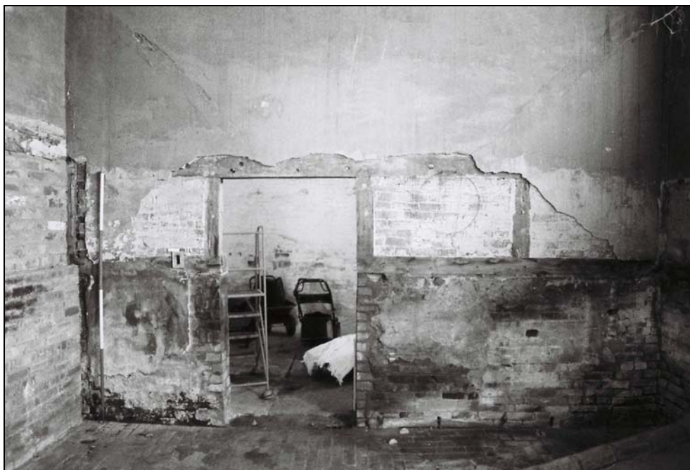
Plate 17, 35: room 3, View of the south wall with exposed timber and brick noggin, from the north
