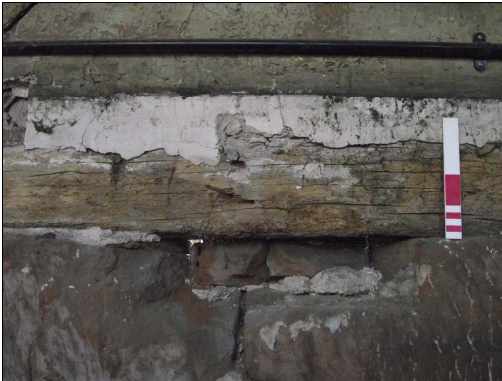
Plate 12, 52: Detail of the recess [3] to the east wall below the sill beam, from the west
