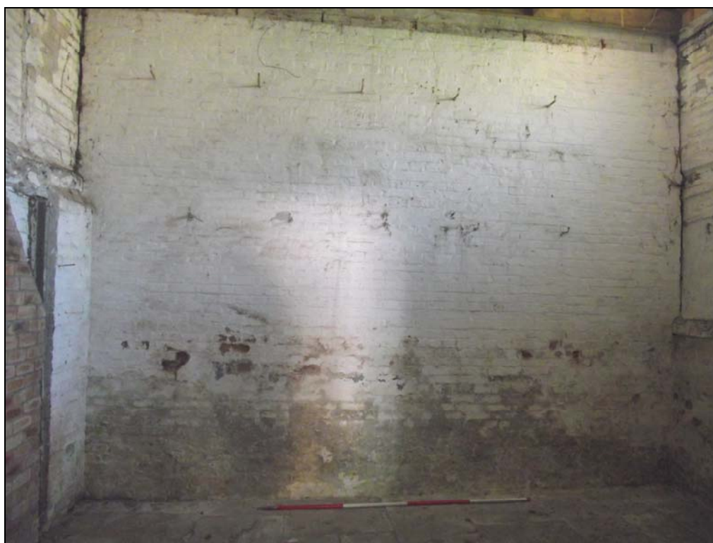
Plate 20, 48: view of the inserted brick south wall with two rows of bracket hooks [8], from the north
