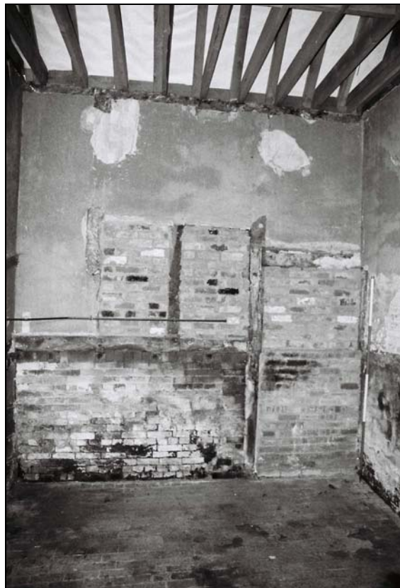
Plate 16, 34: room 3, view of the east wall with blocked doorway [4], from the west
