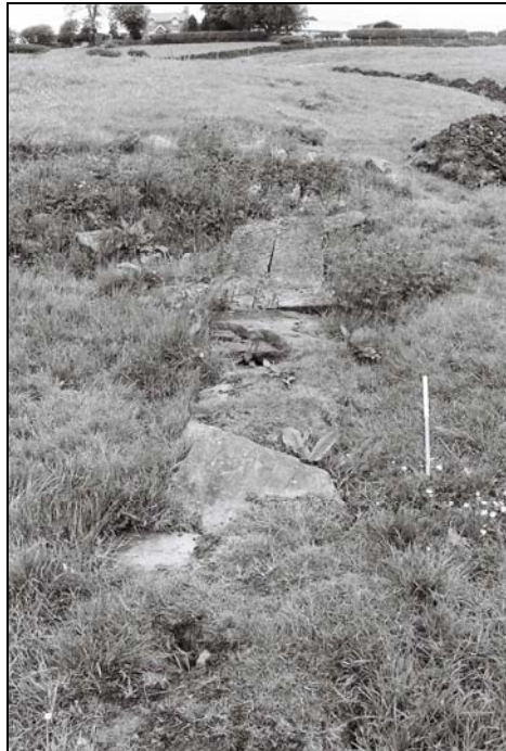
Plate 1, 1: pre-excitation view of the exposed top of the stone culvert, from the east
