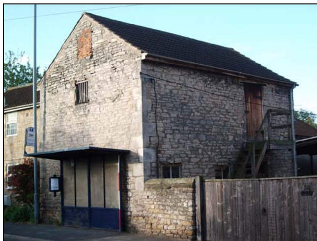
Plate 3, 3: oblique view of the front gable wall of the stable (Blg B), looking southwest
