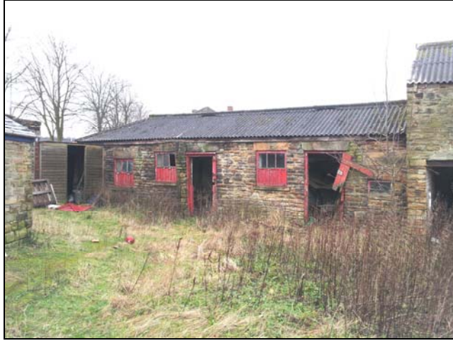
Plate 13: view of the front SE elevation of the Mistal/Stable (Blg. E), looking southwest
