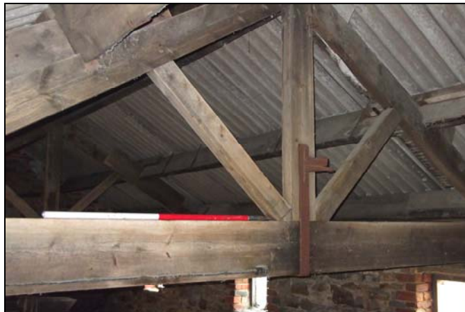
Plate 19: the barn, (Blg. F) view of the king post roof truss, looking southwest
