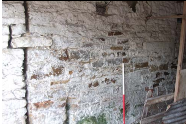
Plate 16: detail of the vertical building line with the barn wall (Blg. F: left) stitched in to the earlier Mistal/Stable wall (Blg. E), looking southwest
