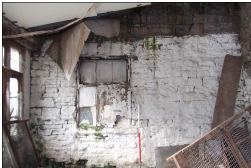
Plate 21: Blg. G, internal view of the glazed window, looking northwest towards the once external southeast elevation, looking northwest
