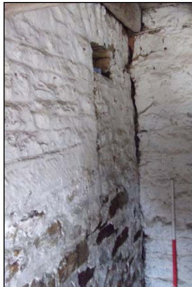
Plate 17: Blg. F, SW wall, view of the blocked arched opening, looking west
