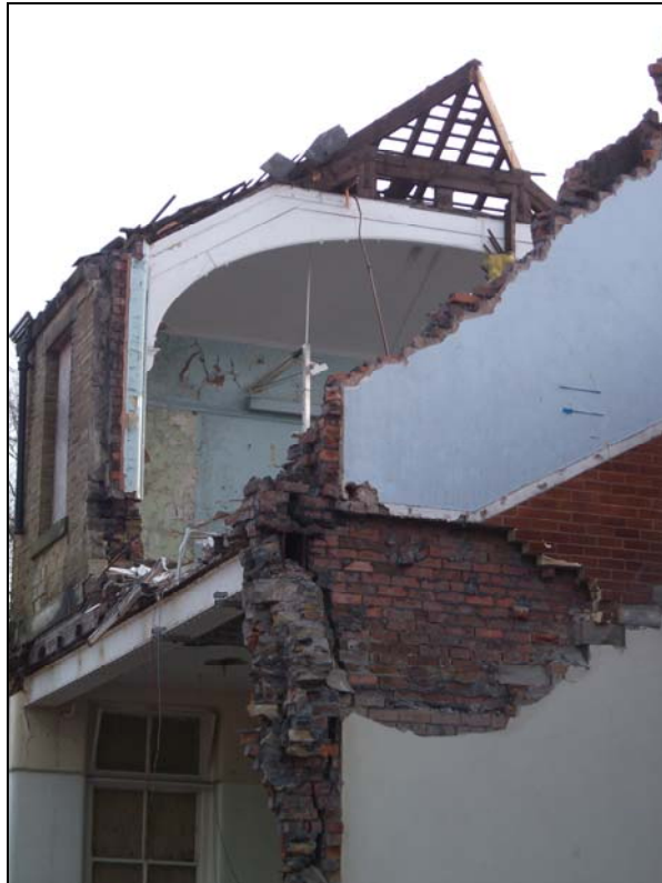
Plate 11, 48: view of a cross sectional view through the building with the type 3 roof truss in situ, from the west
