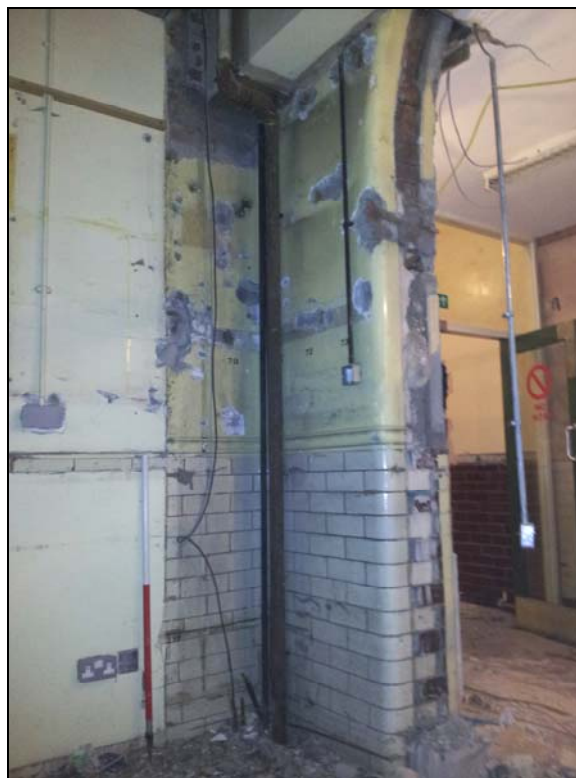
Plate 4, 17: room 16, exposed view of the original walls and archway, from the west
