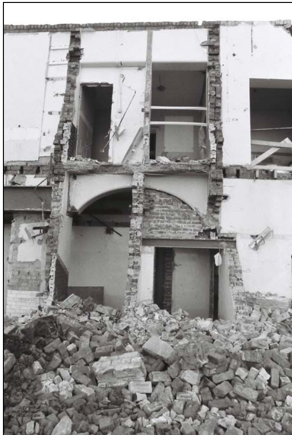
Plate 6, 23: view of the part blocked archway to the SW staircase, from the northwest
