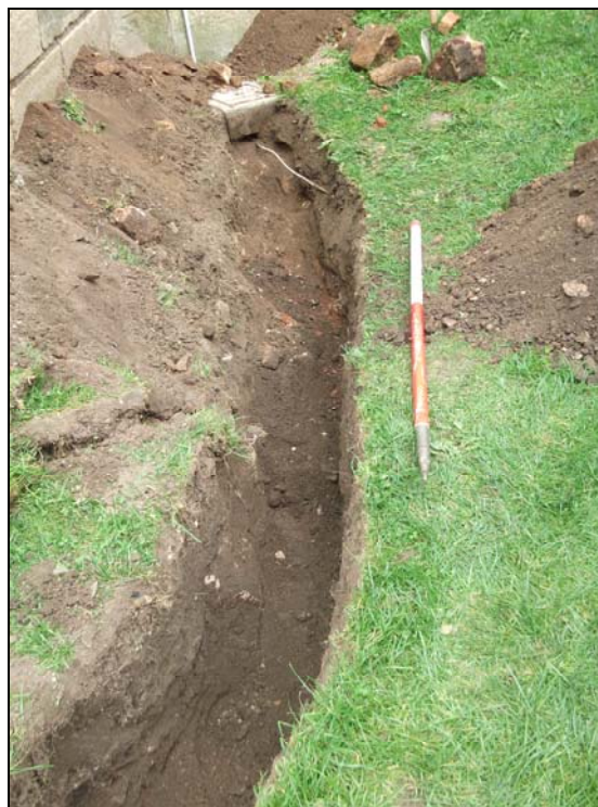
Plate 7, 9: general view of the trench linking to the existing lightning conductor, from the south southeast
