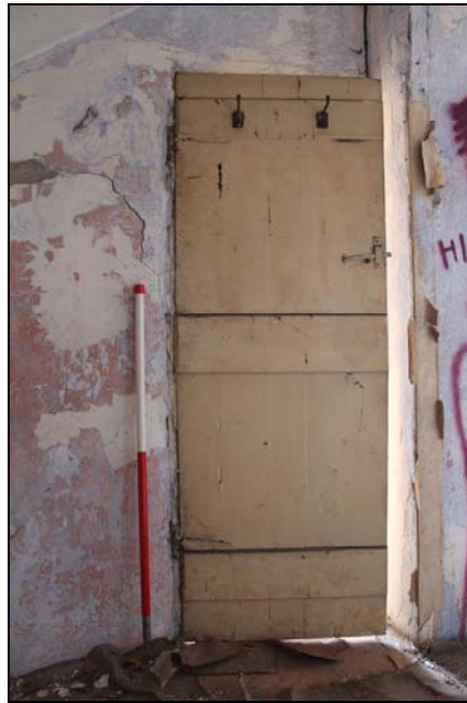
Plate 24, 33: detail of the Bedroom door (the only in situ door into Rm. 7), looking east south east
