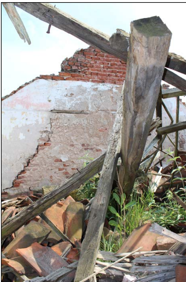
Plate 27, 27: room 9, general view of the collapse roof and SE gable wall, looking southeast
