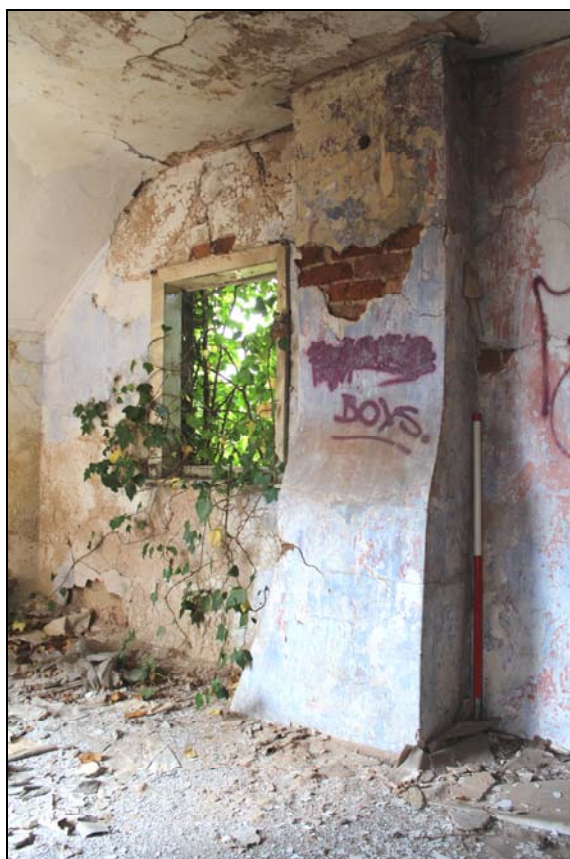
Plate 23, 30: view of the NW wall with single flued chimney breast and sliding sash window, looking northwest
