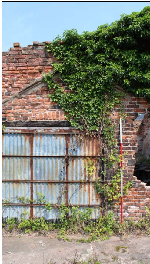
Plate 8, 11: detail of the roof scar [N] and arched doorway [O] above the modern inserted doorway. looking east northeast
