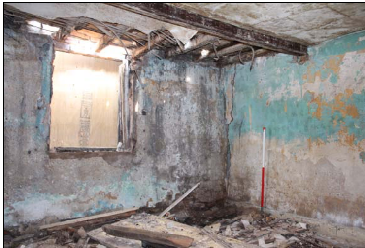
Plate 19, 42: general view of the front NE wall with central window, looking southeast
