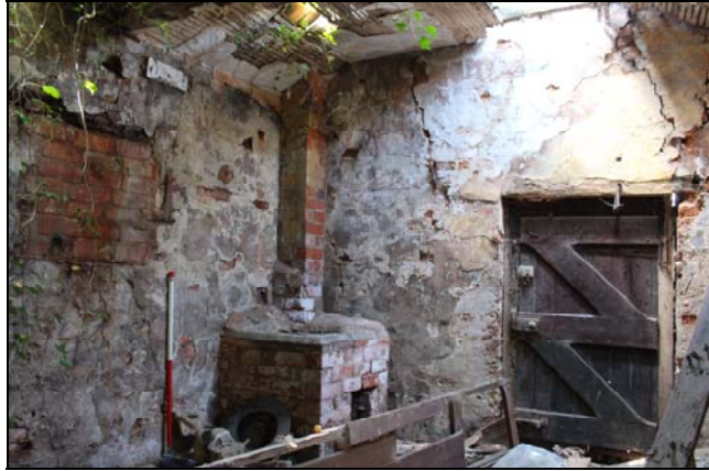
Plate 12, 21: room 1, general view with the inserted boiler and upturned bench top, looking northwest
