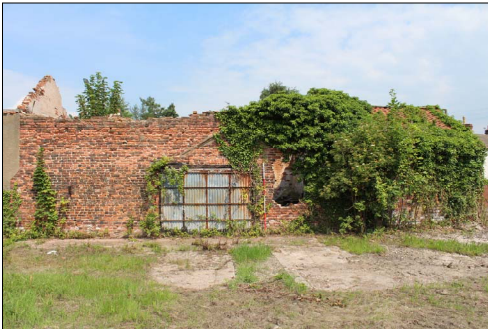
Plate 7, 10: the Barn (Blg. 2), view of the rear SW Elevation of the barn with obscured garage, looking northwest
