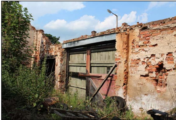
Plate 29, 58: The Barn , room 10, View of the front NE wall with barn door and inserted window [E], looking north
