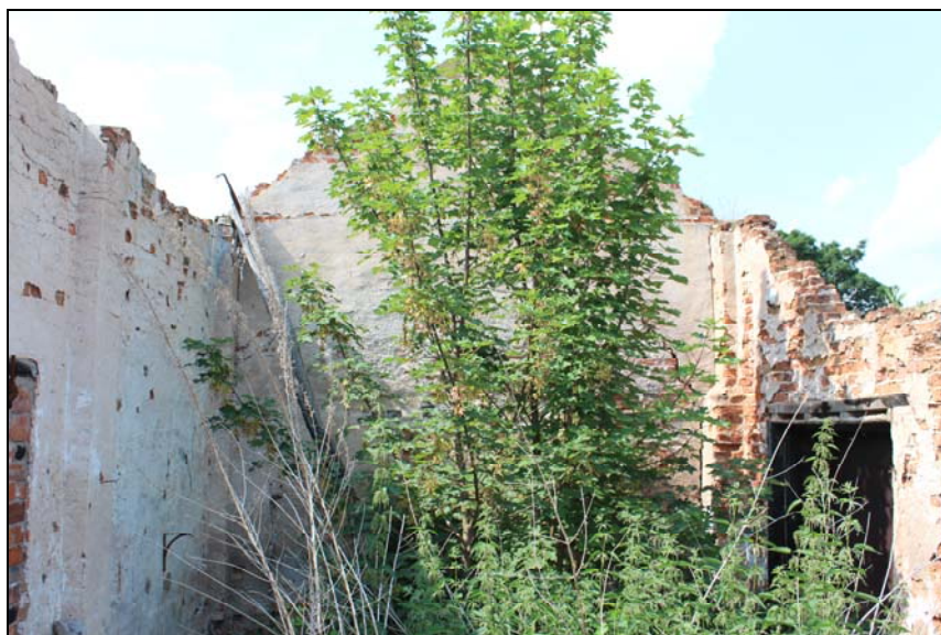
Plate 28, 51: The Barn , room 10, general view of the former barn, looking north northwest
