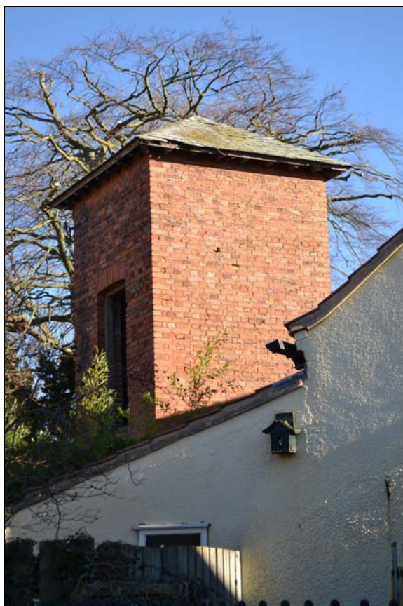
Plate 1, 16: the tower, distant view from in front of the former farmhouse, looking east
