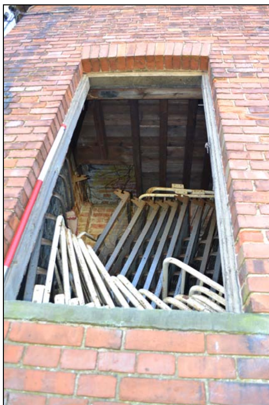
Plate 6, 8: the tower, view of the second floor doorway to the northwest elevation, looking southeast
