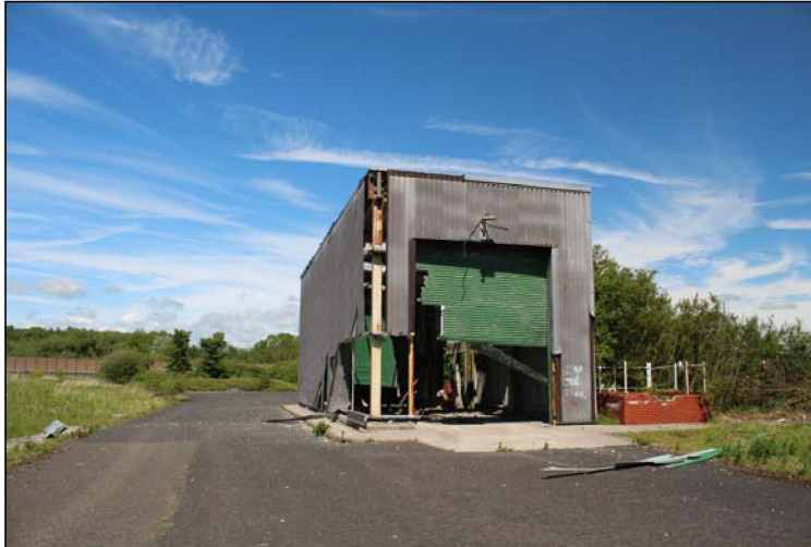
Plate 10, 18: the only building (A) within the PDA, a former truck wash, looking north
