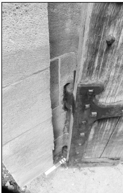
Plate 11, 21-20: view showing how the stone jambs have been inset to take the edges of the gates [5d, 5e] (0.2m scale)
