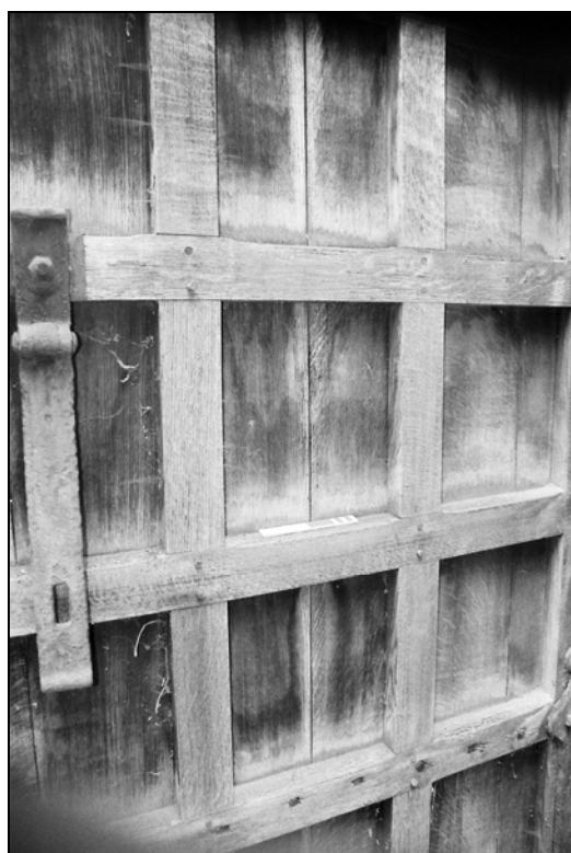
Plate 9, 26: slight oblique view of the construction and detailing of the rear framework, looking north-west [5a]
