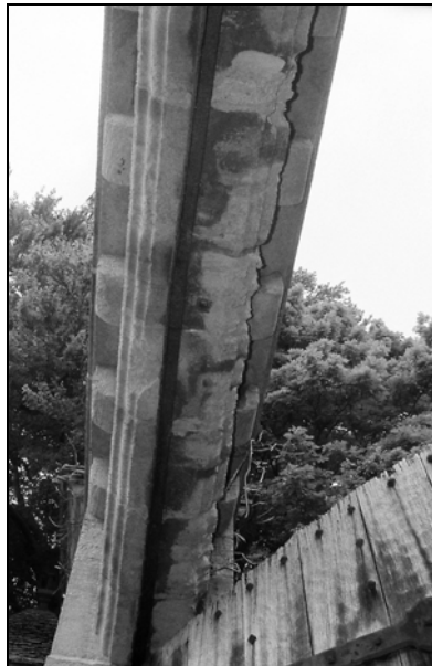
Plate 17, 14: view of the brattished iron detail within the stone arch above the gates [2]
