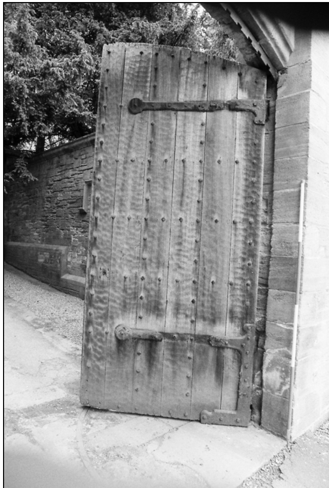
Plate 5, 30: detail of the gate door adzed surface of the oak cladding boards, looking east [4]
