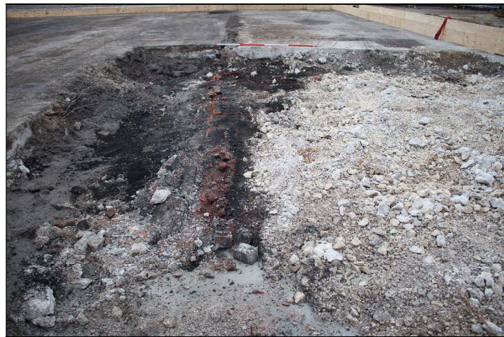
Plate 2: view of the proposed excavations, with in situ wall, from the east
