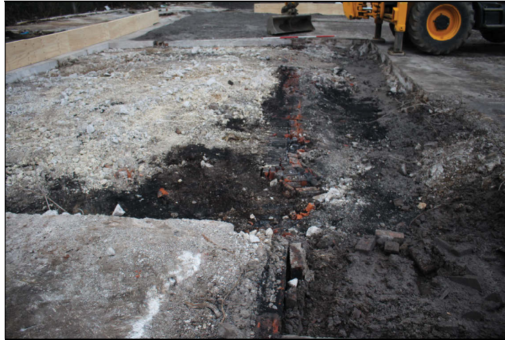
Plate 1: view of the proposed excavations, with in situ wall from the east
