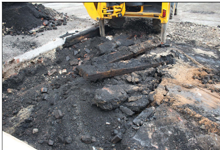
Plate 6: during removal of the brick sett floor machine base timbers were revealed these formed a series of parallel bases down the PDA, from the northwest
