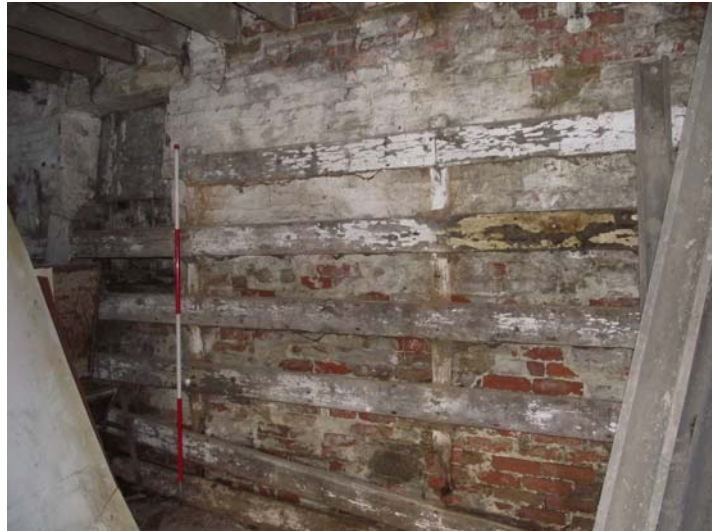
Plate 18, 227: View of the wall mounted racks to the north wall, from the southeast
