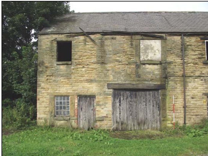
Plate 7, 83: General view of the Store Building (bays 1&2), Southeast Elevation, from the south
