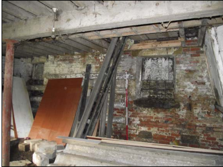
Plate 17, 88: General view of the obscured north wall with timber racking, from the south southeast
