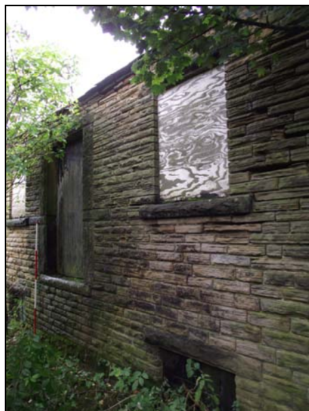
Plate 12, 79: Oblique view of the North Elevation with loading door, from the west northwest
