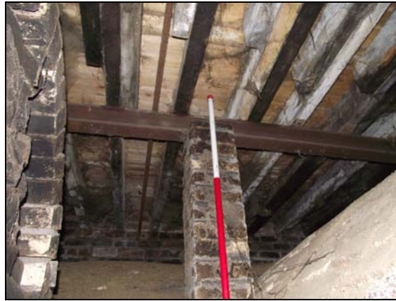
Plate 23, 223: View above the oven with brick pillar supporting the inserted 'I' beam, from the south southeast
