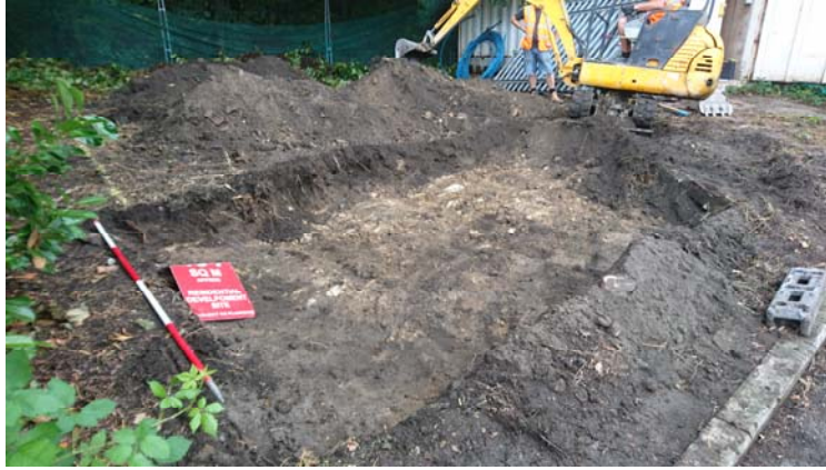
Plate 4: post excavation view of the southern half of the site, looking northeast
