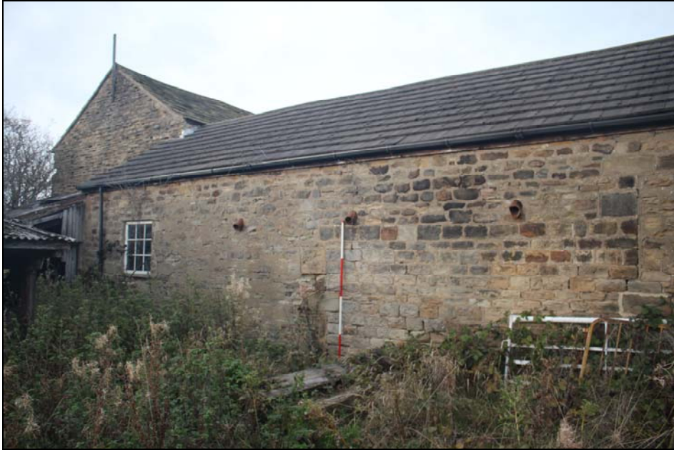
Plate 36, 30: Oblique view of the rear wall of the later Cow House, west end with older in situ walling, from the east southeast
