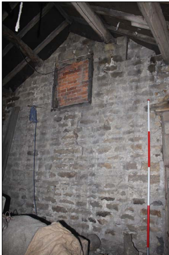
Plate 28, 76: D.3, Full height view of the north wall (former external barn wall), from the east
