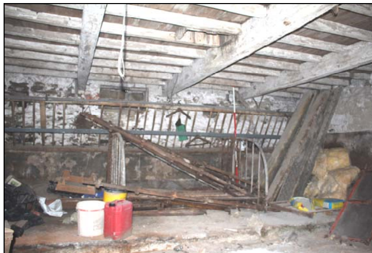
Plate 25, 96: D.2, view of the hayrack, stalls to the west wall, from the east
