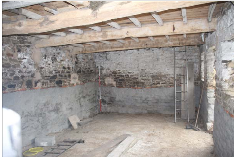
Plate 4,5: Rm B.1, General view of the ground floor, from the west south west
