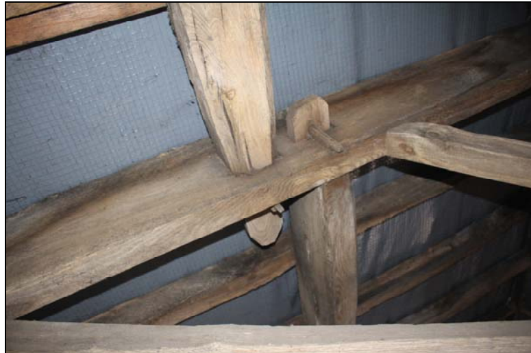
Plate 8, 14: Rm.B.2 detail of the tenoned and pegged purlins and the principle rafter of the king-post roof truss, from the NNE
