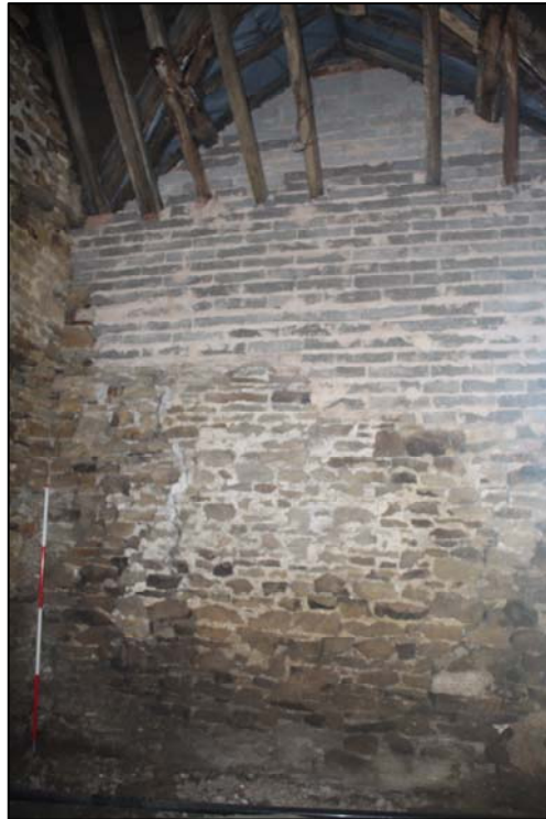
Plate 15, 40A: C.1, View of the Barn's east wall (full height), from the west southwest
