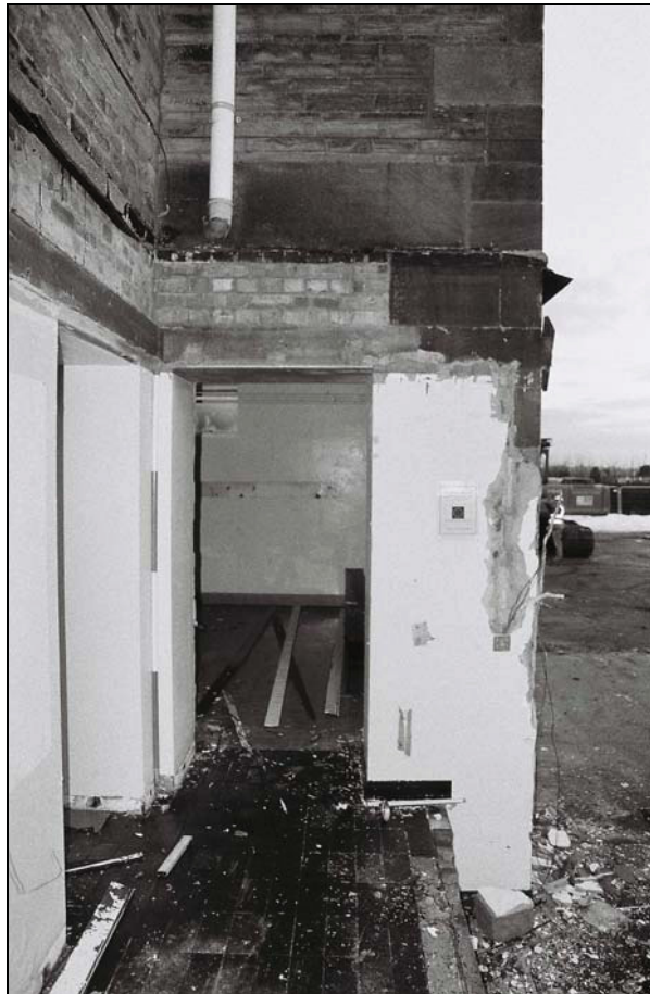
Plate 2: Building 3, detail of an original doorway [1] denoted by ashlar lintel and associated quoins, from the south
