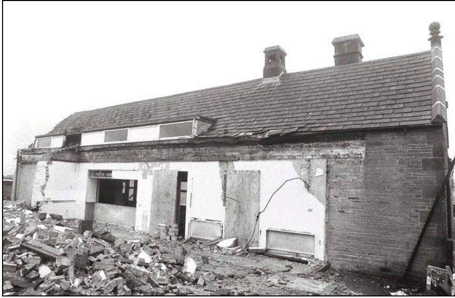
Plate 13: The heavily modified North Elevation with the former kitchen and chimney removed, from the northwest
