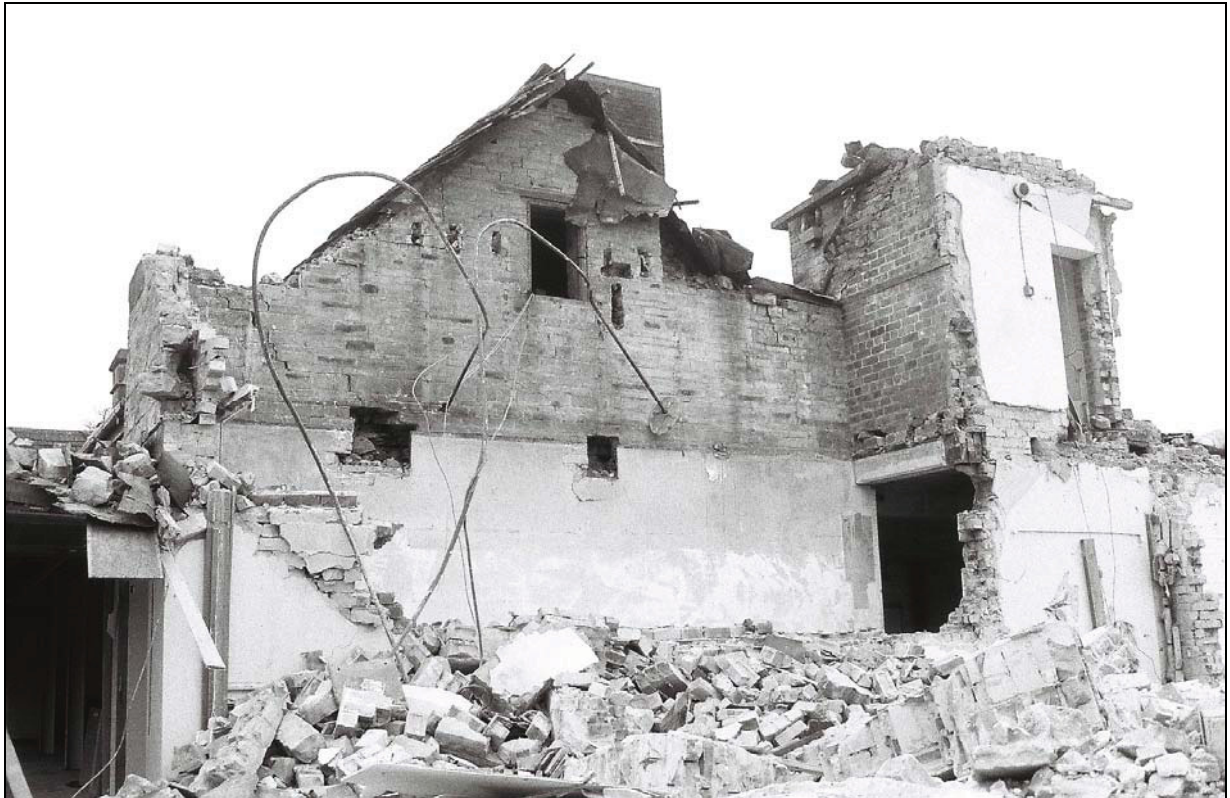
Plate 11: General view of Building 2's eastern gable wall with in situ window (and inserted tie bars [6]), from the south-east
