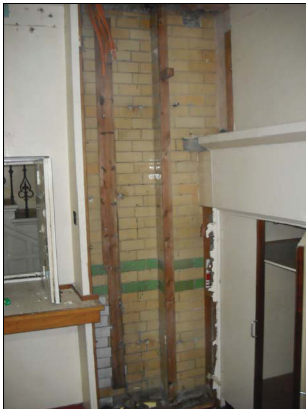
Plate 22: Detail of the original Victorian tiling in the former and original 'Kitchen' (Room 0/3), from the west
