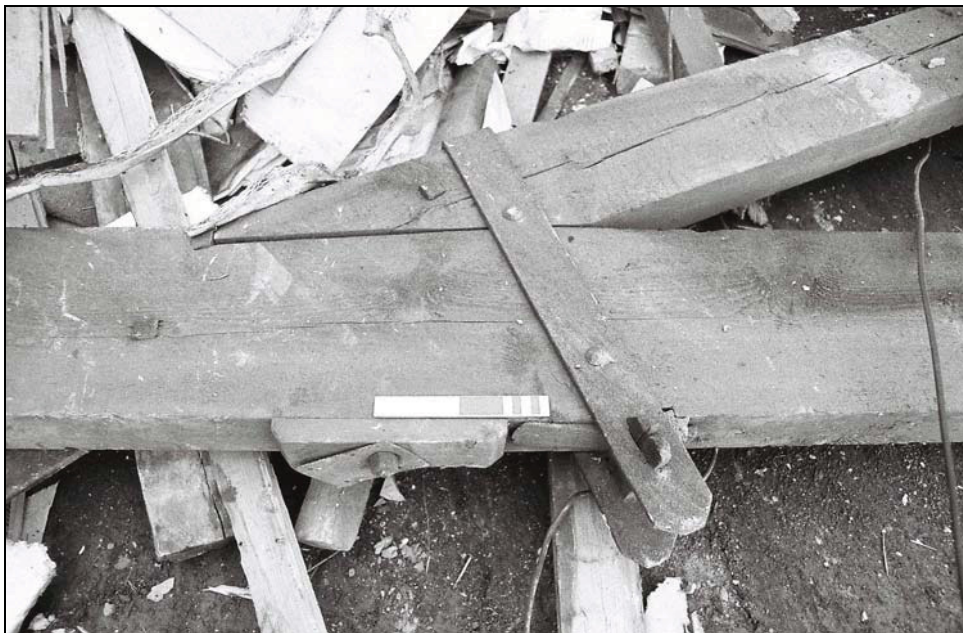
Plate 10: Detail of the roof truss [5] at the junction of the brace and principal rafter with its strengthened joint
