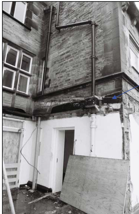
Plate 26: View of the rear entranceway with inclined roof scar and blocked window above, from the northeast
