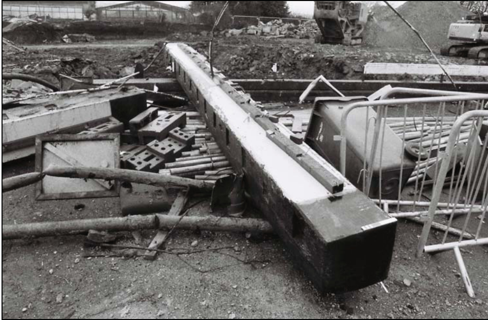
Plate 19: View of the removed lintel with joist rebates of building 2's 'cartdoor', from the south
