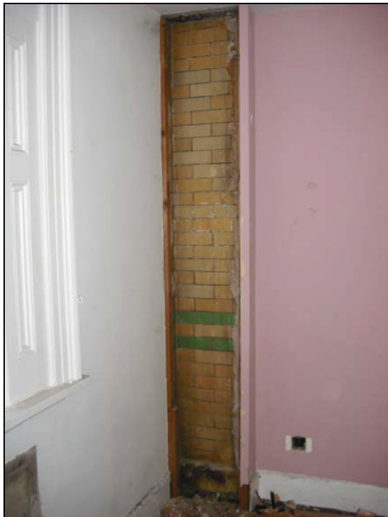
Plate 24: View of the underlying tiling (cream with green bands) of the former 'Servants Hall', from the north northwest
