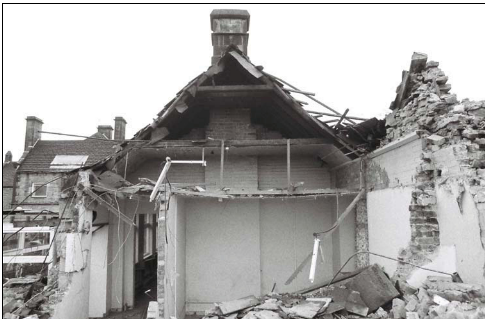
Plate 16: Detailed view of a cross section through Building 2 (southern range), from the north
