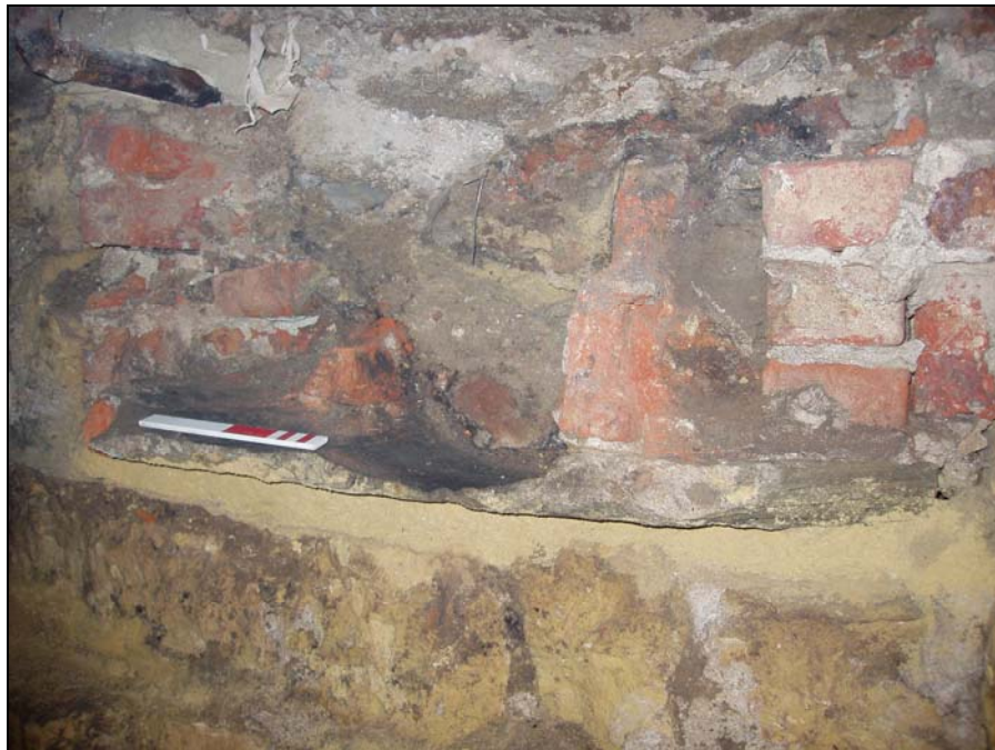
Plate 6, 38: trench 1b, Doorway A with a detailed (oblique) view (0.2m scale) of the brick duct [108] with partially collapsed baffle and soot stained moulded flagstone, from the northwest
