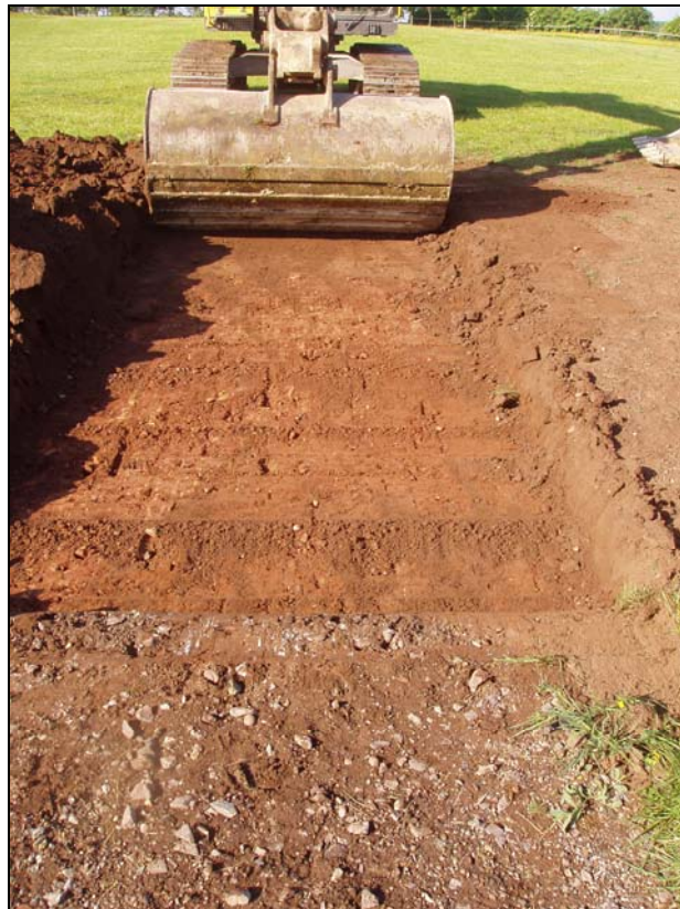
Plate 2: working shot of the initial excavations revealing a linear feature [004] (with alignment highlighted), from the northeast
