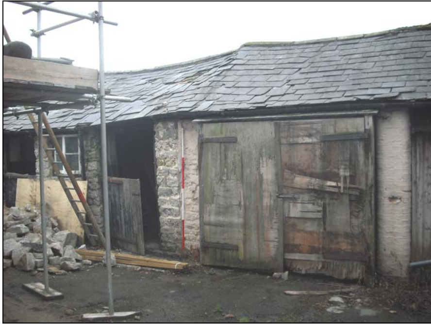
Plate 17, 8: general view of the southern end of the Northeast Elevation , from the north
