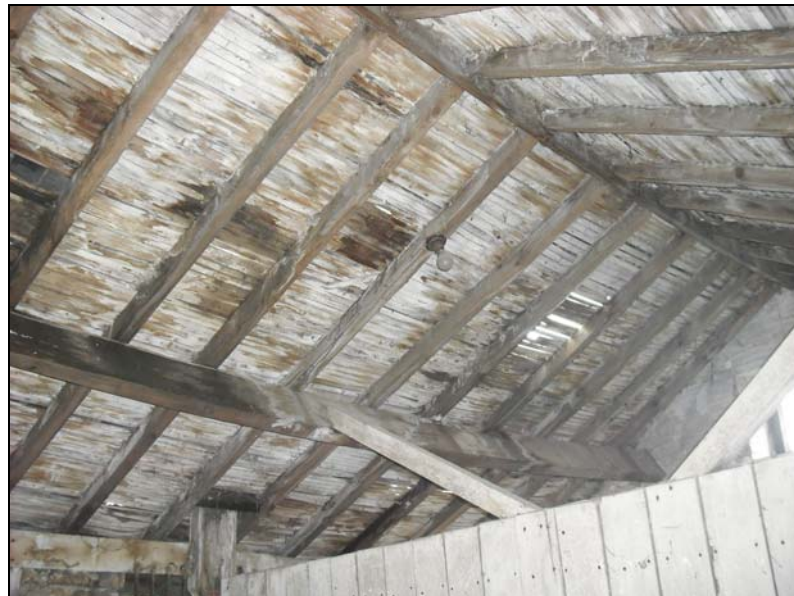
Plate 22, 45: building B, room 6, view of the roof underdrawn with laths (no evidence for a plastered underdrawn finish), from the southeast
