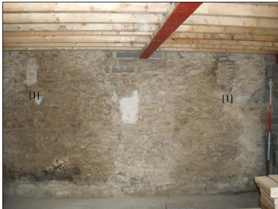
Plate 8, 23: view of the southeast wall (northwest end) with 2 blocked slit ventilators [1] and blocked window [3] below the inserted 'I' beam, from the northwest
