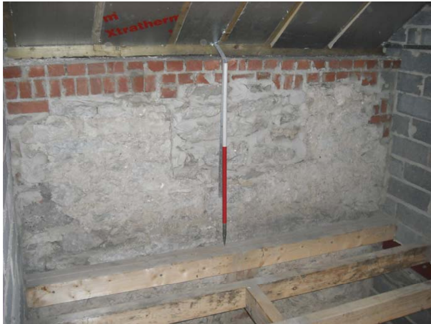
Plate 15, 32: view of the southeast wall with first floor blocked window [3], from the northwest
