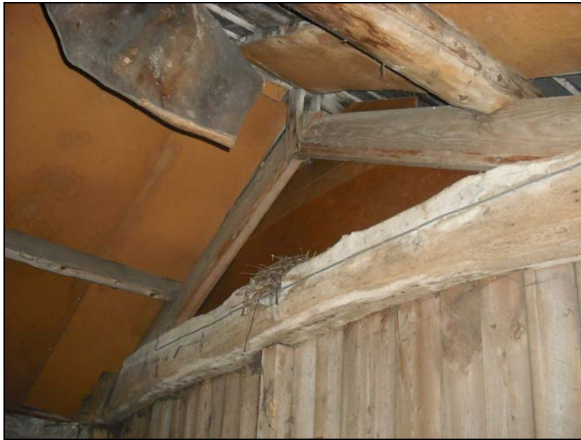
Plate 23, 49: building B, room 7, view of the re-used oak collar from a roof truss, from the east
