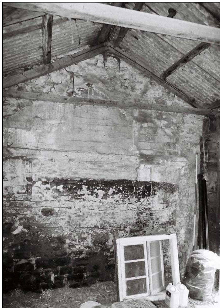
Plate 29, 64: Building C, view of the earlier northeast wall which Building C abuts, from the southwest
