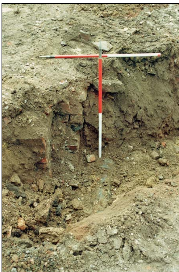
Plate 4: View of the brick wall that was associated with the main cast iron pipe that was aligned SW to NE across the PDA, from the northeast
