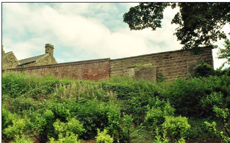
Plate 8: General view of the extant buttressed wall (taken from the bottom of the castle's moat, from the west
