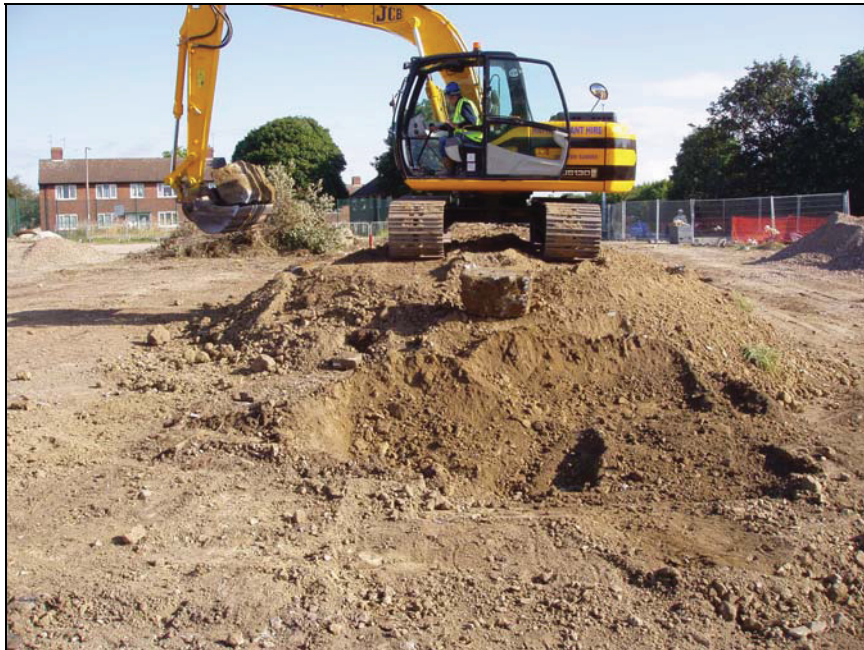
Plate 4: working view of the excavation and removal of the bund, looking north
