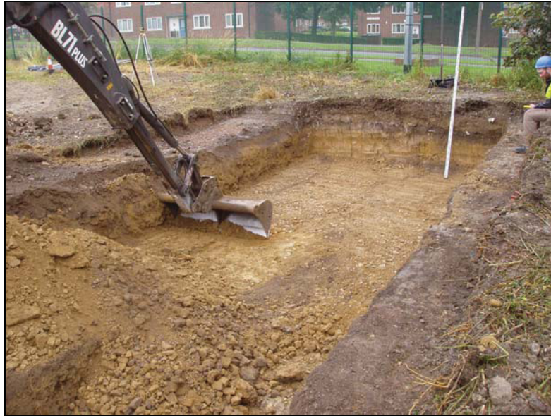
Plate 1: general view during the removal of the upper natural substrate at the electric substation, looking northwest
