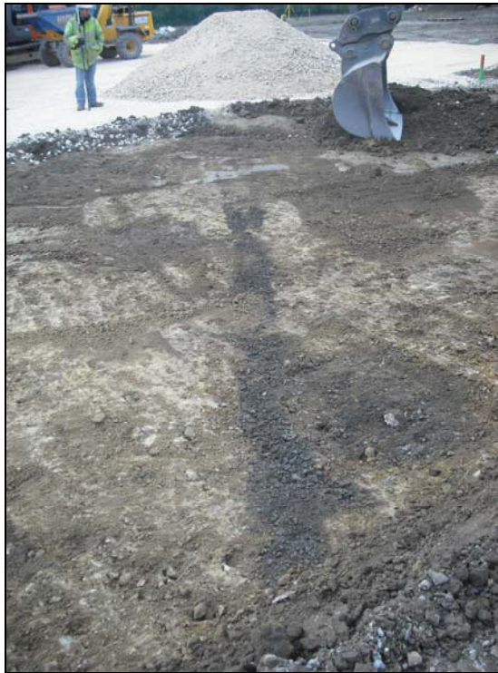
Plate 6: view of the upper terrace with modern land drains and adjacent foundation pads (now removed and backfilled), looking southwest
