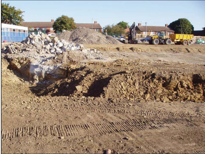
Plate 9: general view of the start of the basement excavations to the SPDA, looking north
